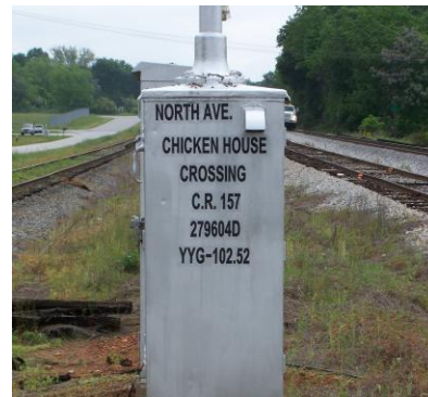
USDOT ID (279604D) on signal equipment enclosure
