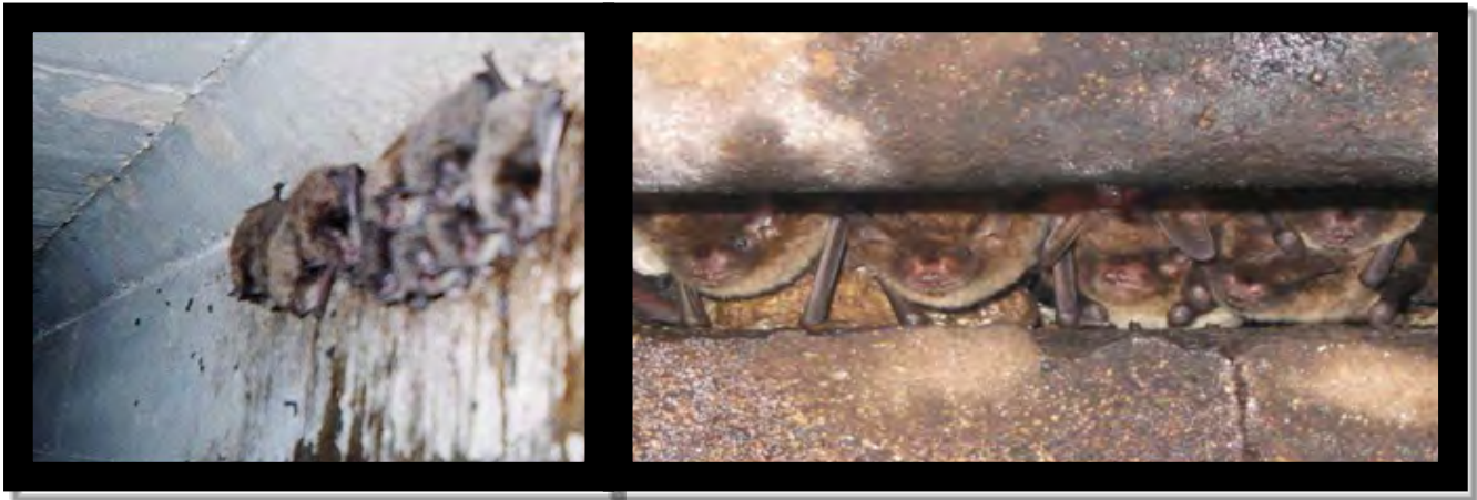
Image 5. Bats roosting in bridges using cracks in support beams & bridge joints Source: https://www.environment.fhwa.dot.gov/esawebtool/Site/ibatNLEBBA.aspx#fiveseven
