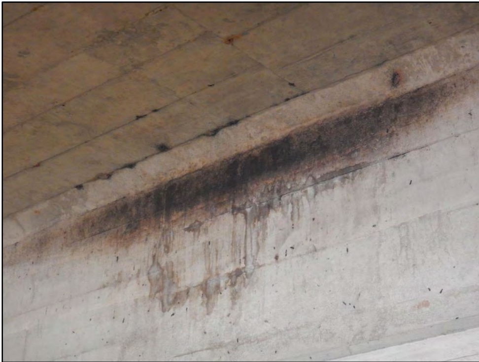
Image 6. Urine staining and guano on support beam Photo By: Anne Sexton, GDOT, Ecologist
