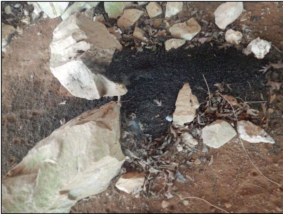
Image 7. Guano pile below bridge deck Photo By: Anne Sexton, GDOT, Ecologist
