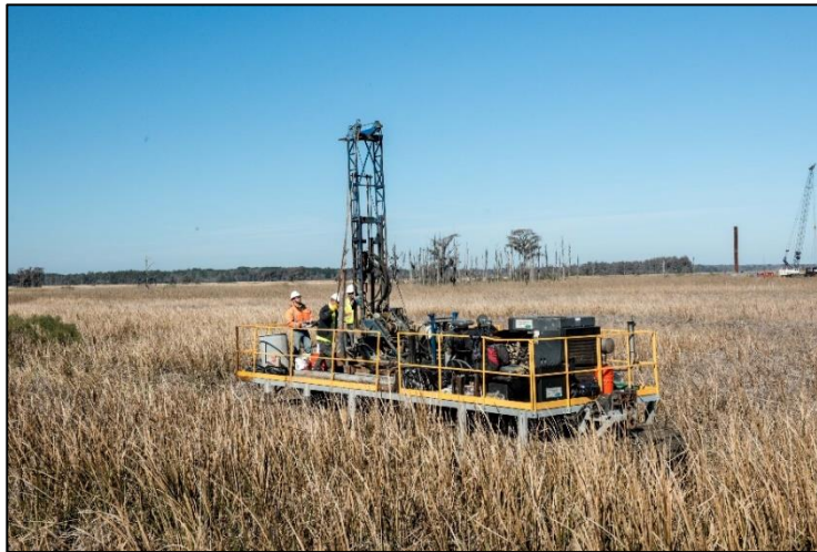
Photo 1. Amphibious rig in a marshland during a GDOT project drilling event. Source: Terracon
