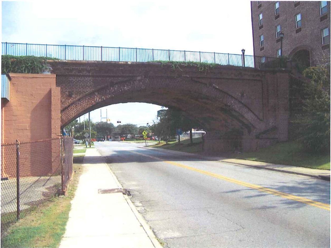
Chatham County, GDOT Bridge 051-0152-0, Central of Georgia RR (abandoned) , over West Boundary Street, 1860
