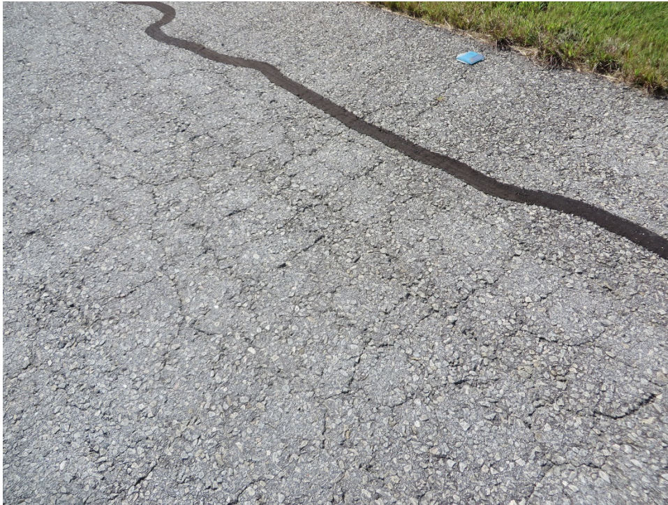
THANGWI-10. Alligator Cracking (Sample Unit No. 02).
