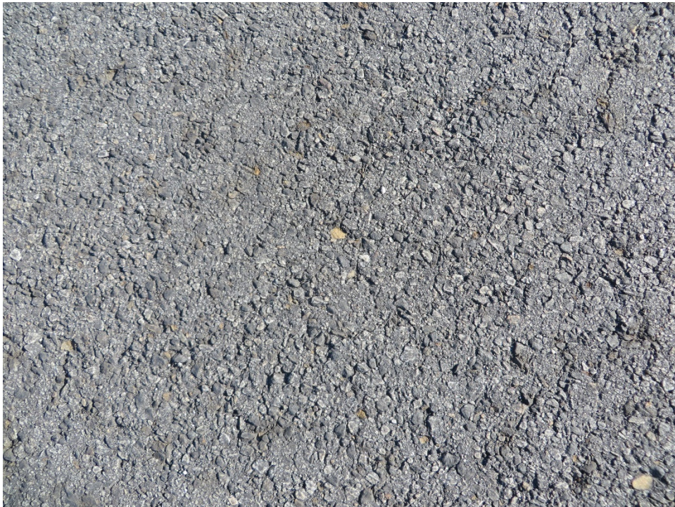
TBWI-20. Weathering (Sample Unit No. 03).
