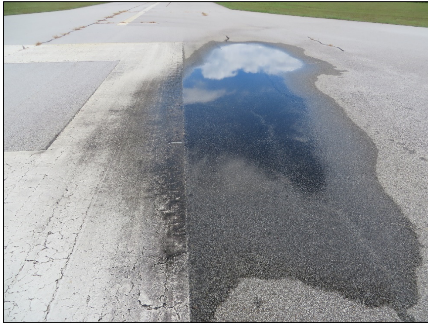
FIGURE H-3 HIGH-SEVERITY DEPRESSION
