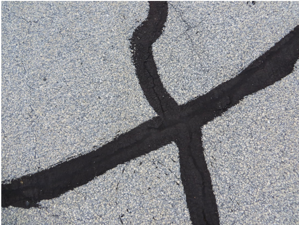
TDWI-30. L&T Cracking (Sample Unit No. 01).
