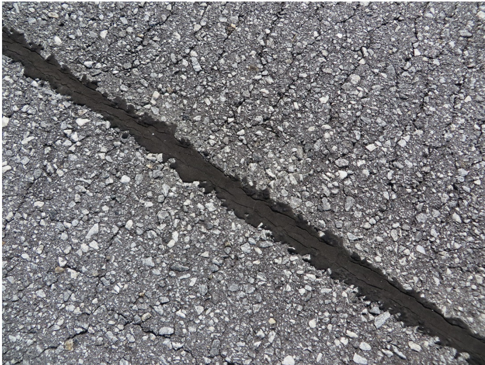
TDWI-10. L&T Cracking (Sample Unit No. 22).
