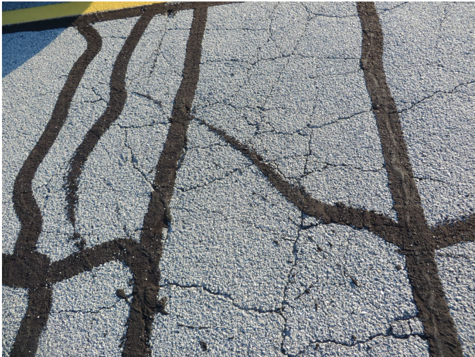
A01WI-10. Alligator Cracking (Sample Unit No. 30).
