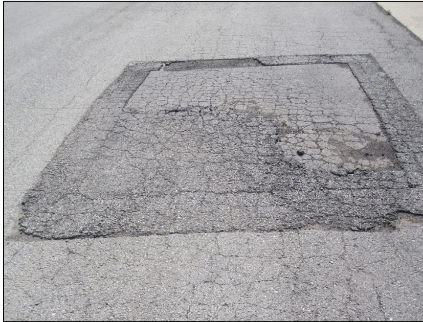
FIGURE H-5 HIGH-SEVERITY PATCHING
