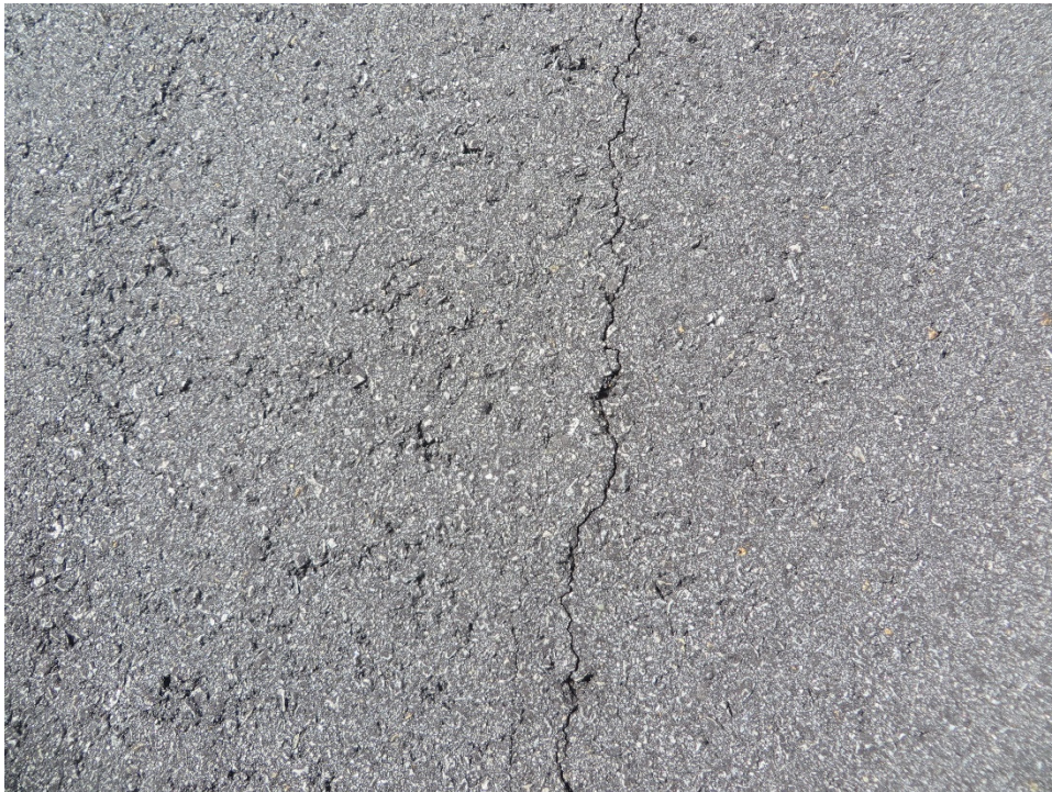
R1331WI-10. L&T Cracking (Sample Unit No. 13).
