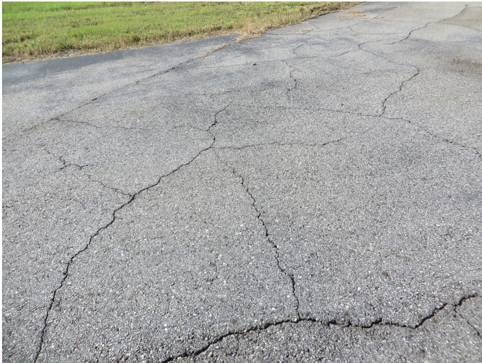
A02WI-20. Block Cracking (Sample Unit No. 05).
