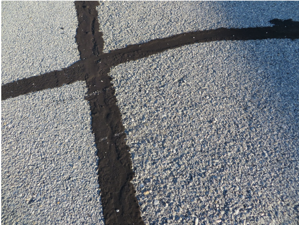
A01WI-10. L&T Cracking (Sample Unit No. 16).
