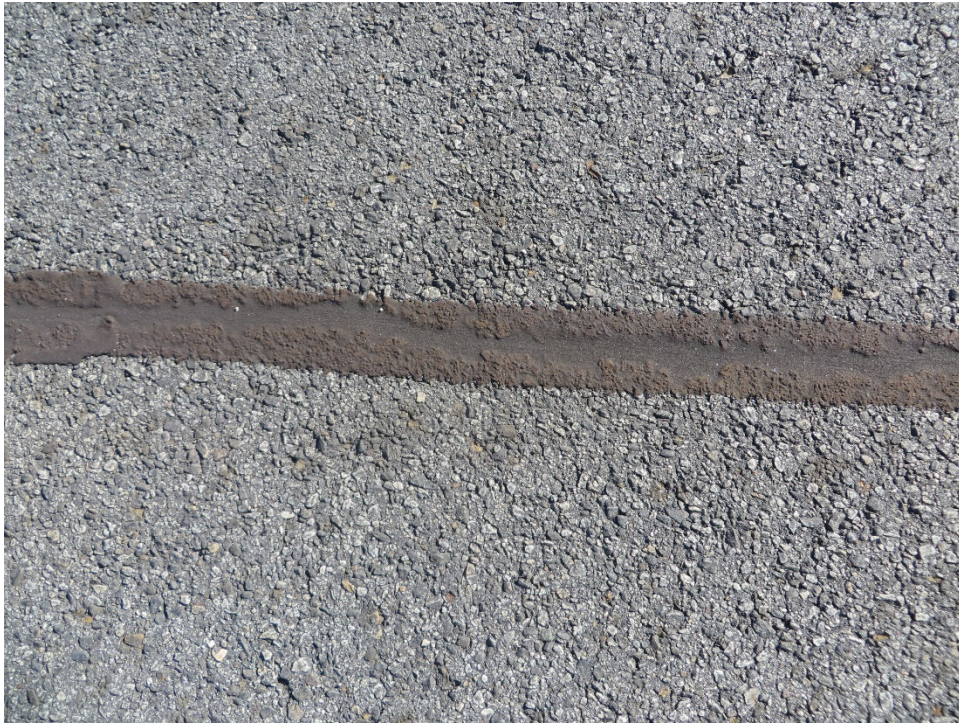
TBWI-20. L&T Cracking (Sample Unit No. 03).
