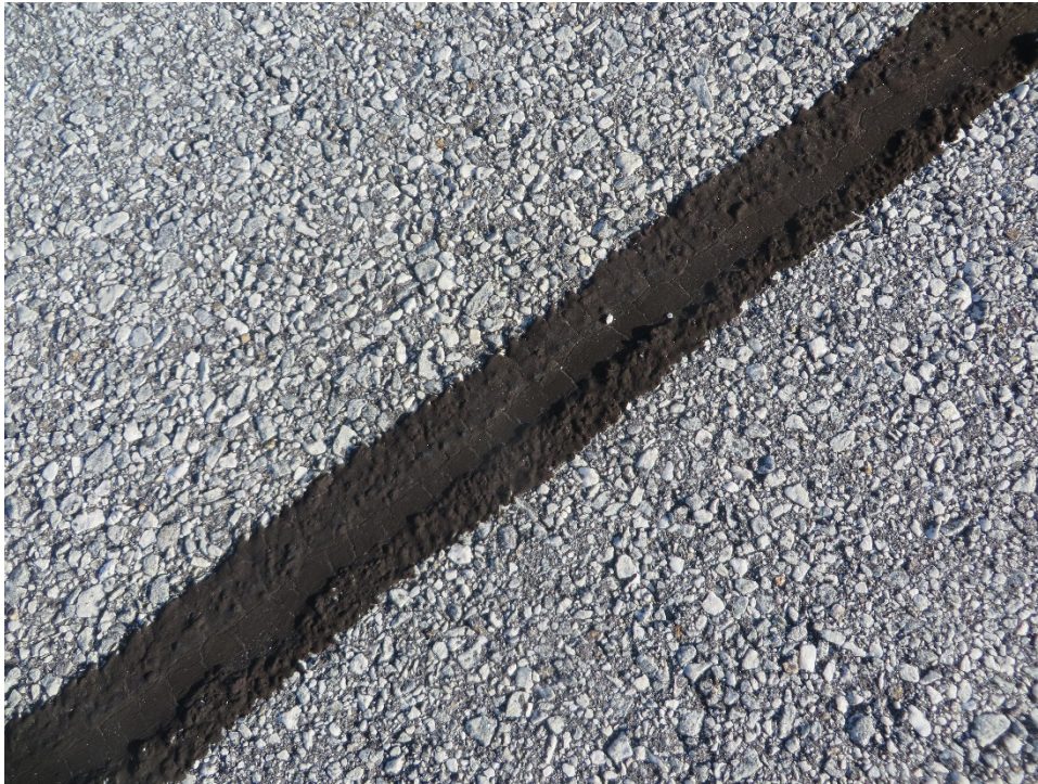
R523WI-10. L&T Cracking (Sample Unit No. 04).
