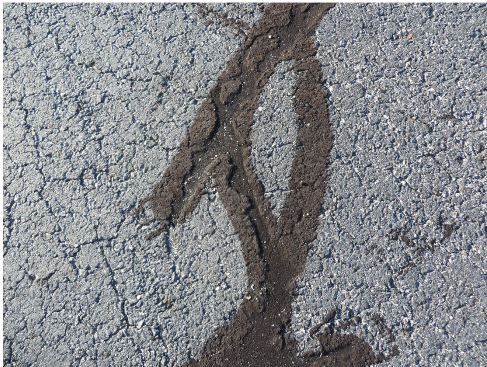
A01WI-20. L&T Cracking (Sample Unit No. 02).
