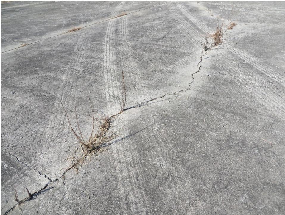
A02WI-30. LTD Cracking (Sample Unit No. 06).
