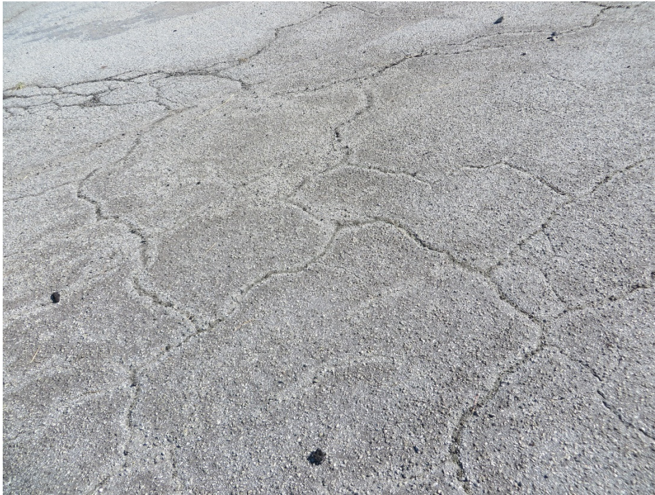
A02WI-10. Block Cracking (Sample Unit No. 03).
