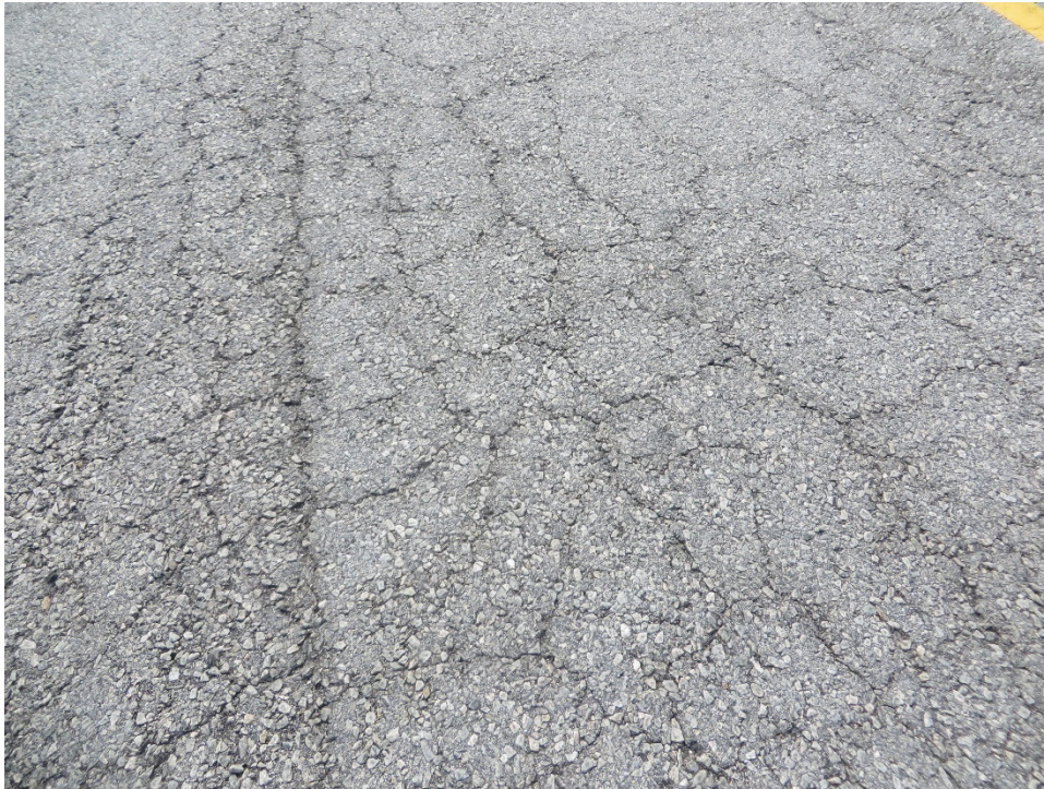
TDWI-20. Alligator Cracking (Sample Unit No. 01).
