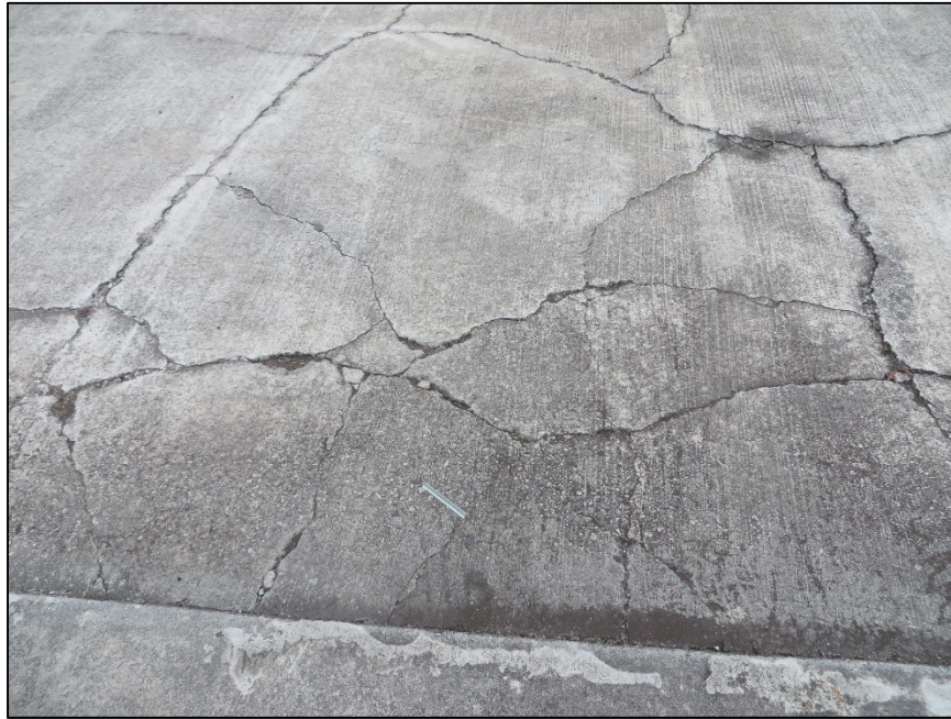
FIGURE H-17 HIGH-SEVERITY SHATTERED SLAB
