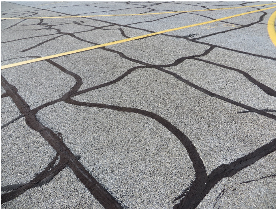
TBWI-10. Block Cracking (Sample Unit No. 43).
