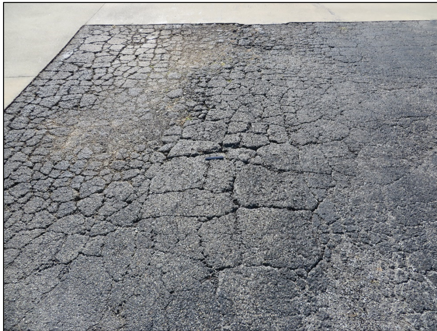
FIGURE H-1 HIGH-SEVERITY ALLIGATOR CRACKING
