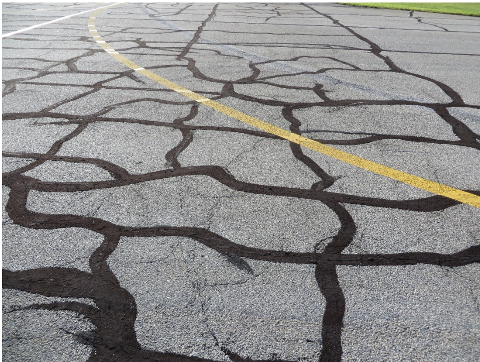
R523WI-20. Block Cracking (Sample Unit No. 02).
