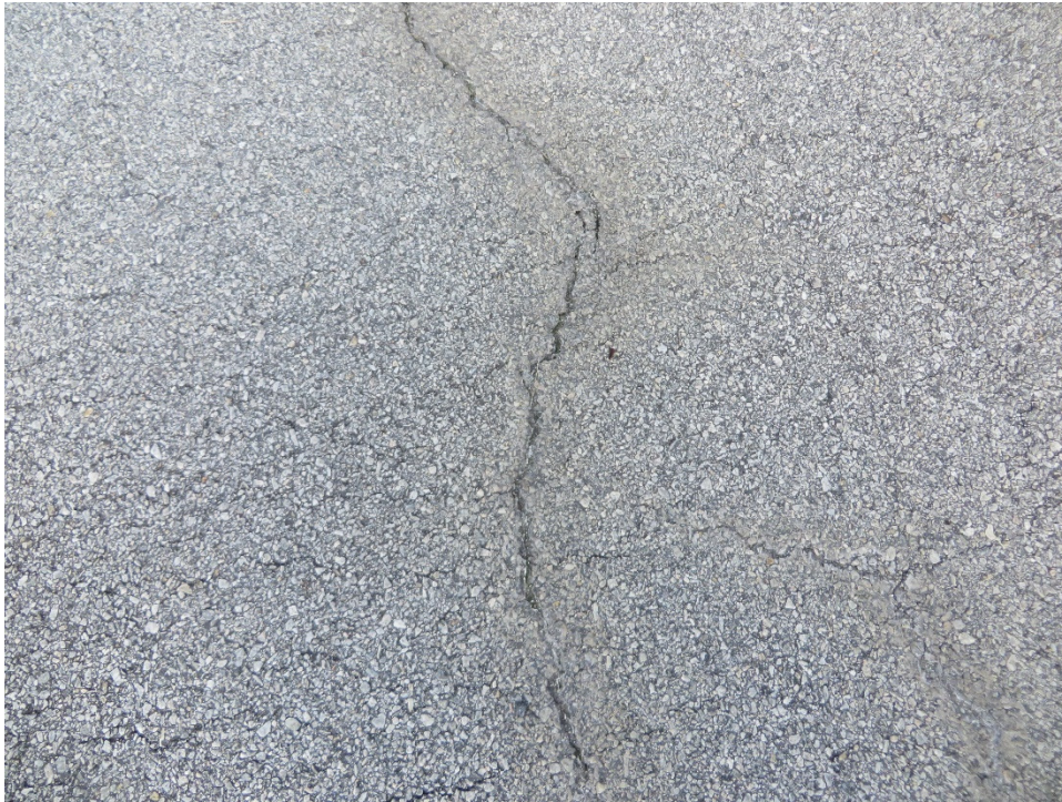
THANGWI-30. L&T Cracking (Sample Unit No. 02).
