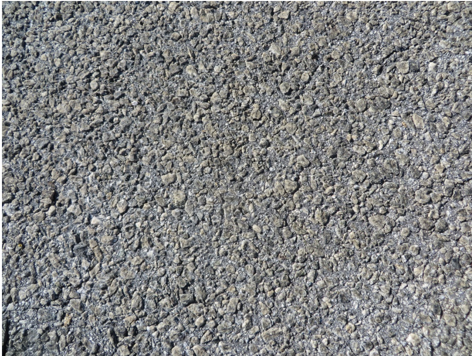
TBWI-10. Weathering (Sample Unit No. 43).
