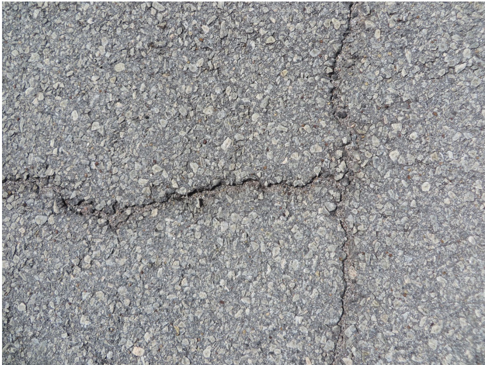
THANGWI-20. L&T Cracking (Sample Unit No. 17).
