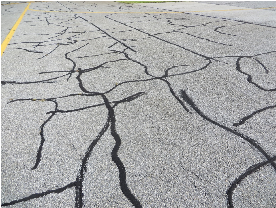
TAWI-10. Block Cracking (Sample Unit No. 25).
