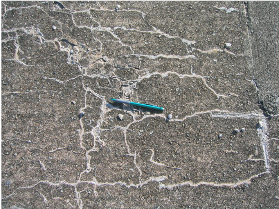
R1331VD-10. Durability cracking.
