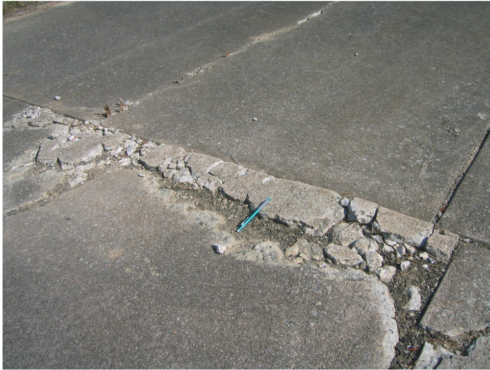
R1331VD-10. Joint spall.
