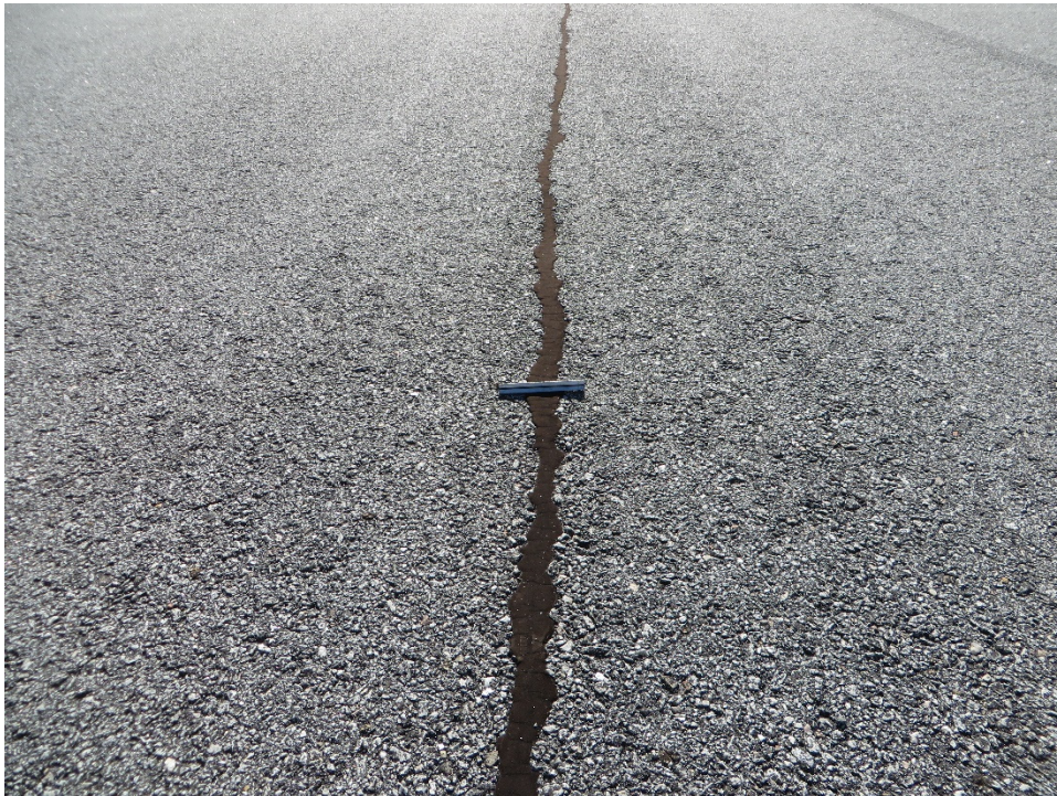
R1735ML-10. L&T Cracking (Sample Unit No. 10).
