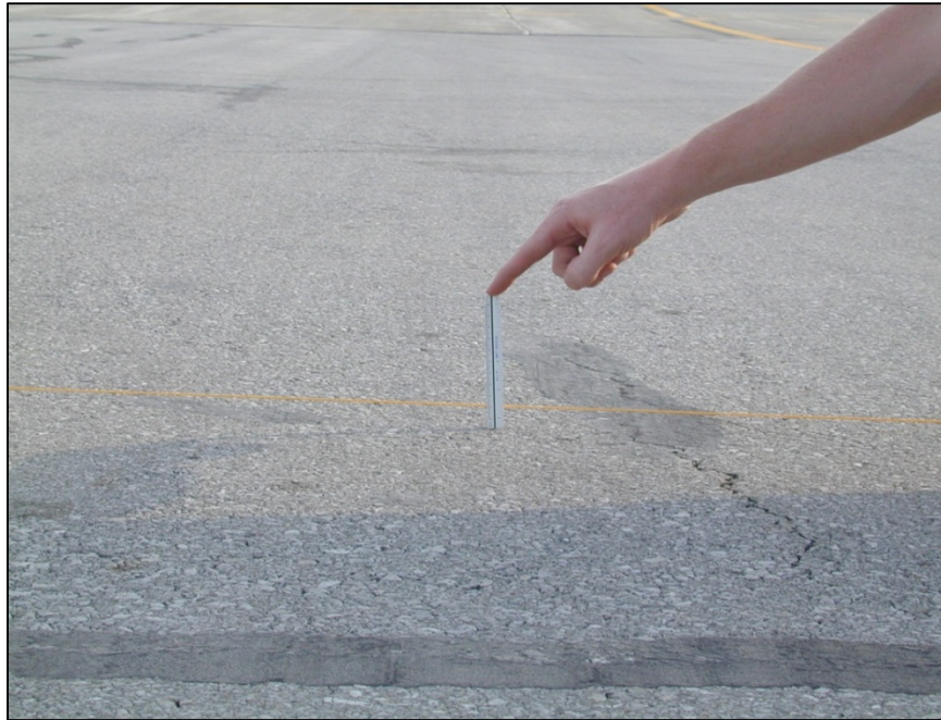
FIGURE H-7 HIGH-SEVERITY RUTTING
