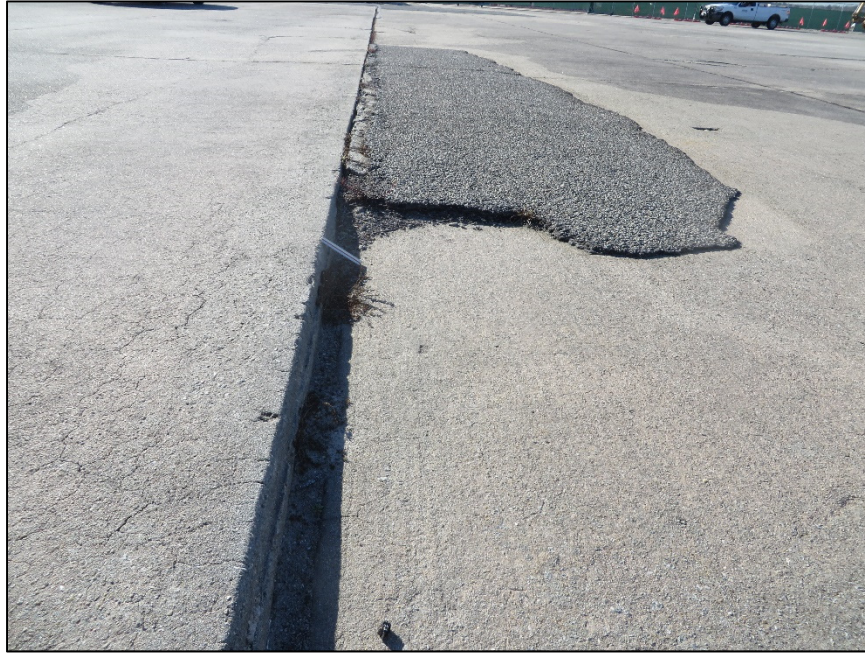
FIGURE H-16 HIGH-SEVERITY FAULTING/SETTLEMENT
