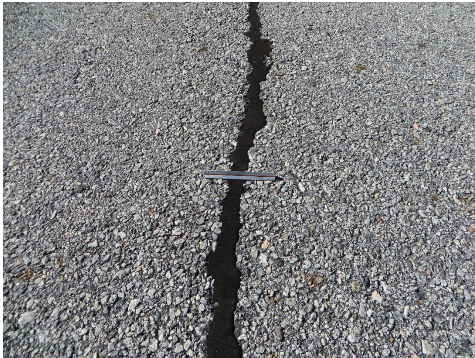
THANGML-10. L&T Cracking (Sample Unit No. 05).
