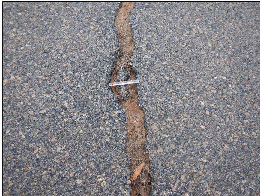
FIGURE H-4 HIGH-SEVERITY CRACKING
