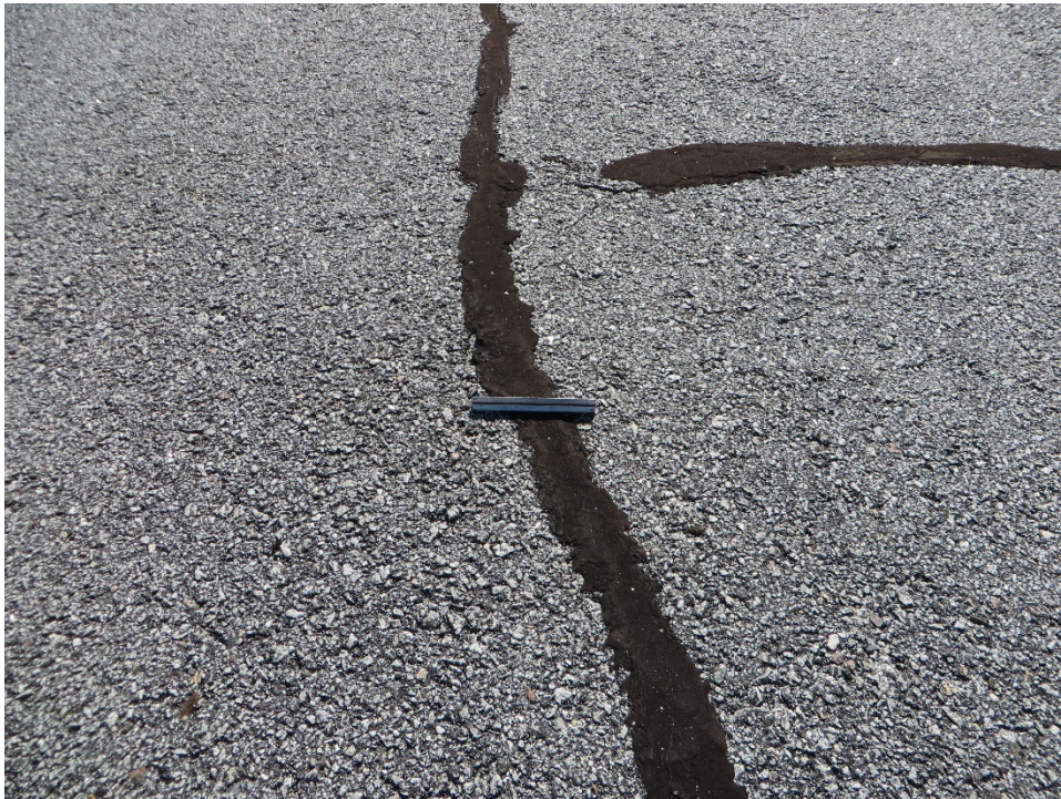
A01ML-10. L&T Cracking (Sample Unit No. 05).
