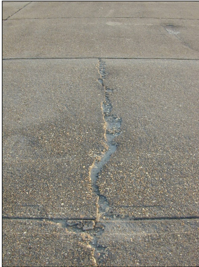
FIGURE H-12 HIGH-SEVERITY LTD CRACKING
