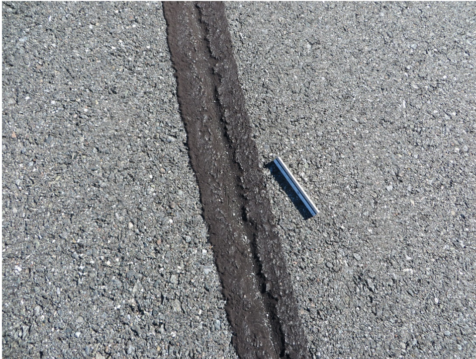
R1432HO-20. L&T Cracking (Sample Unit No. 12).
