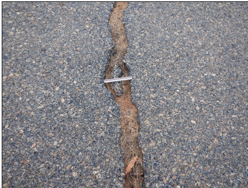
FIGURE H-4 HIGH-SEVERITY CRACKING
