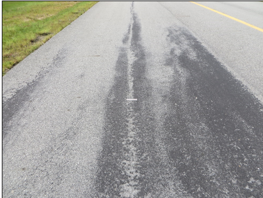
FIGURE H-2 EXTENSIVE BLEEDING
