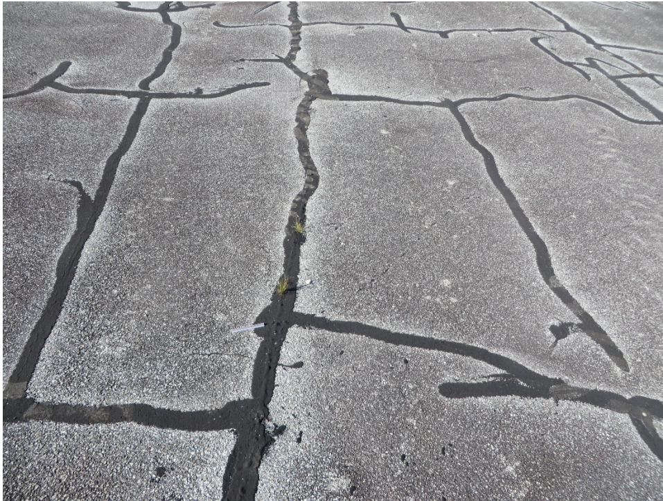
R1432HO-10. Block Cracking (Sample Unit No. 48).
