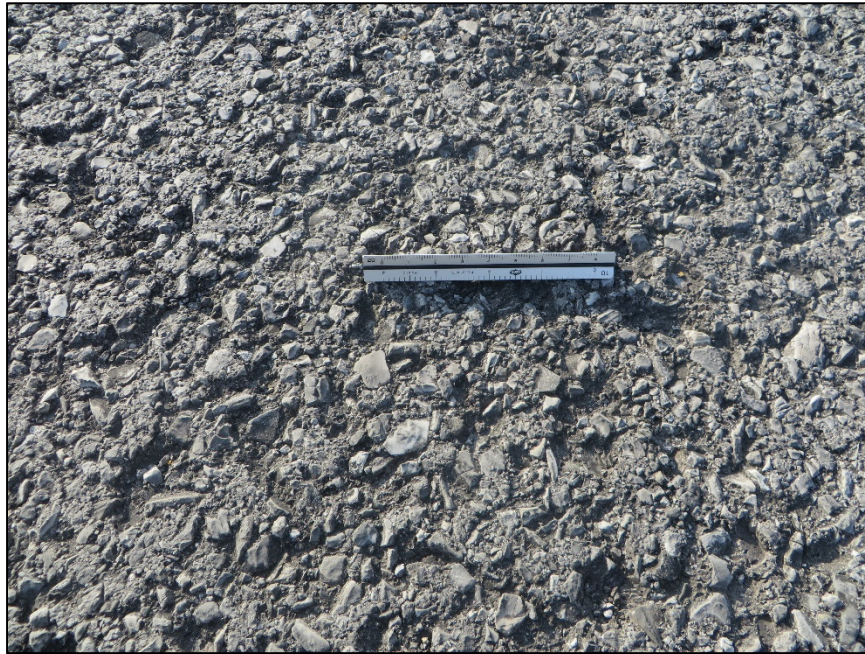
FIGURE H-6 HIGH-SEVERITY RAVELING
