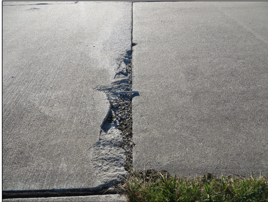
FIGURE H-18 HIGH-SEVERITY JOINT SPALLING
