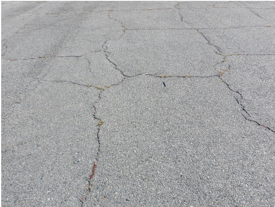
A01HO-10. Block Cracking (Sample Unit No. 03).
