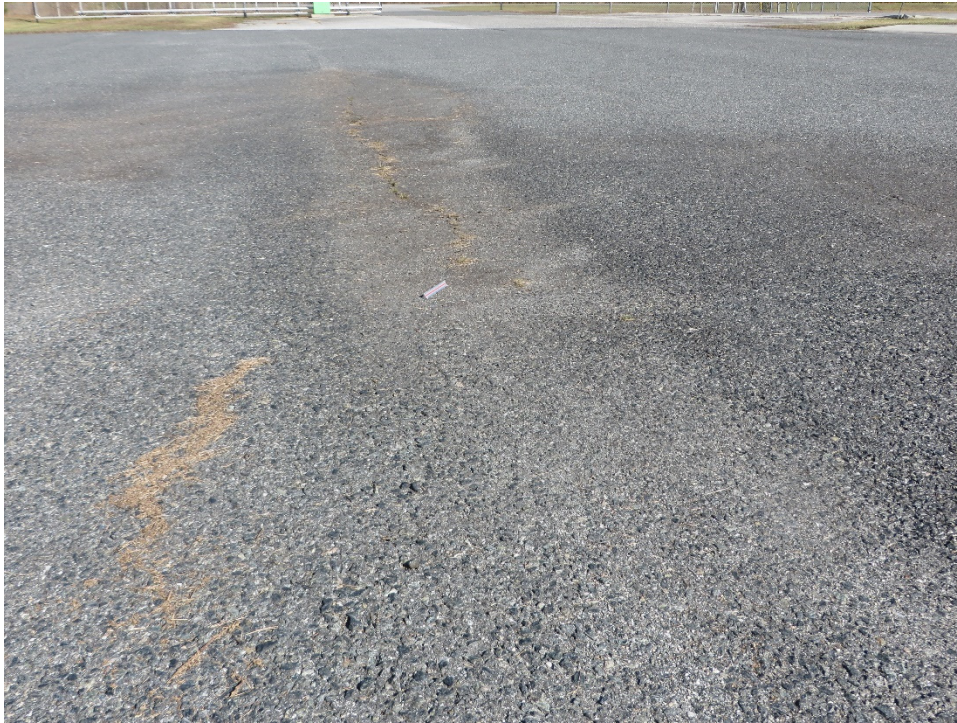
A01HO-20. Rutting (Sample Unit No. 01).
