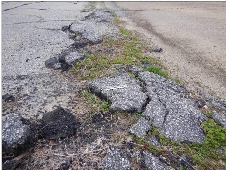
FIGURE H-8 HIGH-SEVERITY SHOVING AT AC/PCC INTERFACE
