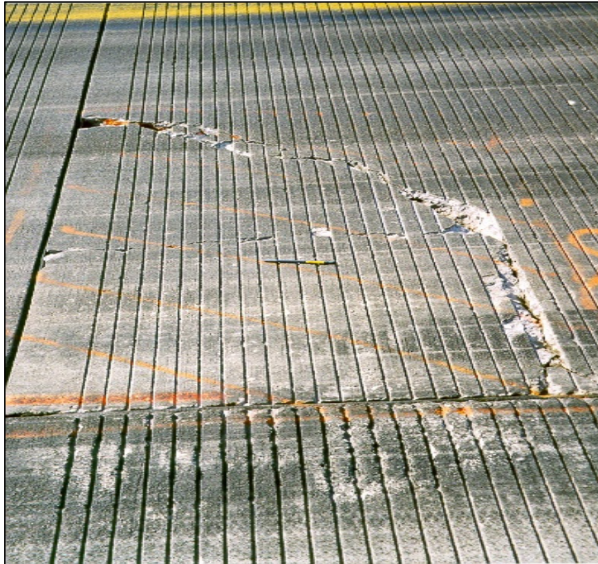
FIGURE H-11 HIGH-SEVERITY CORNER BREAKING
