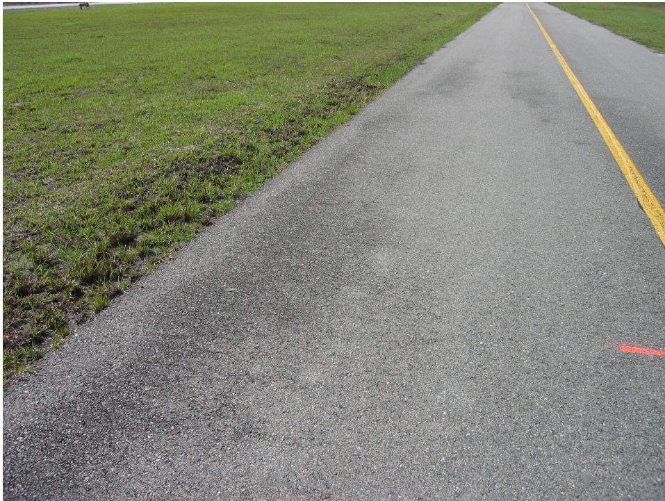
TAHO-10. Raveling and weathering.
