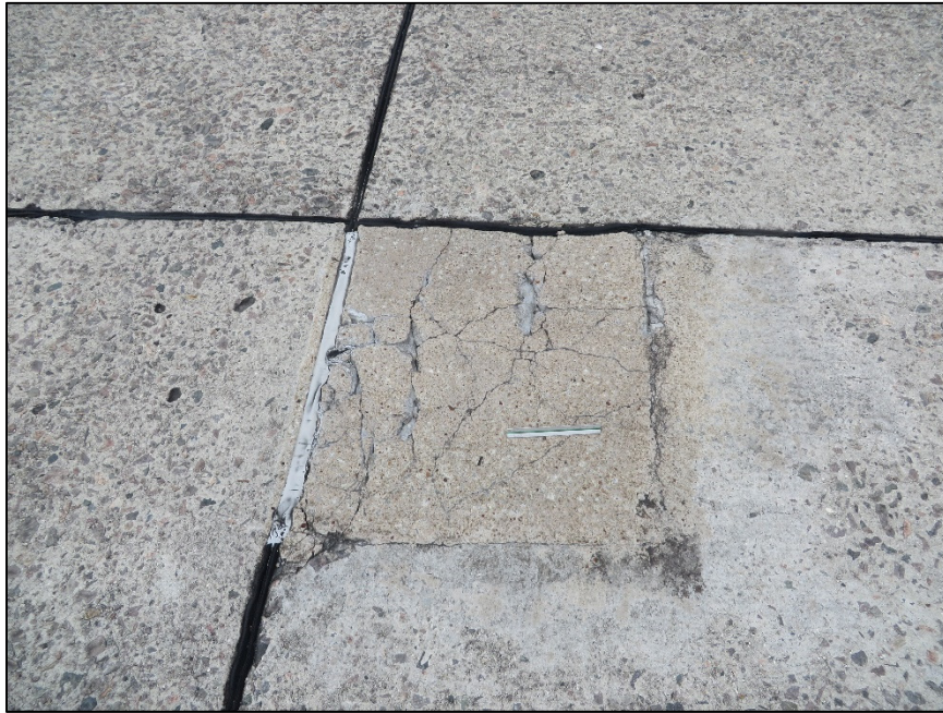
FIGURE H-14 HIGH-SEVERITY PATCHING
