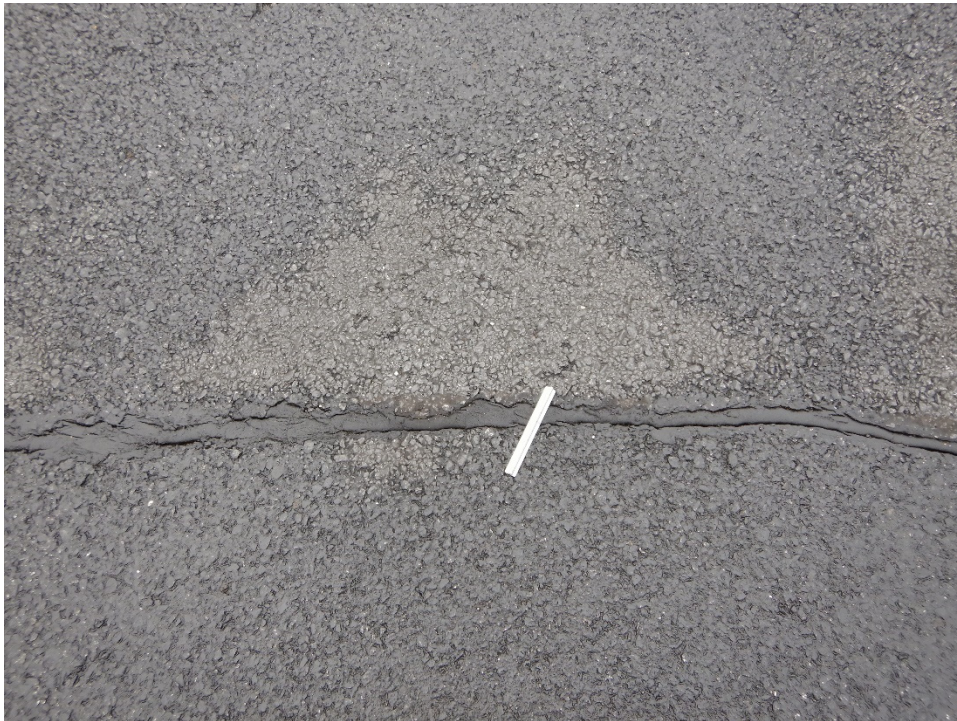
A01ES-10. L&T Cracking (Sample Unit No. 04).
