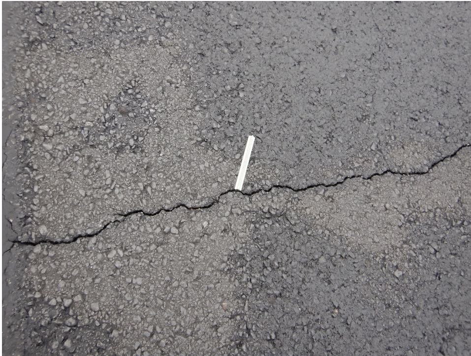
TBES-10. L&T Cracking (Sample Unit No. 03).
