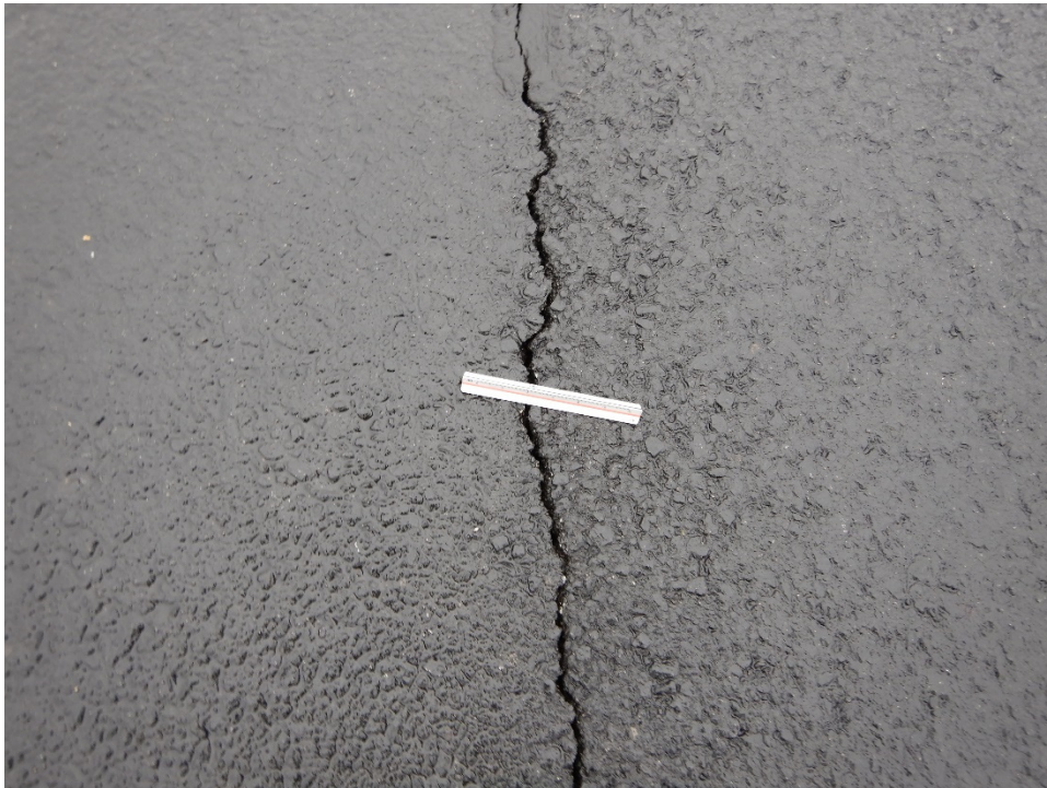
TAES-10. L&T Cracking (Sample Unit No. 93).
