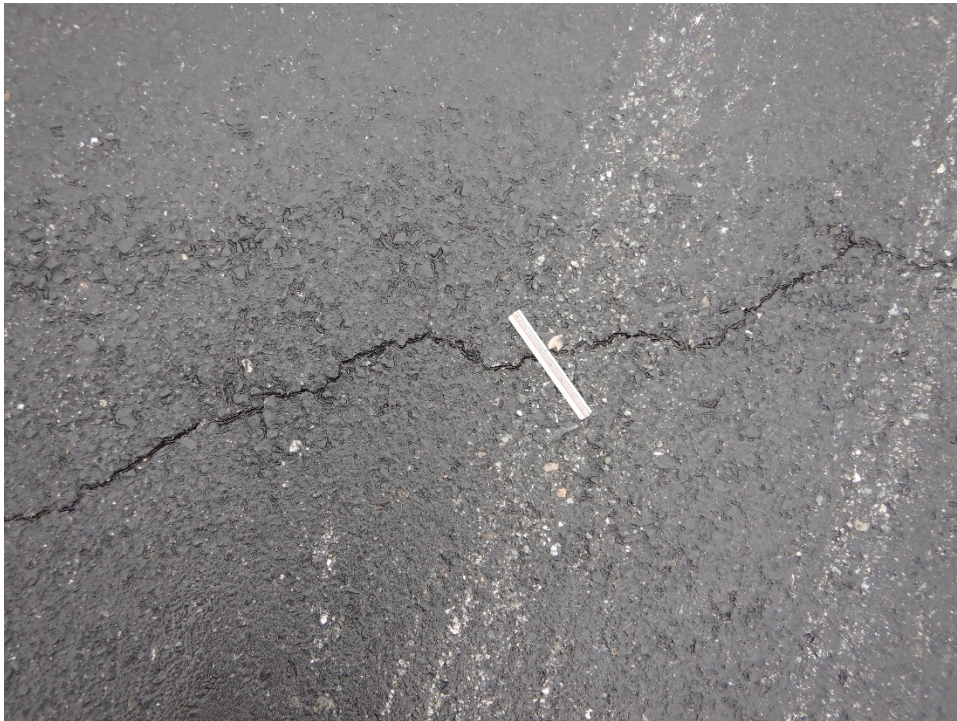
A01ES-20. L&T Cracking (Sample Unit No. 02).
