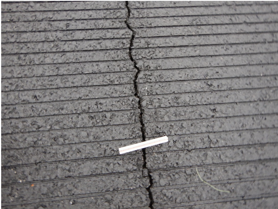
R220ES-10. L&T Cracking (Sample Unit No. 125).
