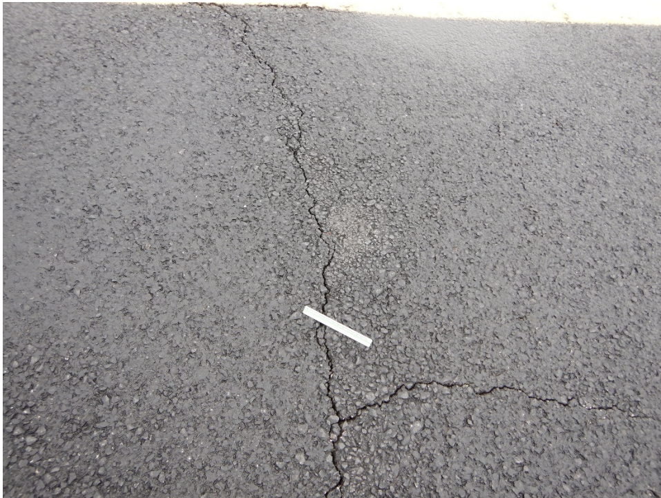
TEES-10. L&T Cracking (Sample Unit No. 04).
