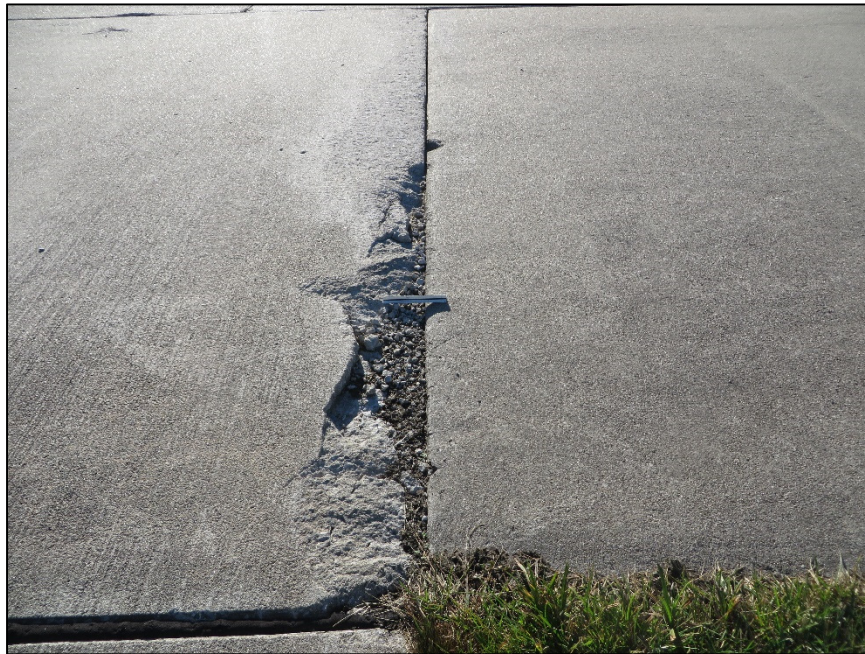
FIGURE H-18 HIGH-SEVERITY JOINT SPALLING
