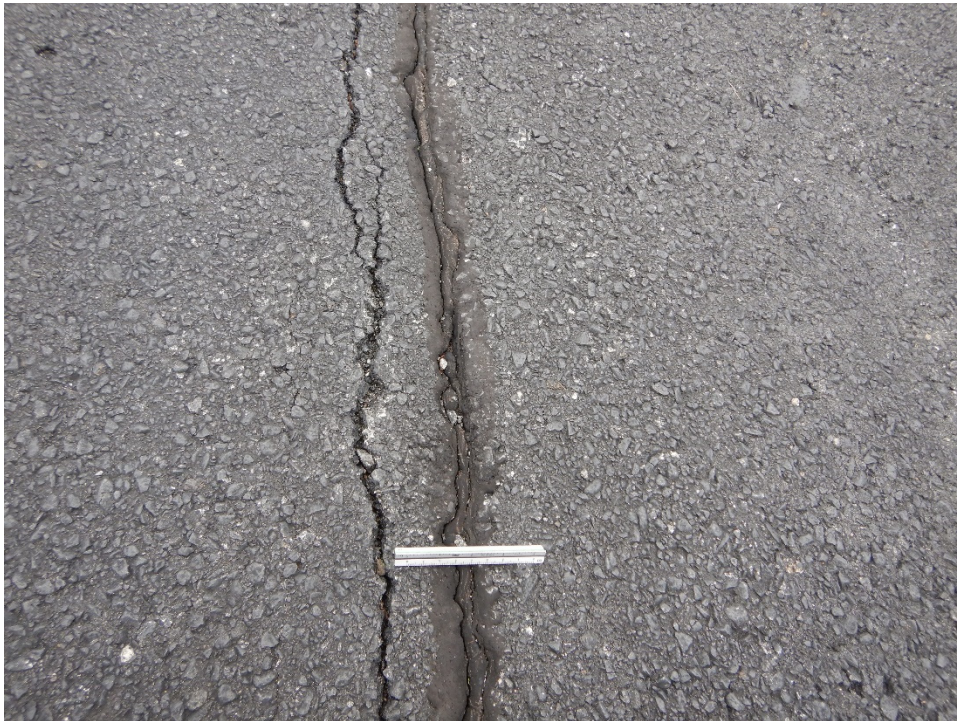
THANGES-10. L&T Cracking (Sample Unit No. 02).
