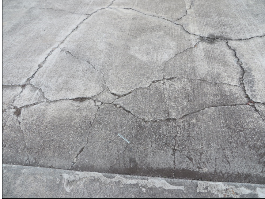
FIGURE H-17 HIGH-SEVERITY SHATTERED SLAB
