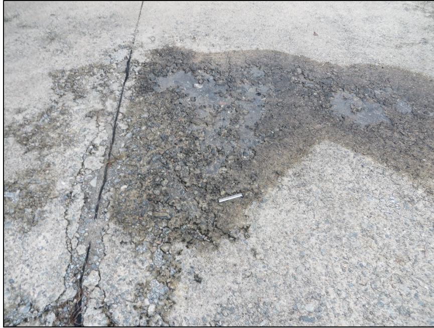
FIGURE H-15 HIGH-SEVERITY SCALING
