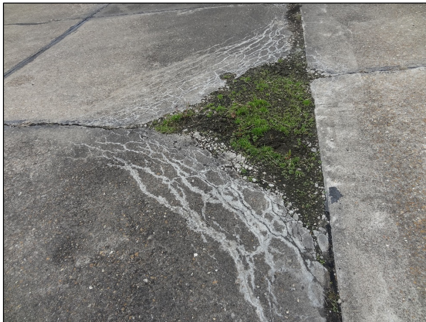
FIGURE H-20 HIGH-SEVERITY ASR
