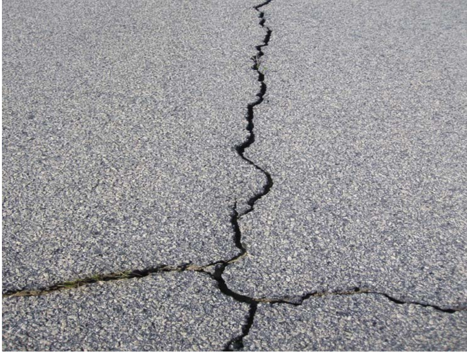
TAWB-10. Longitudinal and Transverse Cracking (Sample Unit #02).
