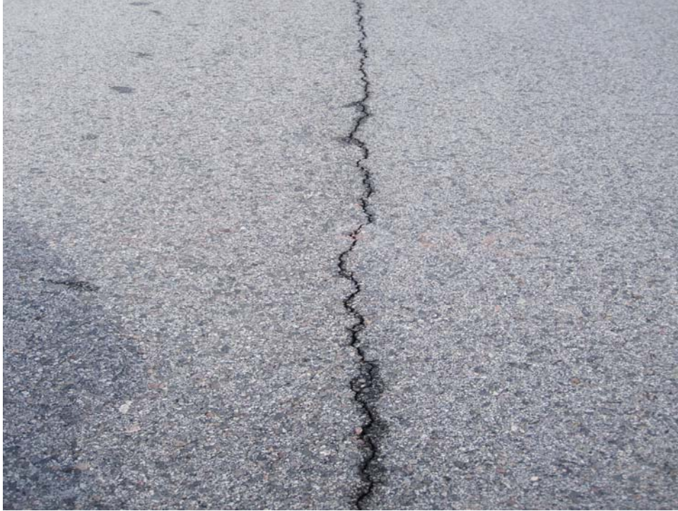
R826WB-10. Longitudinal and Transverse Cracking (Sample Unit #50).
