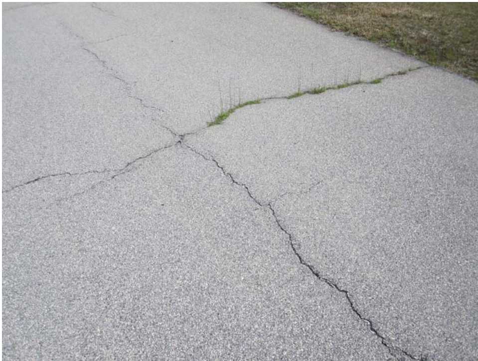
R826WB-10. Longitudinal and Transverse Cracking (Sample Unit #14) (2).
