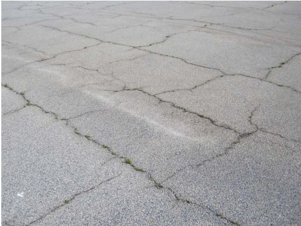
A01WB-10. Block Cracking (Sample Unit #06).
