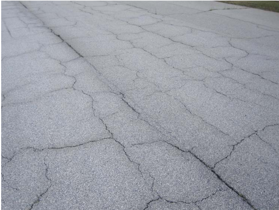
R826WB-10. Block Cracking (Sample Unit #05).
