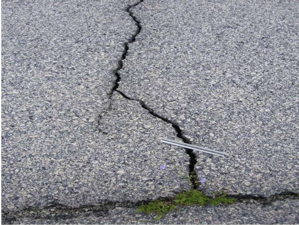
R826WB-10. Longitudinal and Transverse Cracking (Sample Unit #14) (1).
