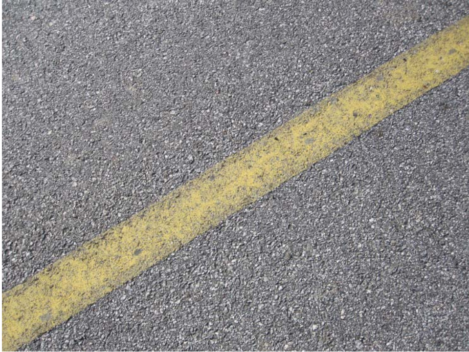
THANGML-10. Unsatisfactory Paint.
