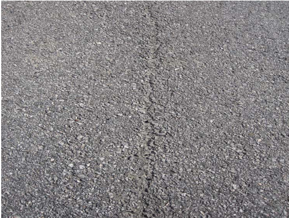
THANGML-10. Longitudinal and Transverse Cracking (Sample Unit #01).
