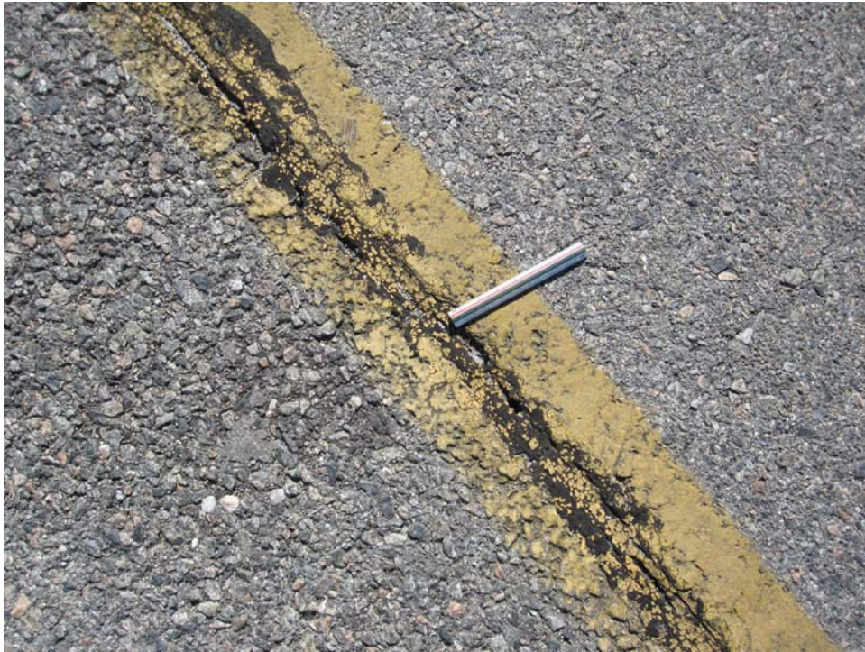
TAHO-10. Longitudinal and Transverse Cracking (Sample Unit #25).
