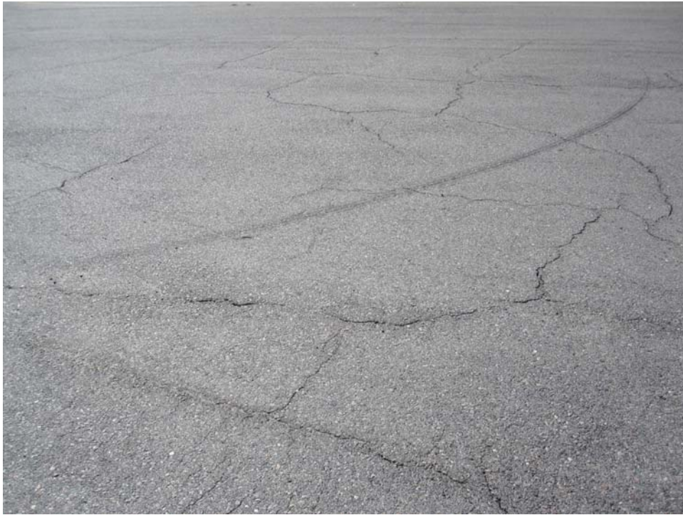
A01HO-10. Block Cracking (Sample Unit #03).
