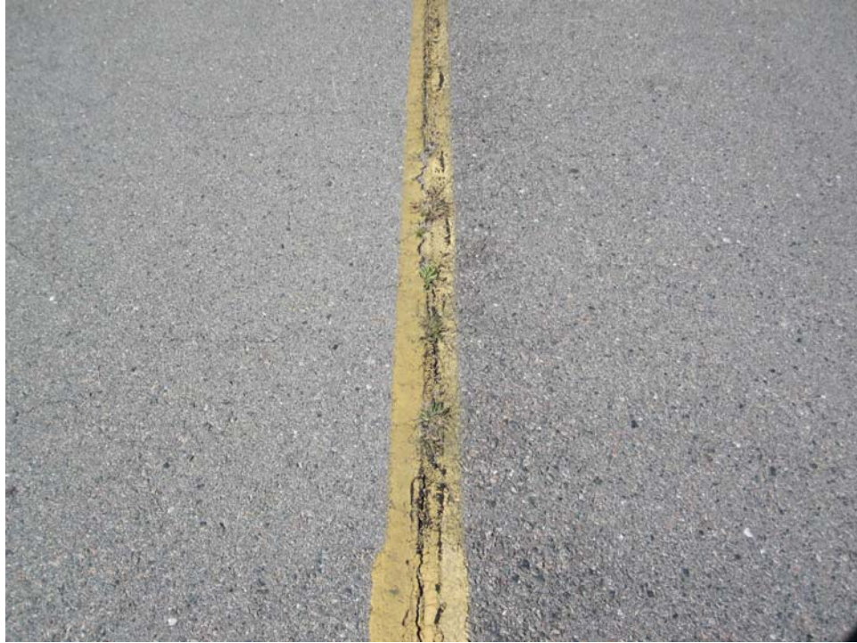
TAHO-10. Unsatisfactory Paint.
