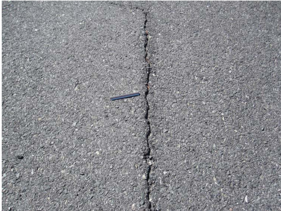
A01HO-20. Longitudinal and Transverse Cracking (Sample Unit #02).
