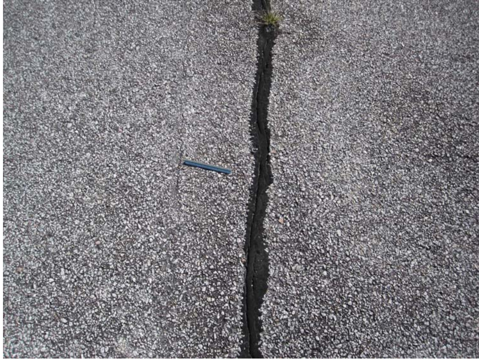
R1432HO-10. Longitudinal and Transverse Cracking (Sample Unit #06).
