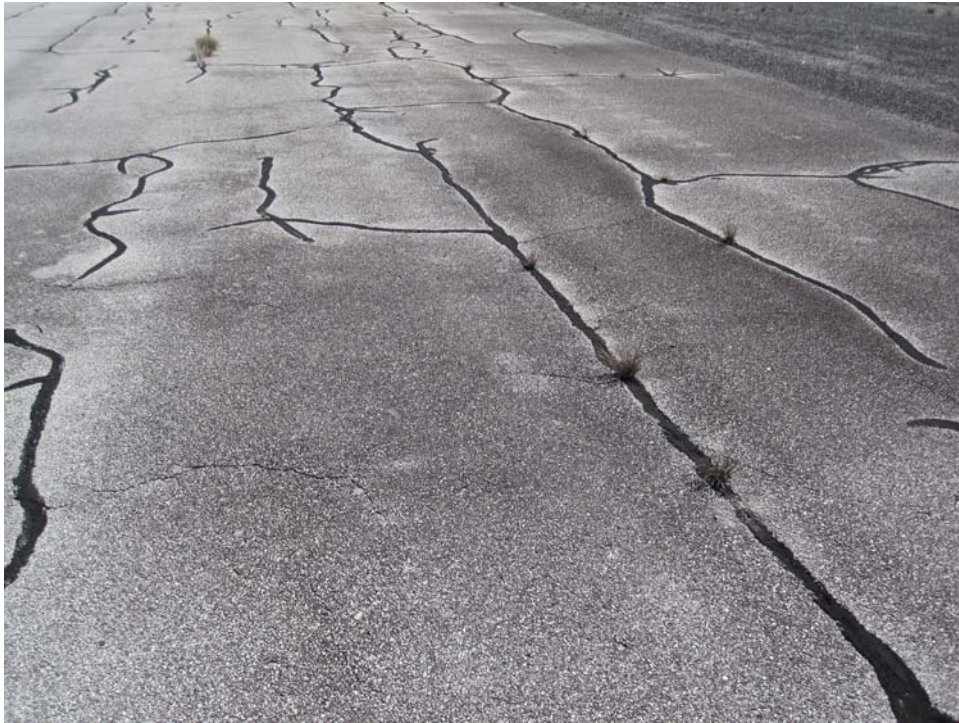
R1432HO-10. Block Cracking (Sample Unit #06).
