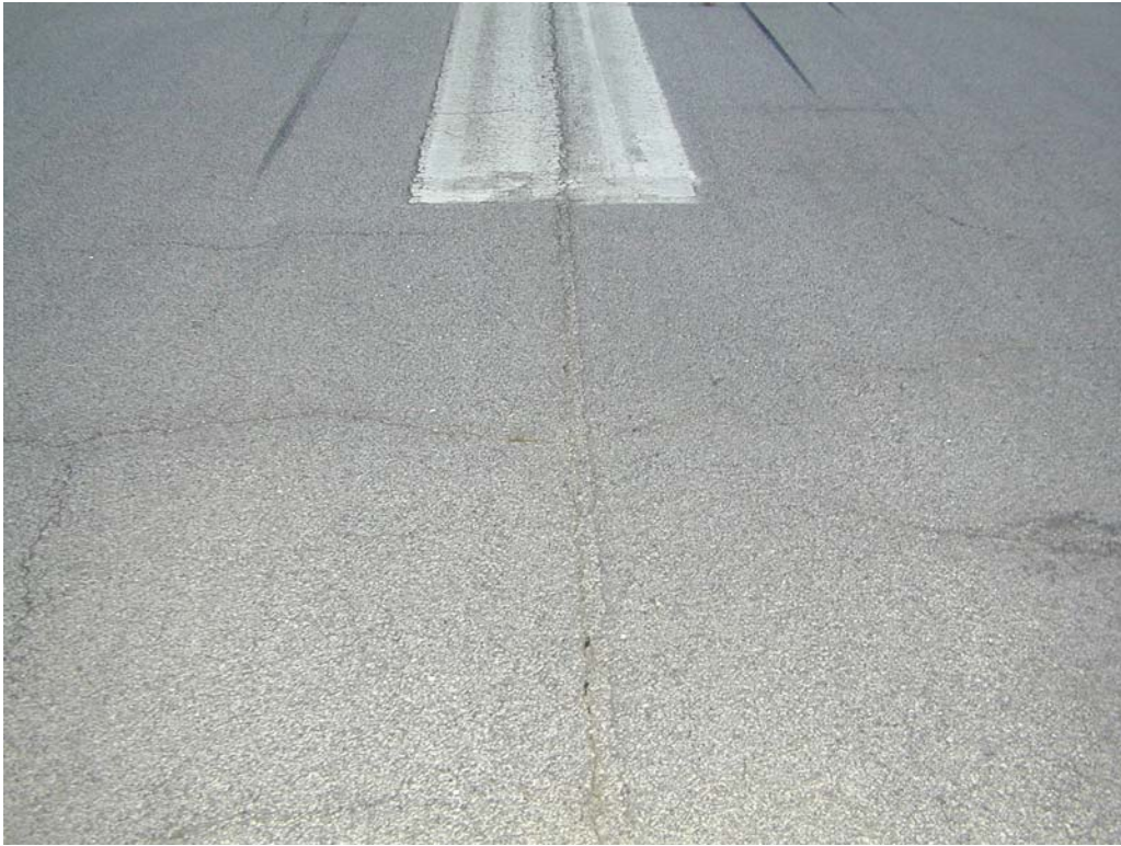
Block cracking in section R826WB-10.
