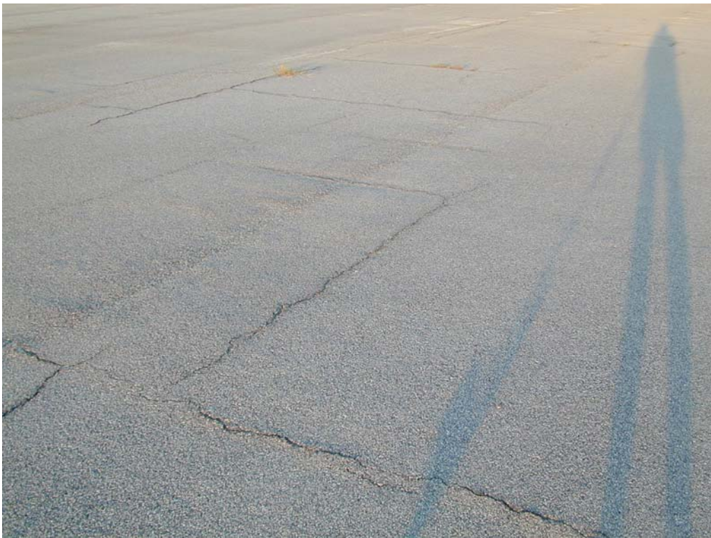
Block cracking in section A01WB-10.
