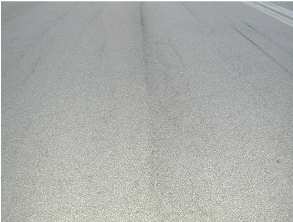
Alligator cracking in section R826WB-10.
