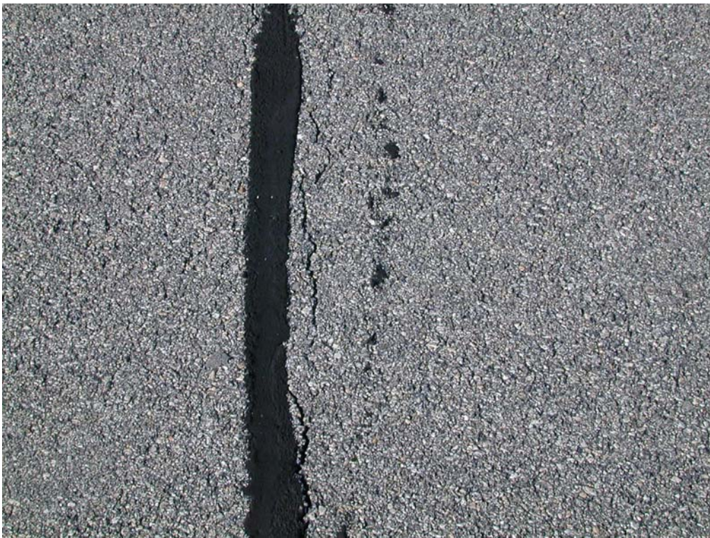
L&T cracking in section R1735ML-10.
