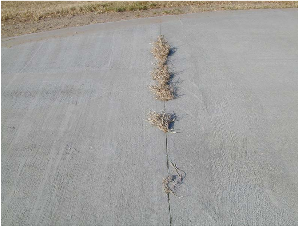
Joint seal damage in section R1735ML-30.
