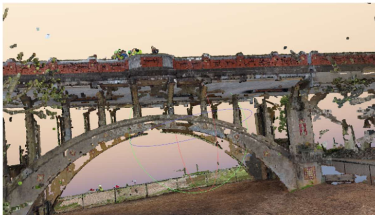
Partial 3D model of the Piedmont Park Bridge generated using Pix4D software.
