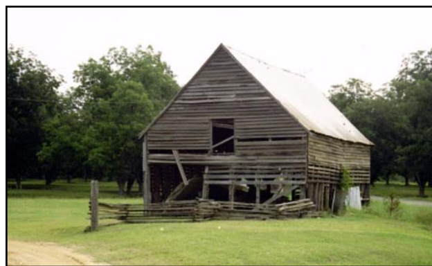
This deteriorating barn in Sumter County may be eligible as a contributing resource to a district that includes the land of its former plantation.
