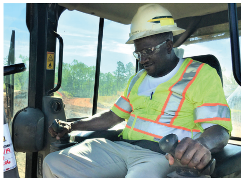
As Project Superintendent James Smith grades the future roadway, the GPS system in his bulldozer ensures he's sticking to level specifications.
