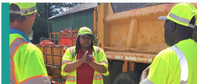
Assistant Area Maintenance Engineer Eureika Thomas dispatches a work crew to reopen a lane closed due to guardrail repair.
