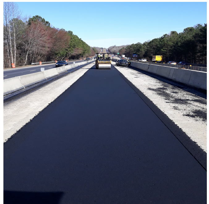
The I-85 Widening project adds one lane in each direction from Hamilton Mill Road in Gwinnett County to SR 53 in Jackson County. To mitigate right-of-way impacts, paving is occurring inside of the existing roadway for the new lanes.
