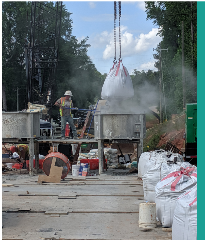
Contractors use UHPC on the Elliott Road over Walnut Creek Bridge project in Henry County that opened in May 2019.
