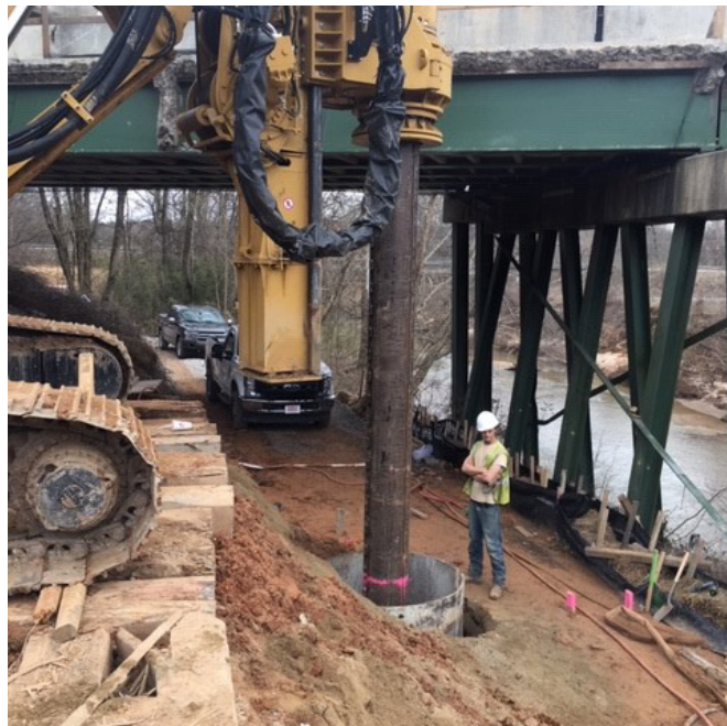
Workers are drilling to install new posts at the Mulberry River bridge, a mainline bridge at the Barrow/Jackson county line. Three overpass bridges are also being replaced as part of the I-85 Widening project.
