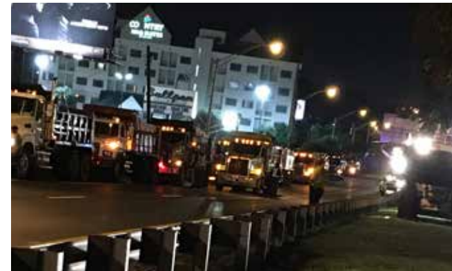
To limit delays and driver inconvenience, much of the repaving work on Metro Atlanta interstates is performed at night. Photo: C.W. Matthews Contracting Co.
