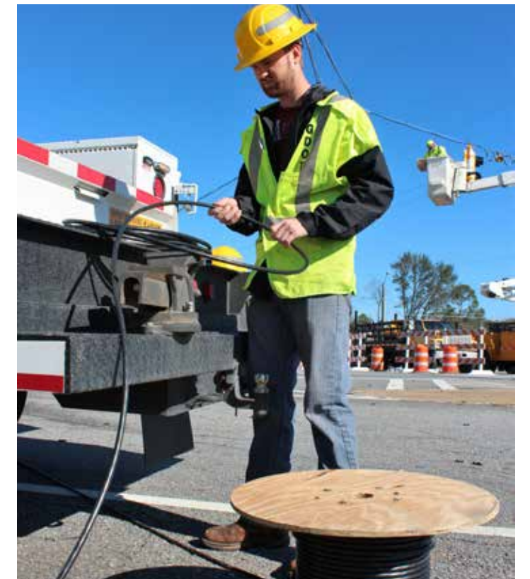
Georgia DOT Signal Technician Kyle Griffin repairs signals in Albany. Photo: Lisa Rodriguez-Presley, GEMA/HS
