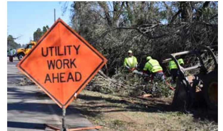
Cutting large tree limbs for removal from a state route right of way in Dougherty County. Photo: Kyle Collins, GDOT
