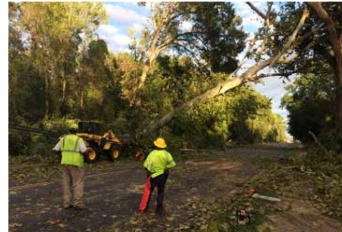
Cleaning up. Once water receded, power companies addressed downed lines, and it was determined safe to enter damaged areas, Georgia DOT crews removed trees and cleared roadways. 795 Georgia DOT personnel deployed to address damage from the hurricane. Photo: Kyle Collins, GDOT
