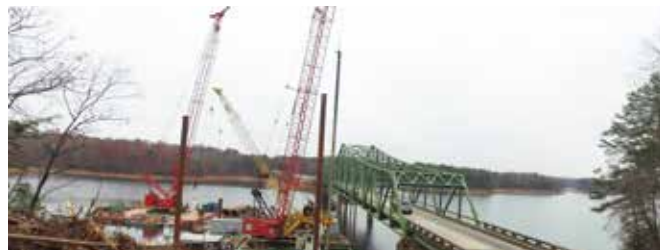
The new bridge is being built next to the aging "big green bridge," which will be demolished after the replacement is completed. Photo: Katie Strickland, GDOT
