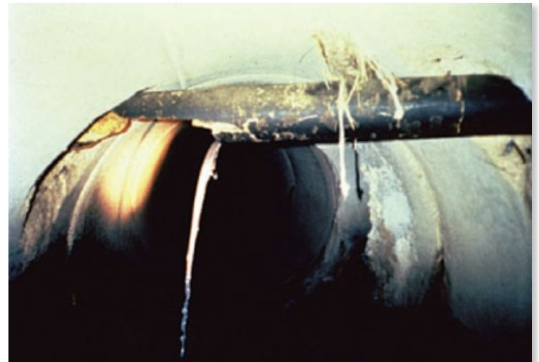
Broken sewer pipe
