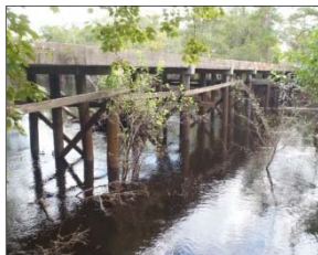
Example of LOCBR candidate - wooden piles with helper bracing (this bridge is closed).
