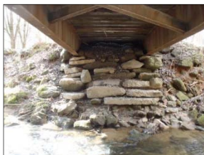
Typical LOCBR project substandard super and substructure
