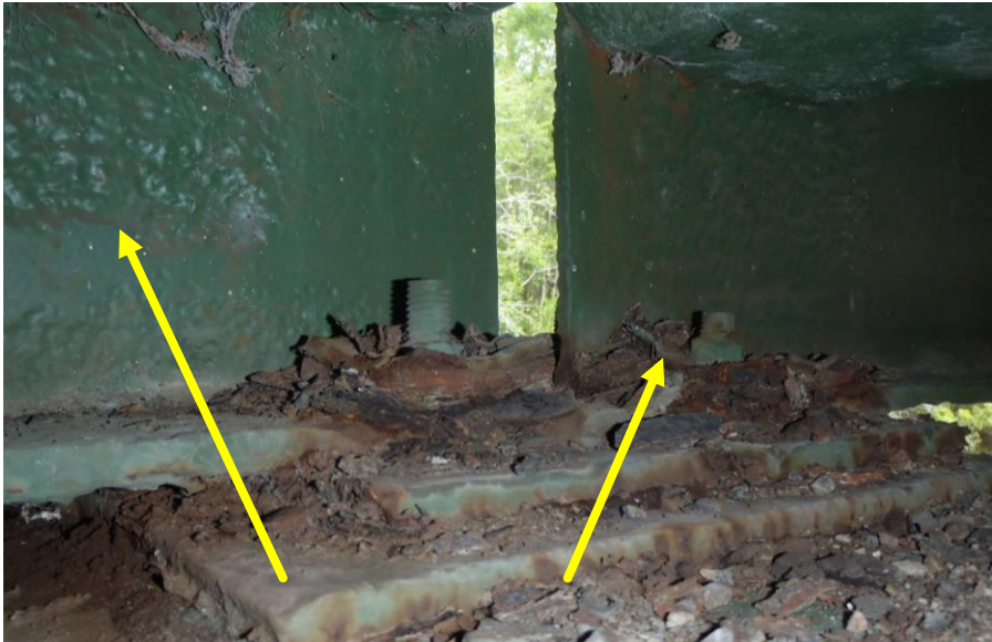
Pitting & Pack Rust
