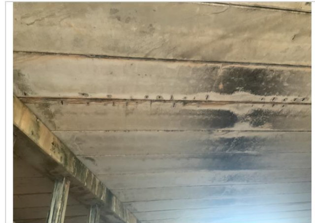
Typical exposed rebar in deck panels. 2022
