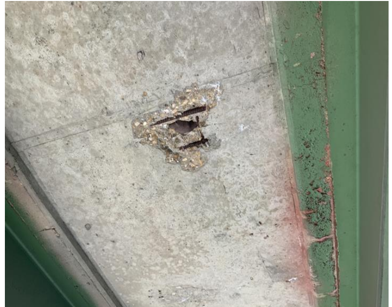
Spall with Exposed Rebar
