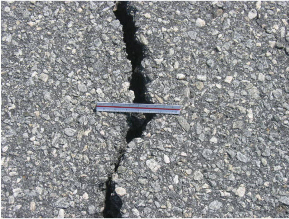
TFVL-20. L&T cracking.
