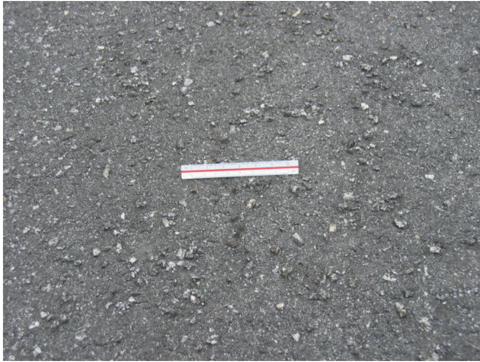
TCVL-10. Raveling and weathering.
