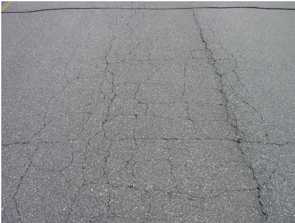
TAMR-10. Alligator cracking.
