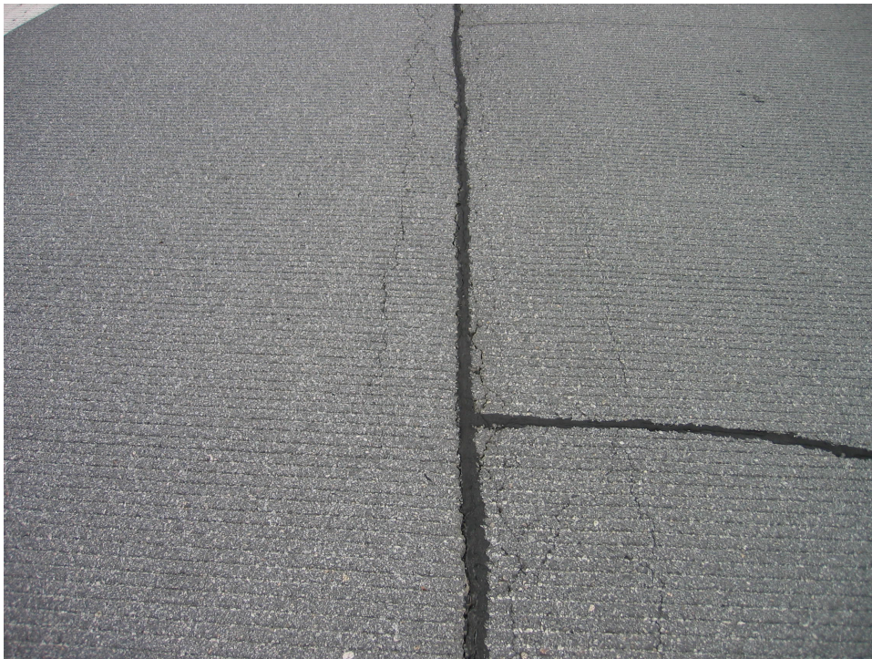
R927MR-10. L&T cracking.
