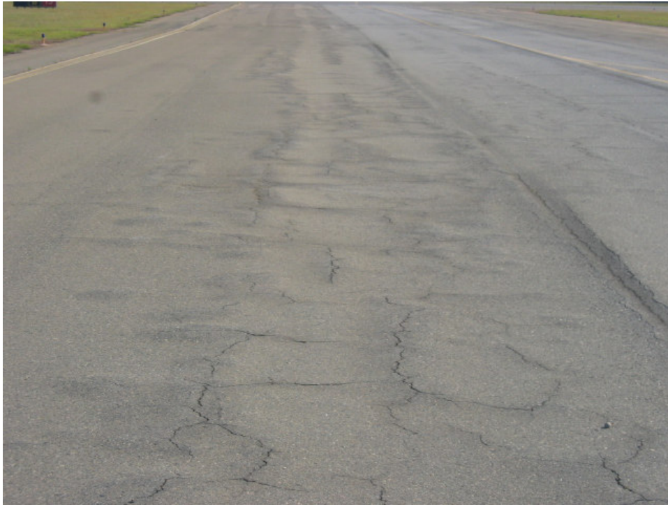
TBMGRA-10. Block cracking.
