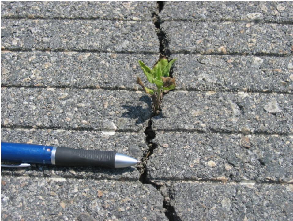
R0523MGRA-10N. L&T cracking.
