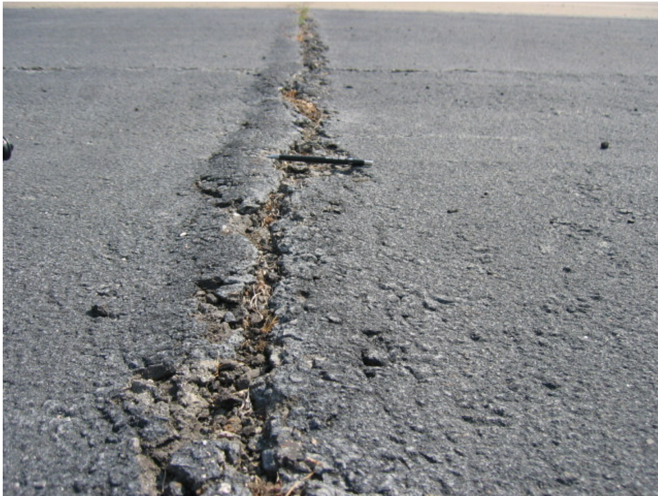
R1331MGRA-10S. L&T cracking (1).
