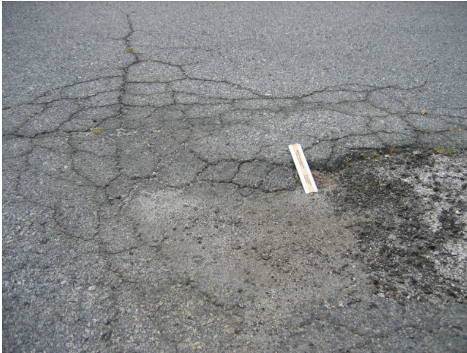
A01MGRA-80. Alligator cracking.
