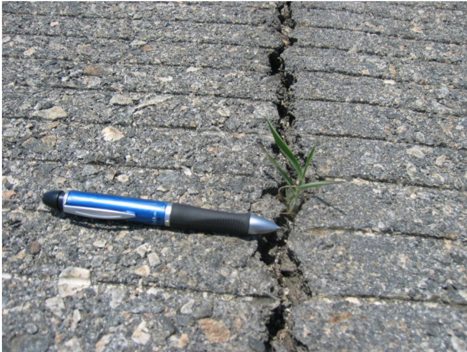
R0523MGRA-10S. L&T cracking.
