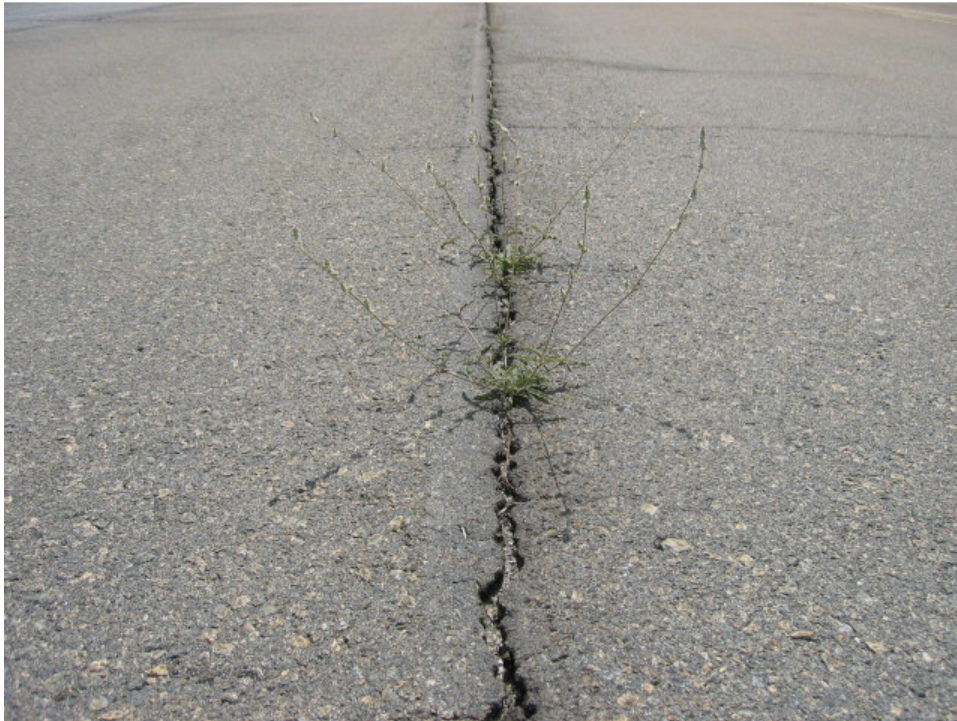
TAMGRA-10. L&T cracking.
