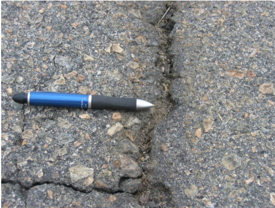
TCMGRA-20. L&T cracking.
