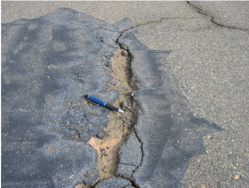
TCMGRA-10. L&T cracking.
