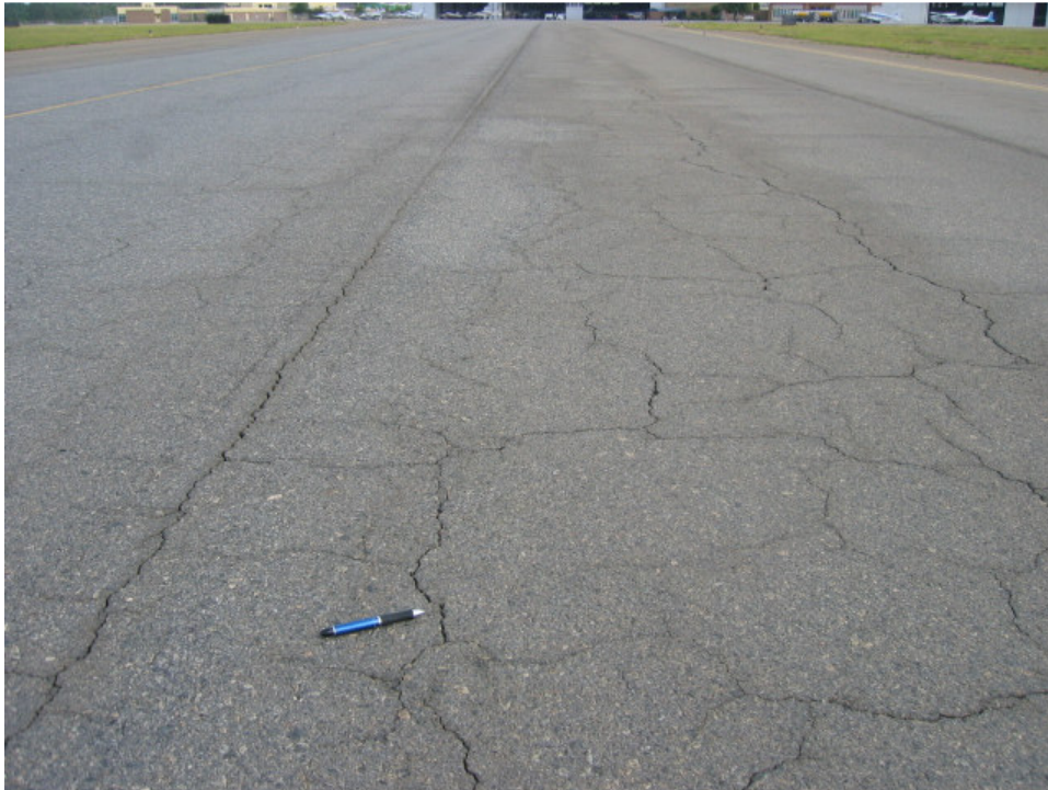
TCMGRA-10. Block cracking.
