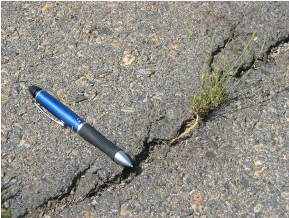
TBMGRA-30. L&T cracking.
