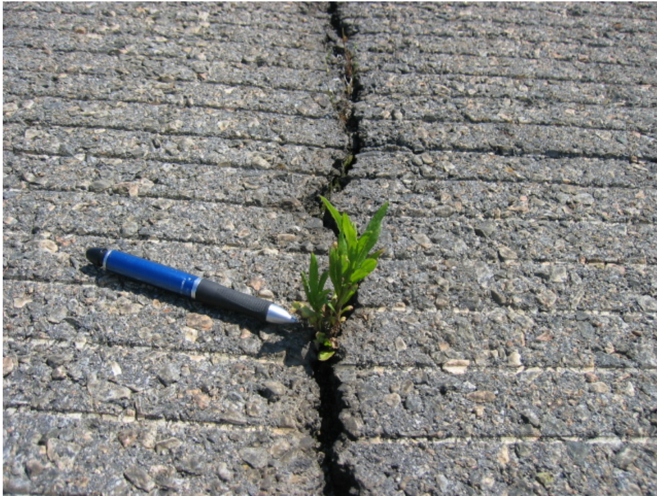
R0523MGRA-20C. L&T cracking.
