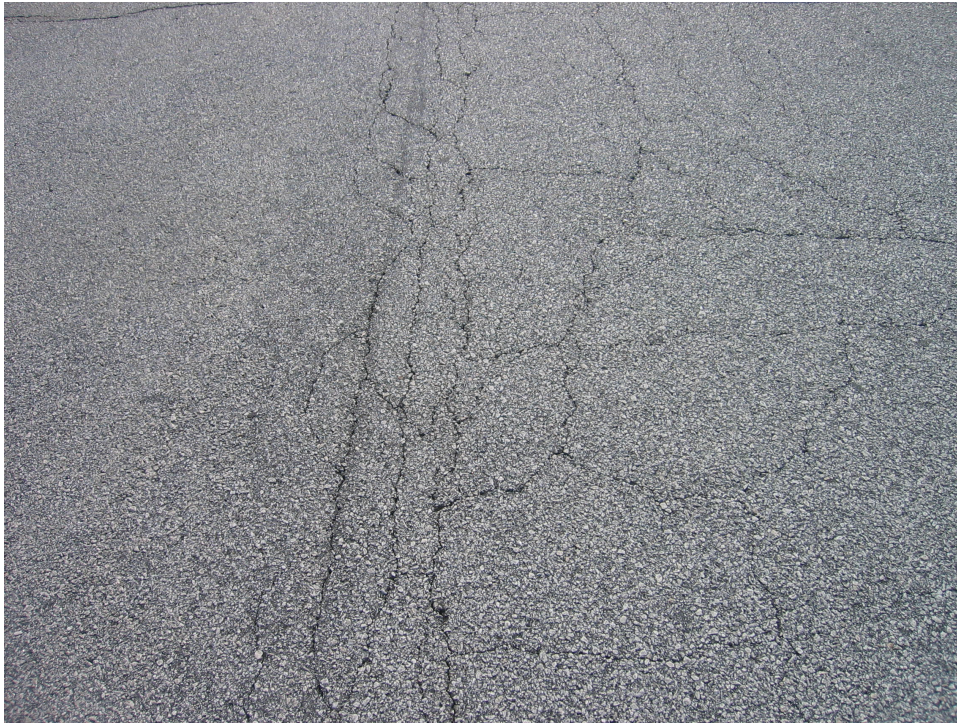
TIAB-10. Alligator cracking.
