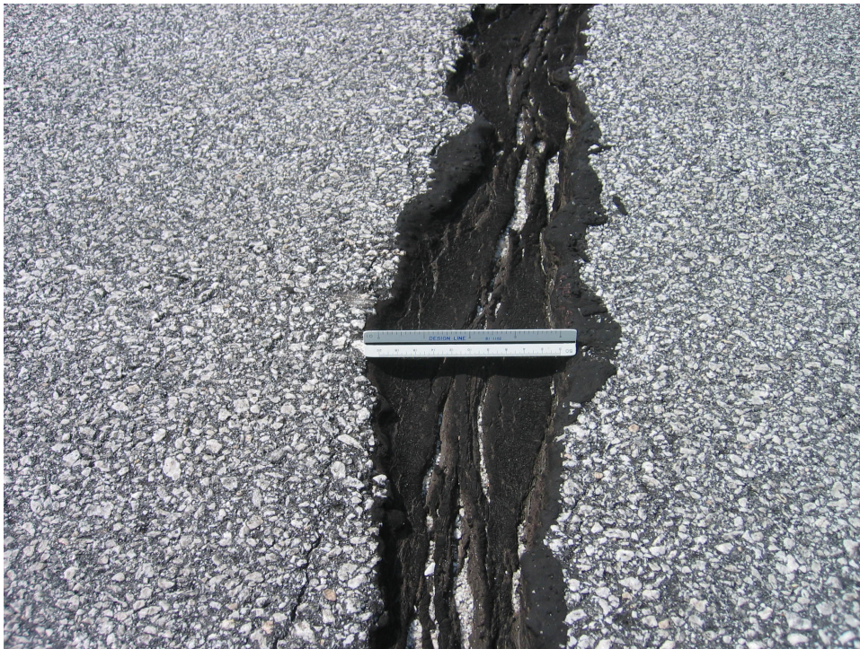
R927AB-10. L&T cracking.
