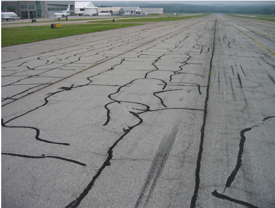
R1432AB-10. Block cracking.
