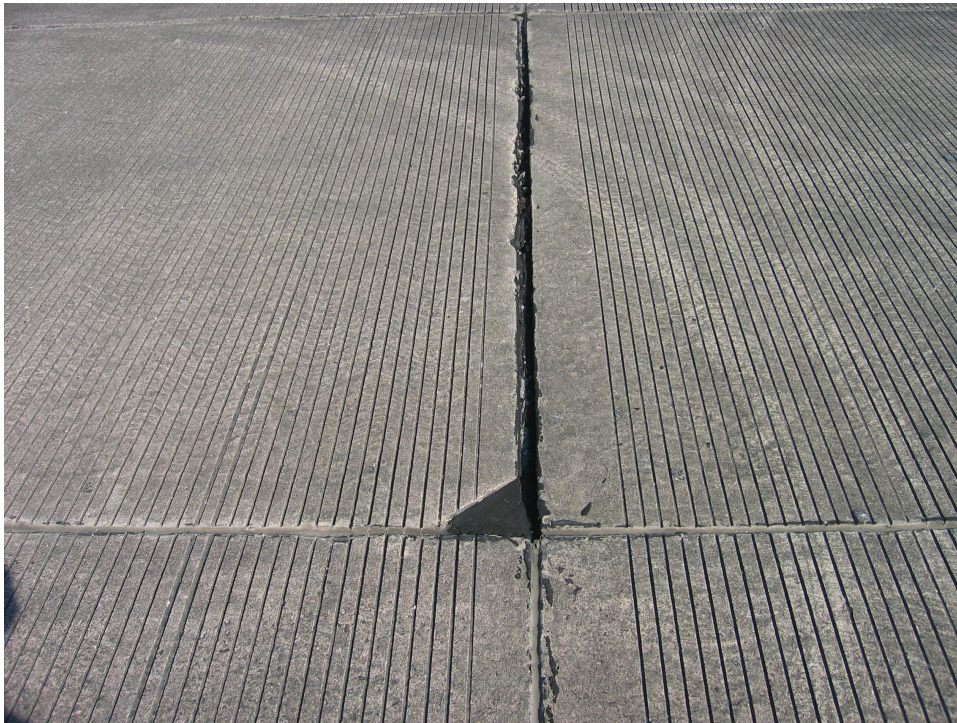
R725GJP-30C. Joint seal damage.
