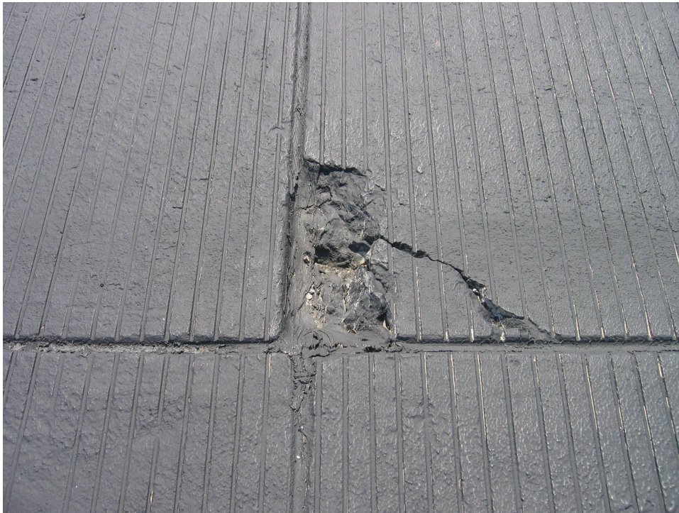
R725GJP-10S. Corner spall.
