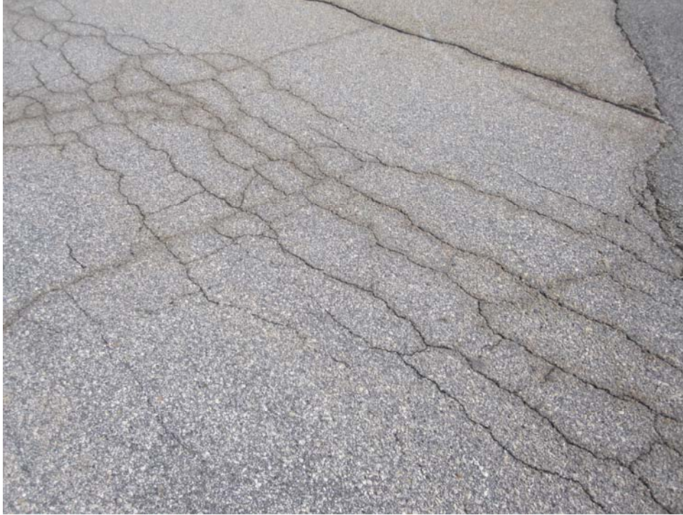
TAAT-30. Alligator Cracking (Sample Unit #06).
