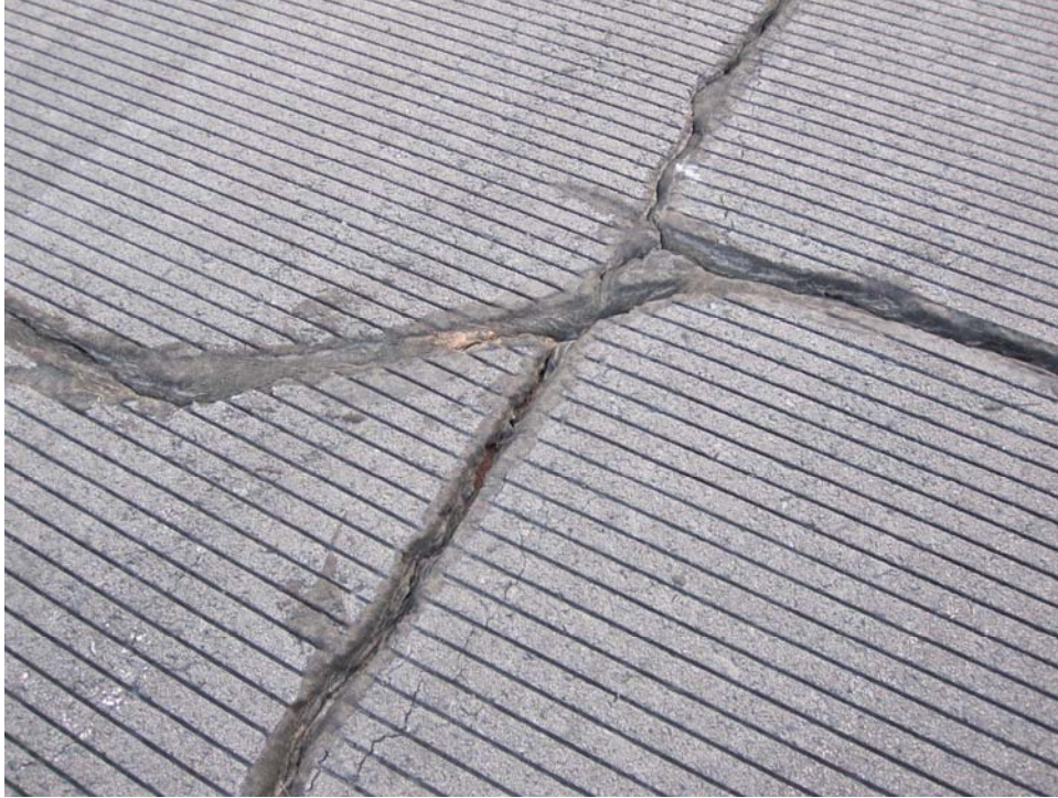
R927AT-10. Longitudinal and Transverse Cracking (Sample Unit #34).
