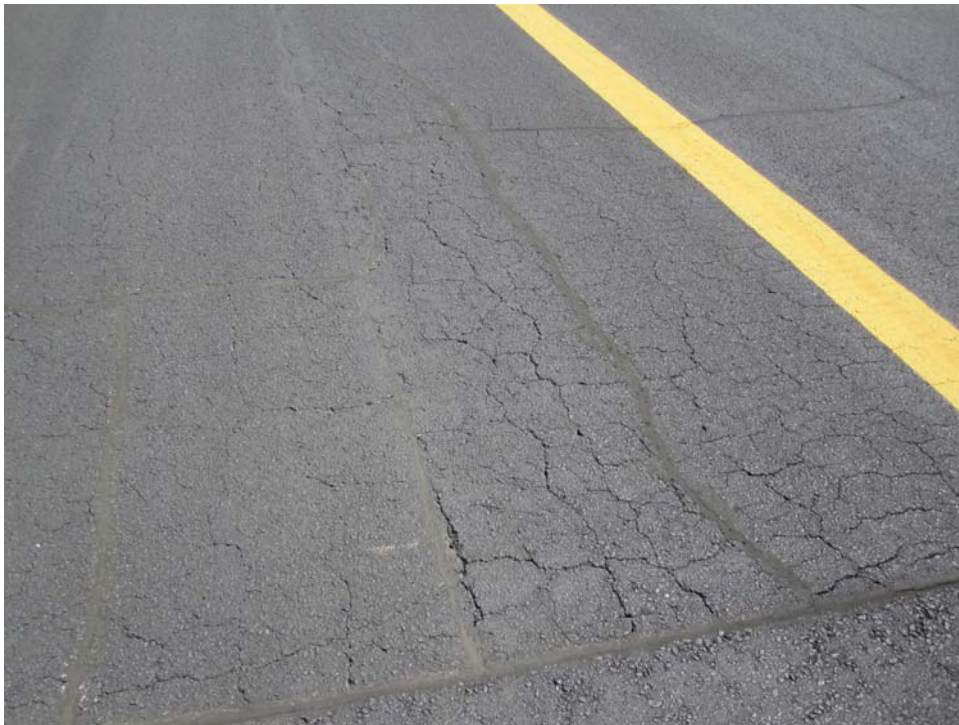
TAAT-20. Alligator Cracking (Sample Unit #24).
