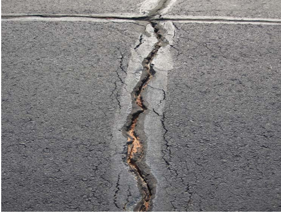
R220AT-10. Longitudinal and Transverse Cracking (Sample Unit #11).
