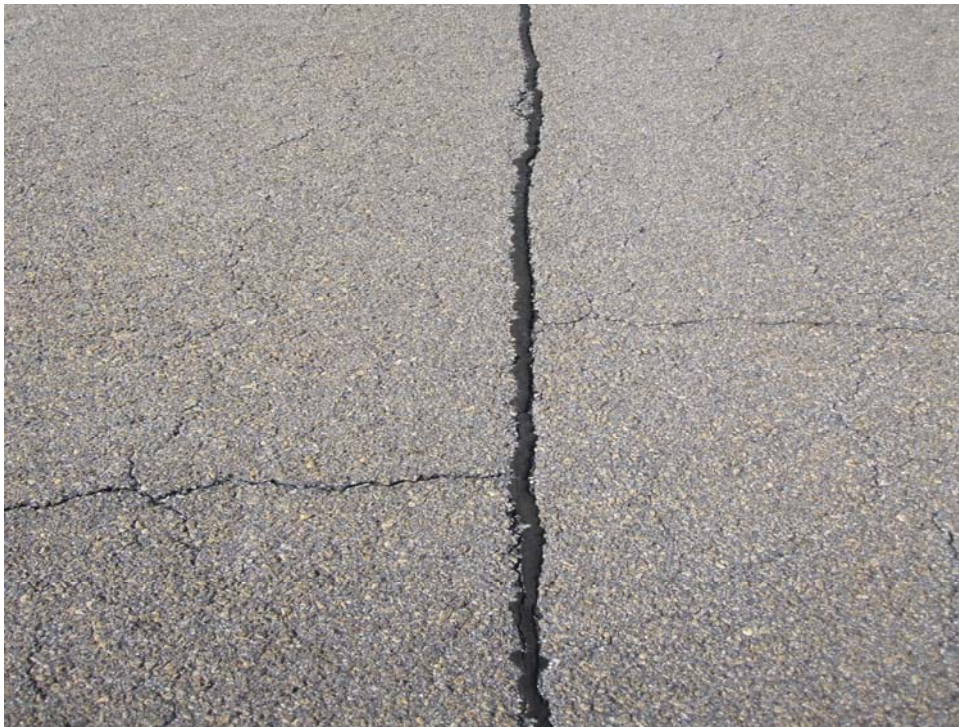
TBAT-10. Longitudinal and Transverse Cracking (Sample Unit #02).
