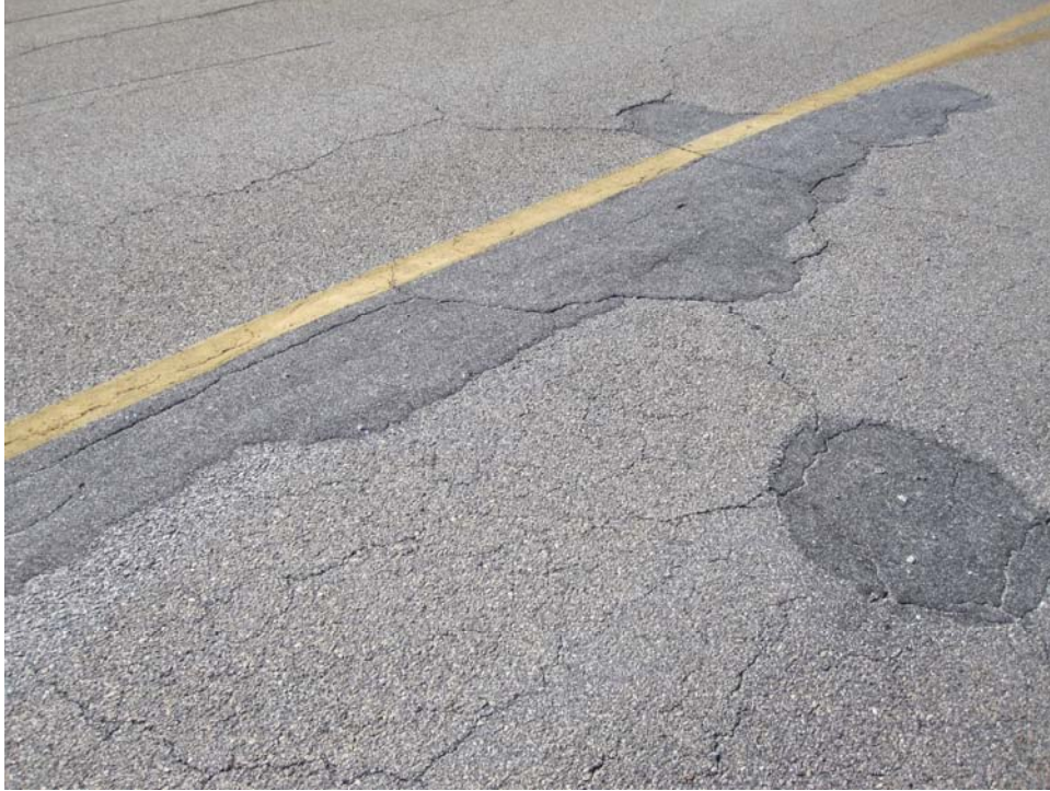
TBAT-10. Patching (Sample Unit #06).
