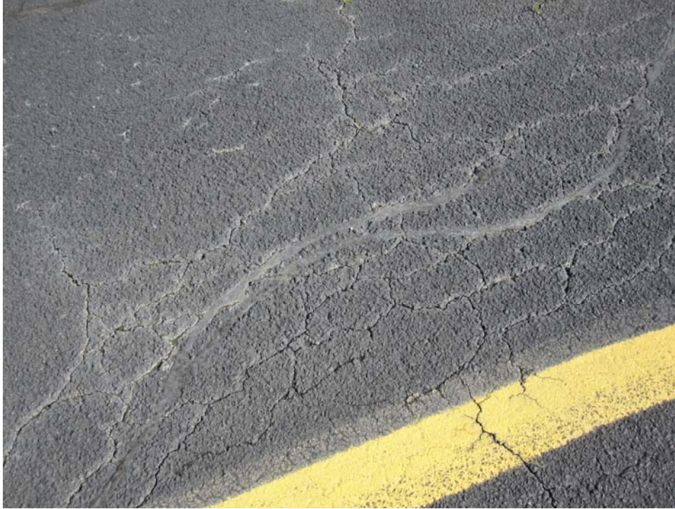
TBAT-30. Alligator Cracking (Sample Unit #02).
