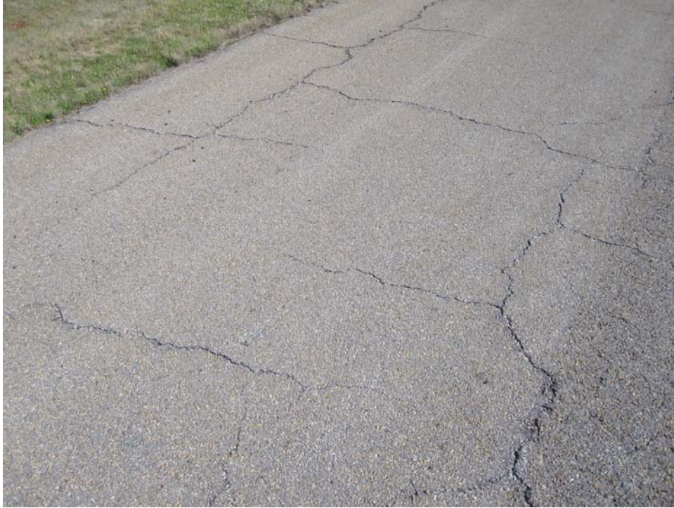
TBAT-10. Block Cracking (Sample Unit #02).
