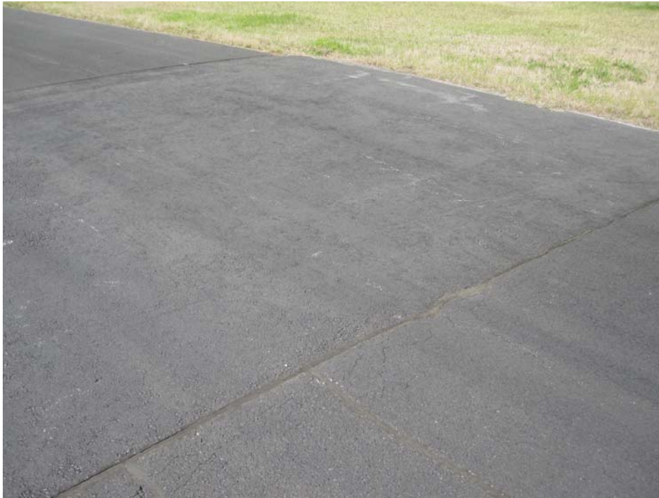
TAAT-20. Patching (Sample Unit #24).
