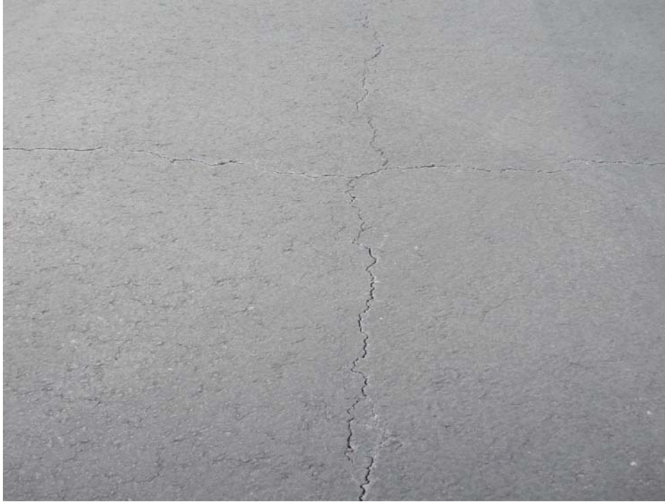
A01AT-20. Longitudinal and Transverse Cracking (Sample Unit #20).
