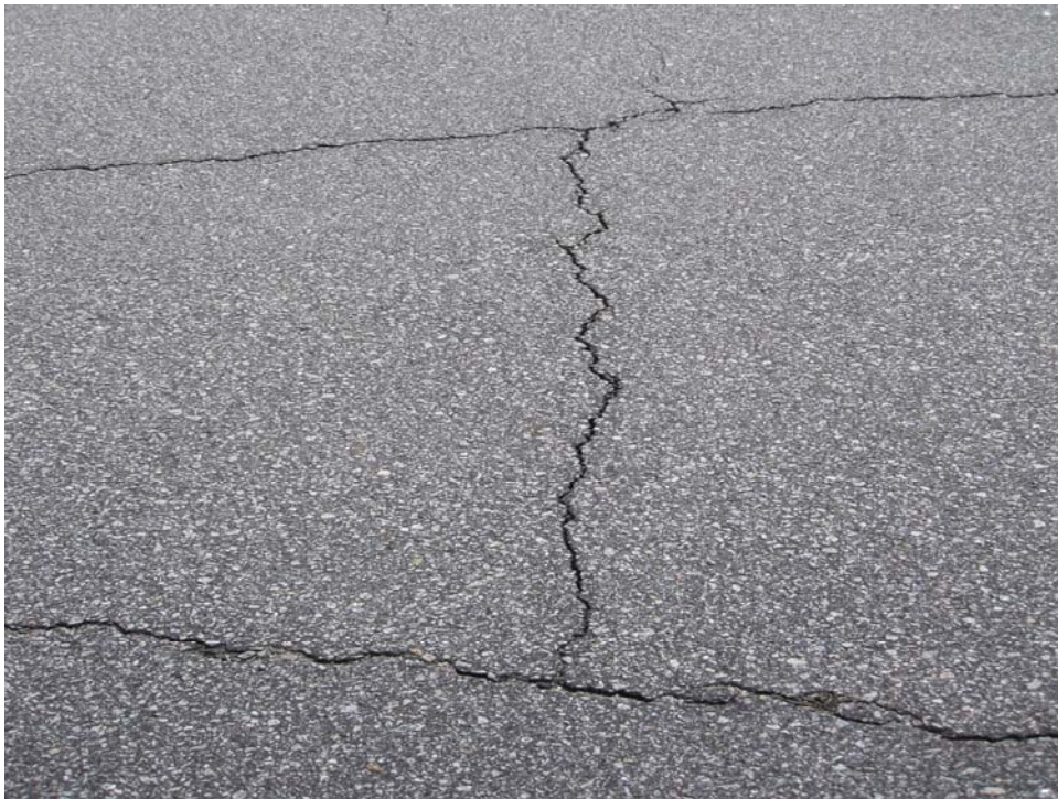
A01AT-20. Longitudinal and Transverse Cracking (Sample Unit #28).
