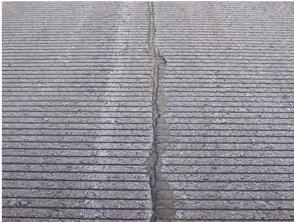
R927AT-10. Longitudinal and Transverse Cracking (Sample Unit #16).
