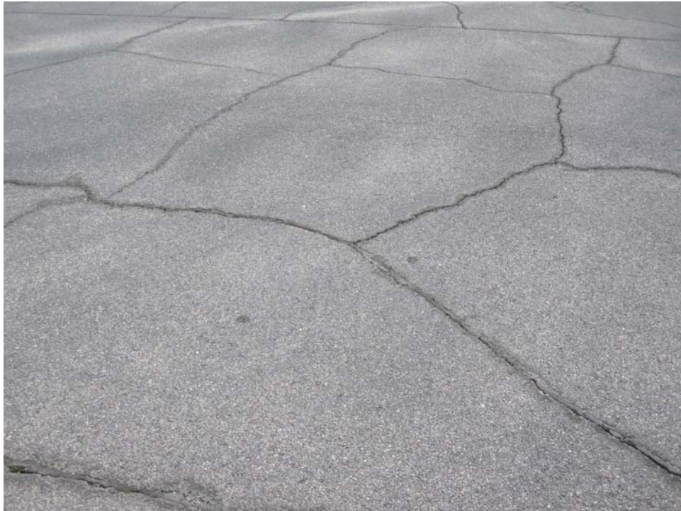
A01AT-10. Block Cracking (Sample Unit #03).
