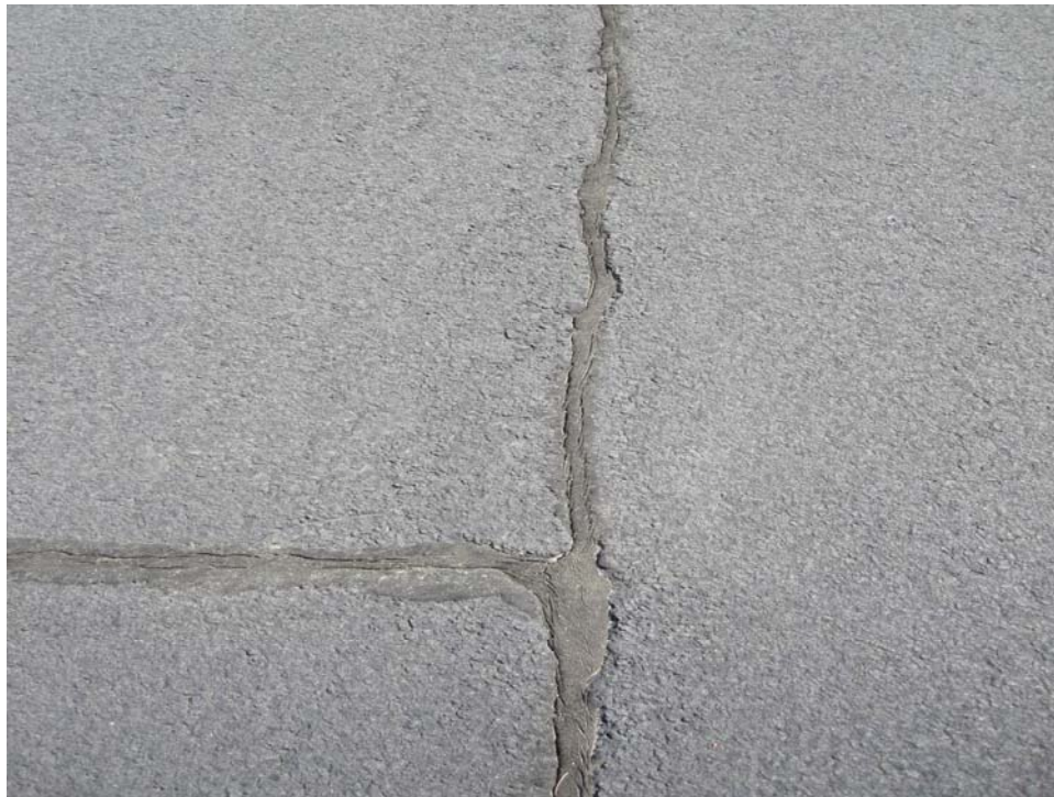
TAAT-10. Longitudinal and Transverse Cracking (Sample Unit #05).
