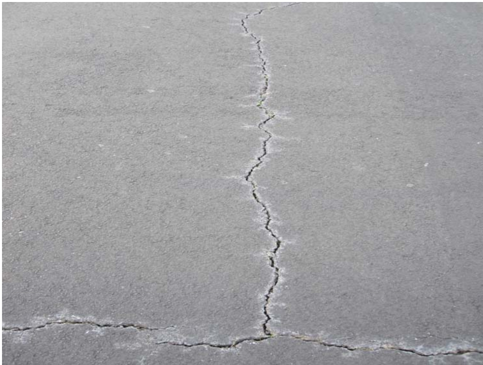
A01AT-20. Longitudinal and Transverse Cracking (Sample Unit #02).
