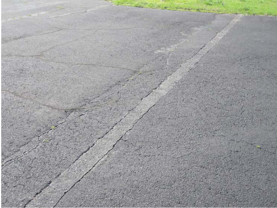
TBAT-30. Patching (Sample Unit #02).
