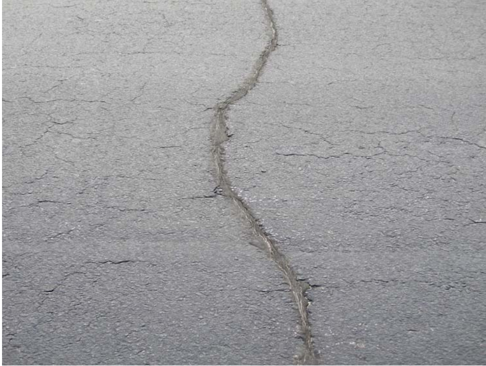
TAAT-20. Longitudinal and Transverse Cracking (Sample Unit #08).
