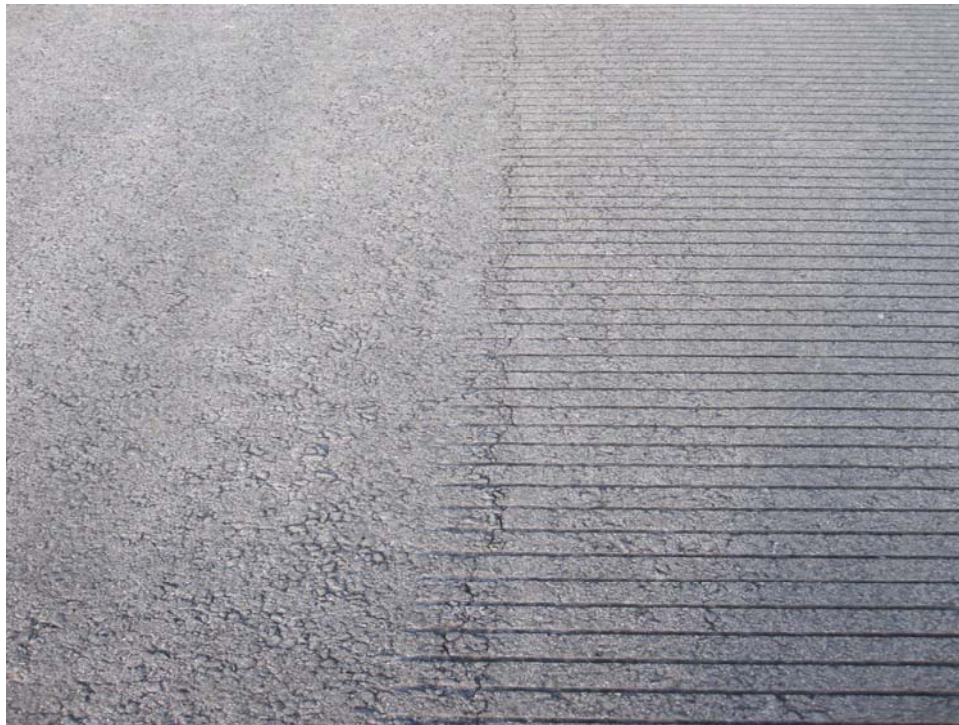
R927AT-20. Longitudinal and Transverse Cracking (Sample Unit #07).
