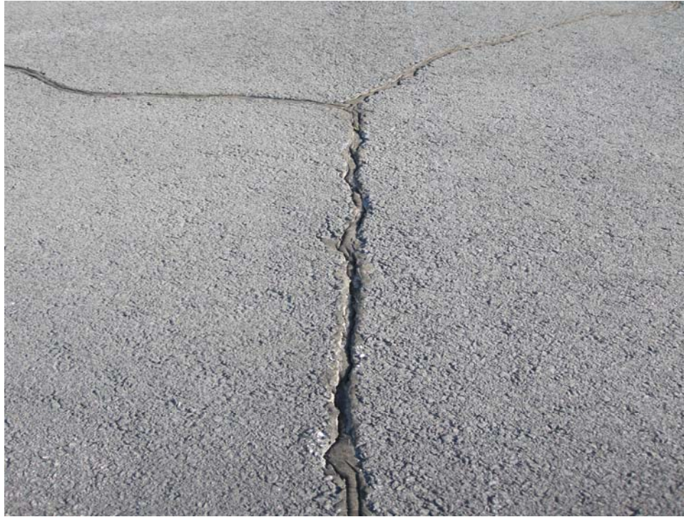
R220AT-20. Longitudinal and Transverse Cracking (Sample Unit #02).
