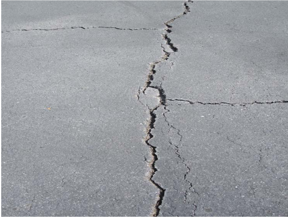
A01AT-30. Longitudinal and Transverse Cracking (Sample Unit #02).
