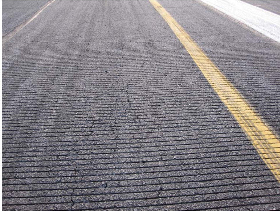
R927AT-10. Alligator Cracking (Sample Unit #25).
