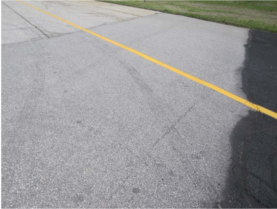
TAAT-30. Patching (Sample Unit #06).
