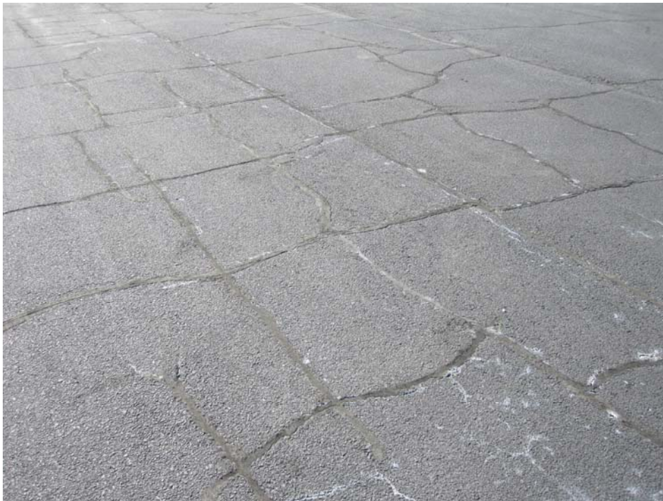
TBAT-15 Block Cracking (Sample Unit #04).
