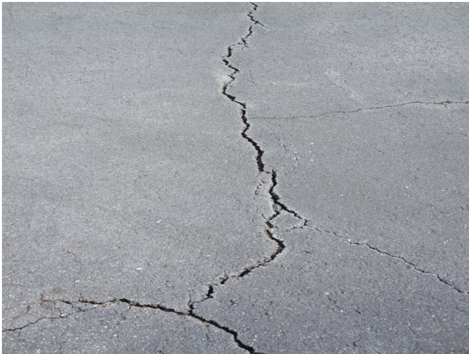
A01AT-30. Longitudinal and Transverse Cracking (Sample Unit #05).
