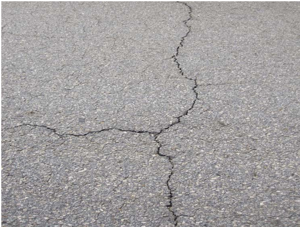
THANGAT-10. Longitudinal and Transverse Cracking (Sample Unit #02).
