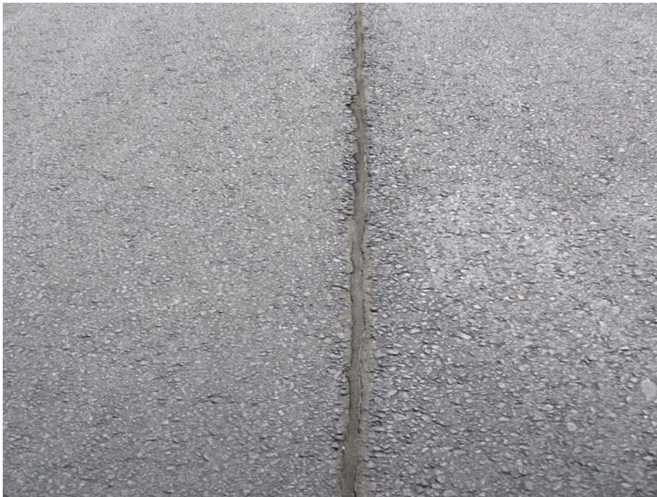
TAAT-40. Longitudinal and Transverse Cracking (Sample Unit #07).
