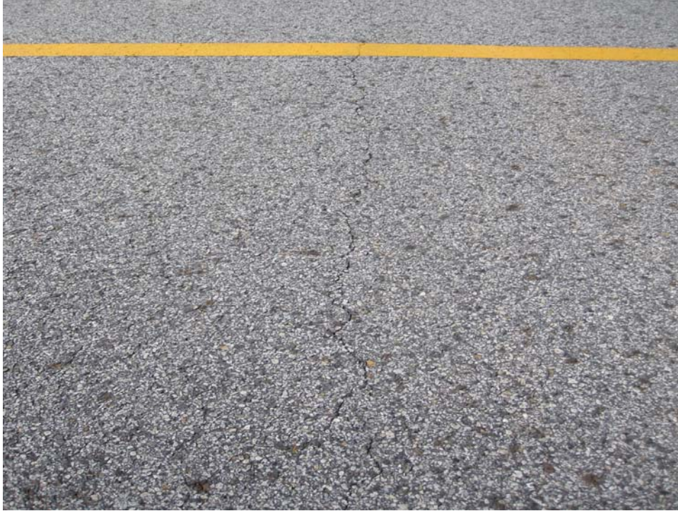
TAAT-50. Longitudinal and Transverse Cracking (Sample Unit #02).
