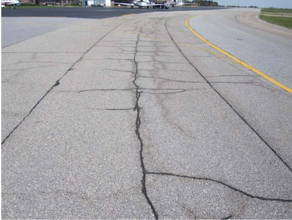
TAAT-30. Block Cracking (Sample Unit (09)).
