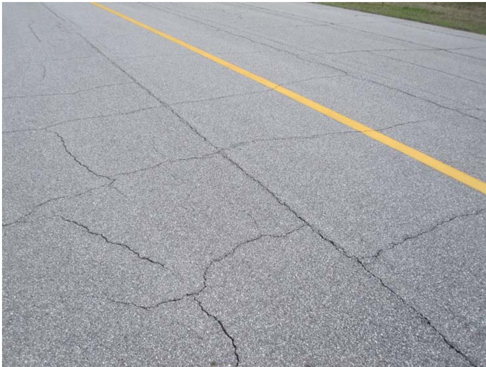
TAAT-30. Block Cracking (Sample Unit #13).
