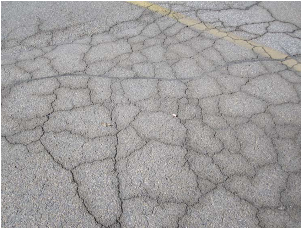
TBAT-10. Alligator Cracking (Sample Unit #08).
