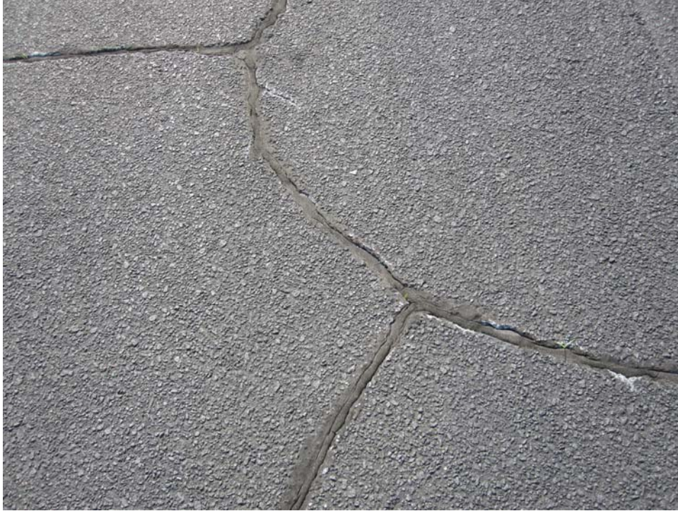
TBAT-15. Longitudinal and Transverse Cracking (Sample Unit #03).
