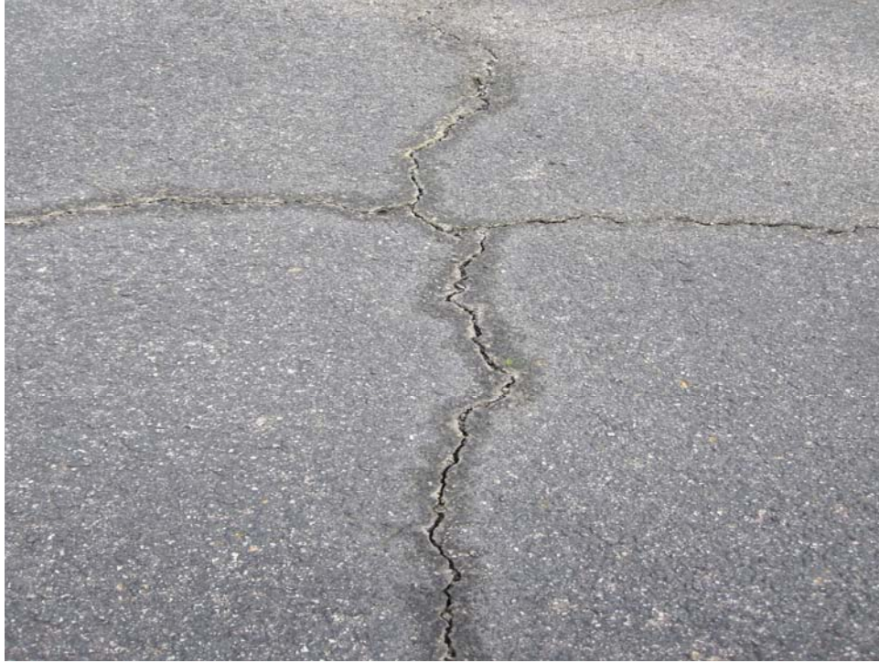
A01AT-10. Longitudinal and Transverse Cracking (Sample Unit #12).
