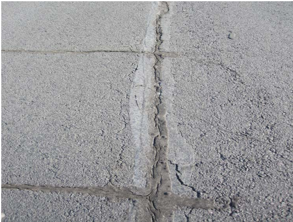
R220AT-30. Longitudinal and Transverse Cracking (Sample Unit #04).
