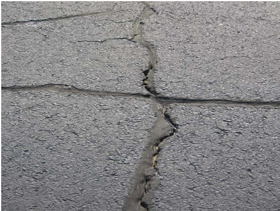
TBAT-20. Longitudinal and Transverse Cracking (Sample Unit #24).
