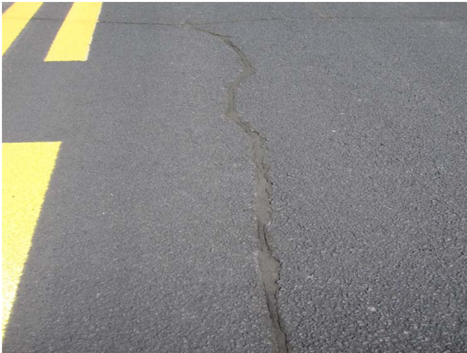
TAAT-30. Longitudinal and Transverse Cracking (Sample Unit #03).
