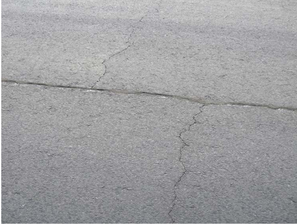
TAAT-10. Longitudinal and Transverse Cracking (Sample Unit #14).
