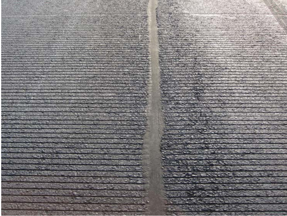
R927AT-20. Longitudinal and Transverse Cracking (Sample Unit #13).
