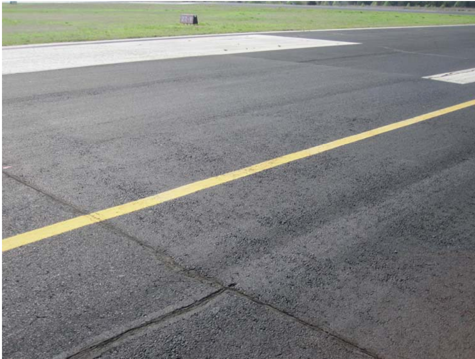
R220AT-10. Patching (Additional Sample Unit #23).
