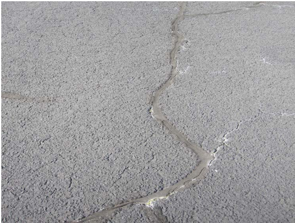
TBAT-30. Longitudinal and Transverse Cracking (Sample Unit #03).
