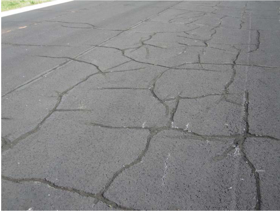
R220AT-30. Block Cracking (Sample Unit #32).
