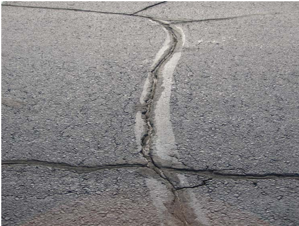
R220AT-10. Longitudinal and Transverse Cracking (Sample Unit #07).
