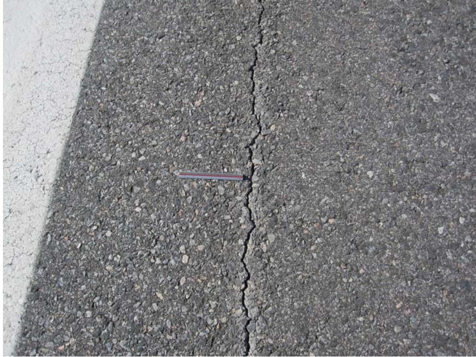
R523AD-10. Longitudinal and Transverse Cracking (Sample Unit #76).
