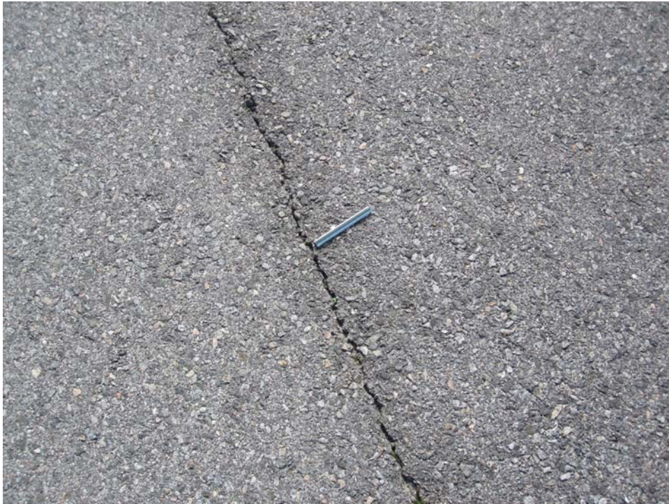
R1533AD-10. Longitudinal and Transverse Cracking (Sample Unit #03).
