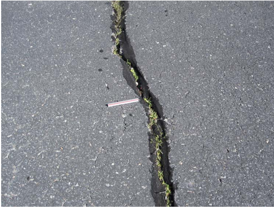
A01AD-10. Longitudinal and Transverse Cracking (Sample Unit #14).
