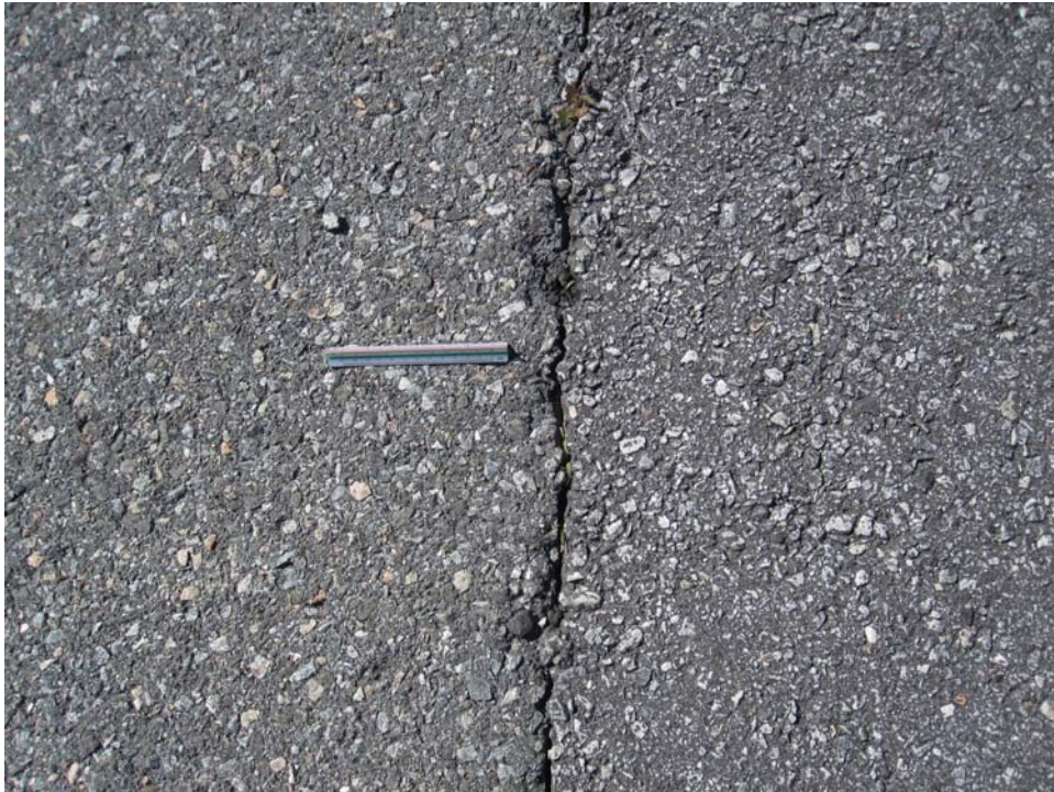
TAAD-10. Longitudinal and Transverse Cracking (Sample Unit #01).
