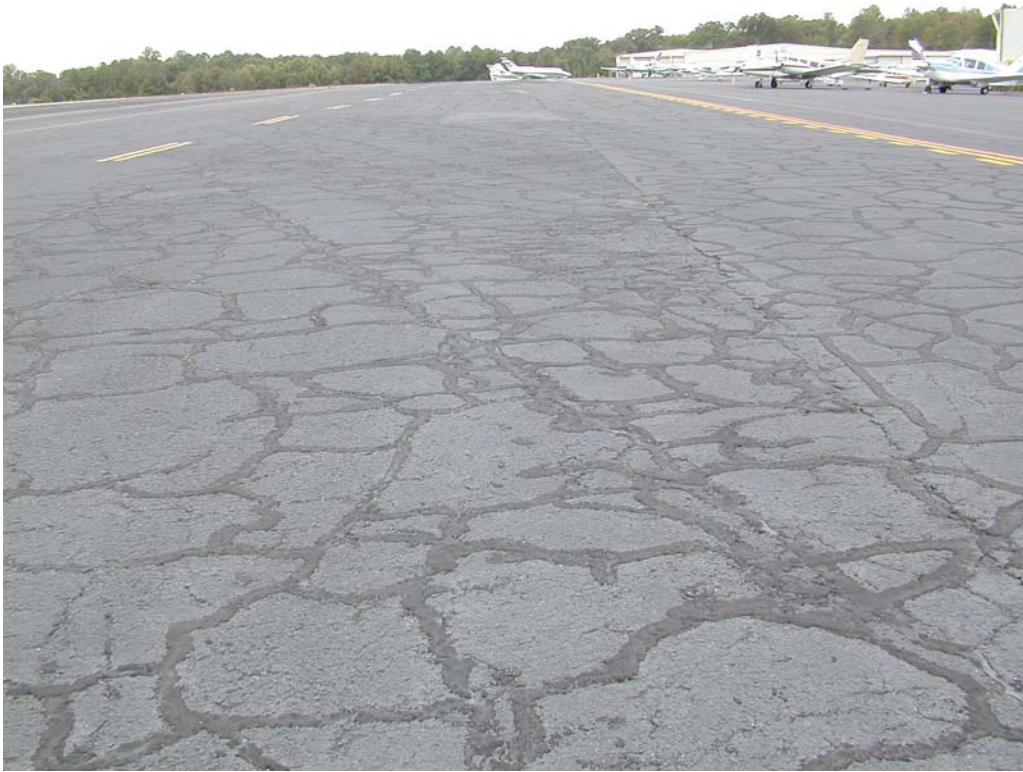
Block cracking in section APERIMAP-10.
