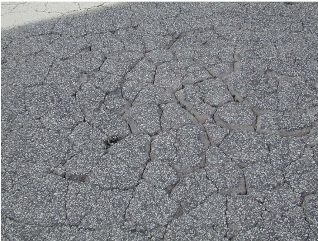
Alligator cracking in section R927AP-20.
