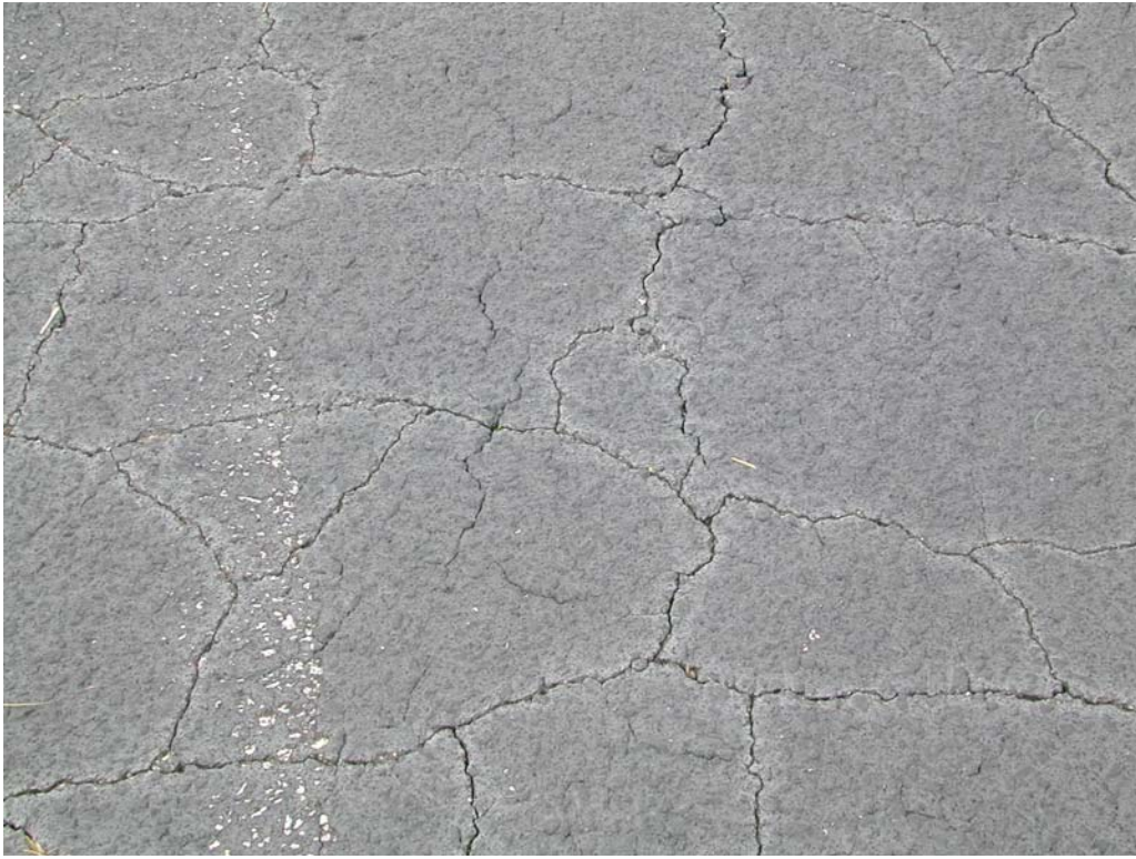
Alligator cracking in section TCAP-20.
