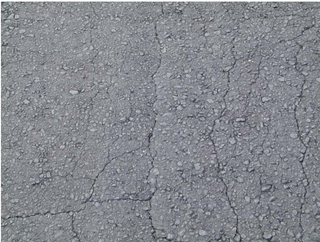
Alligator cracking in section TAAP-20.
