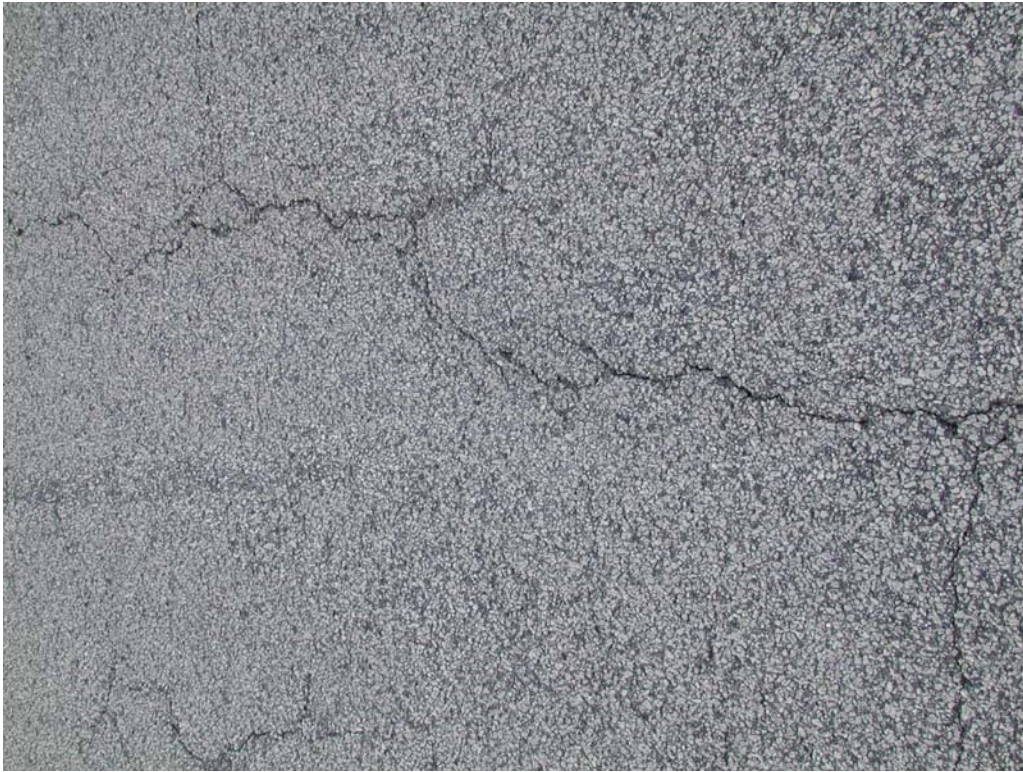
Alligator cracking in section THAP-10.
