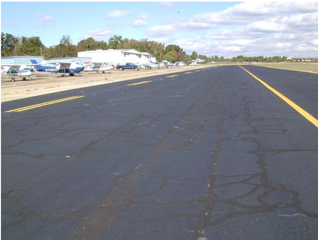
Block cracking in section TBAP-10.
