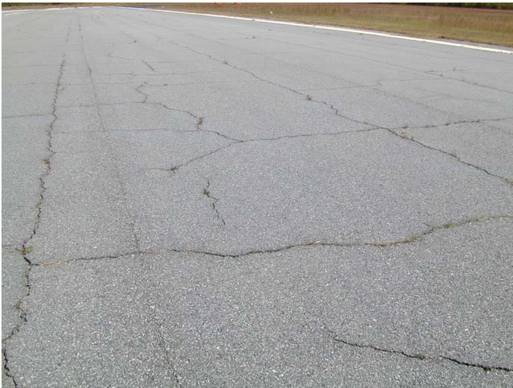
Block cracking in section R927AP-10.
