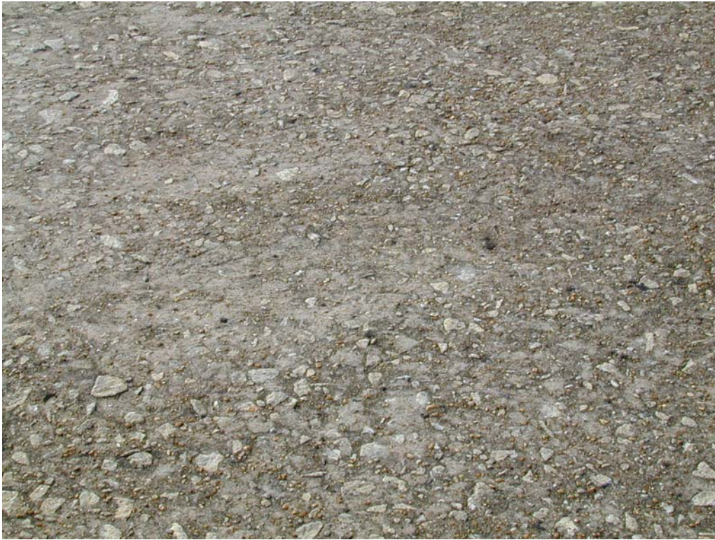
Scaling in section ANWRAMPAP-20.
