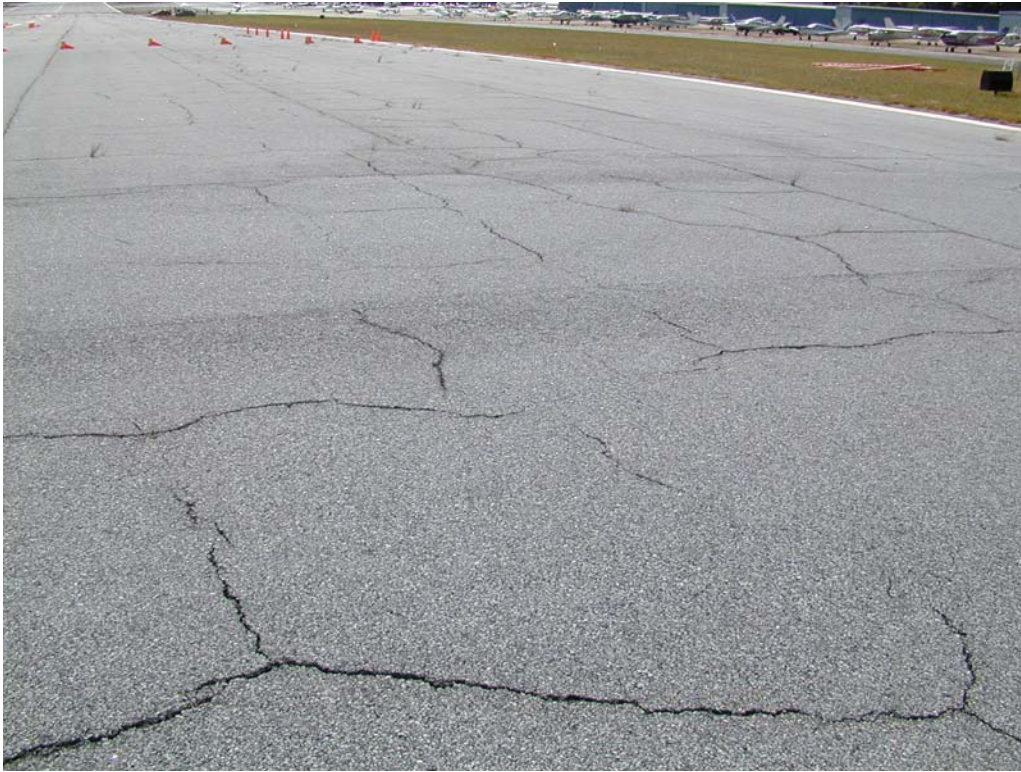
Block cracking in section R1634AP-10.
