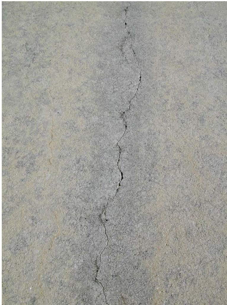
LTD cracking in section TAAP-10.
