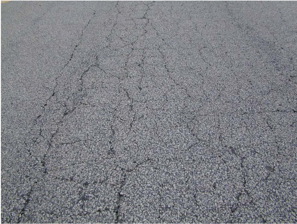
Alligator cracking in section TEAP-10.
