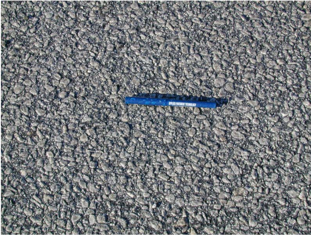
Raveling and weathering in section TKAP-20.
