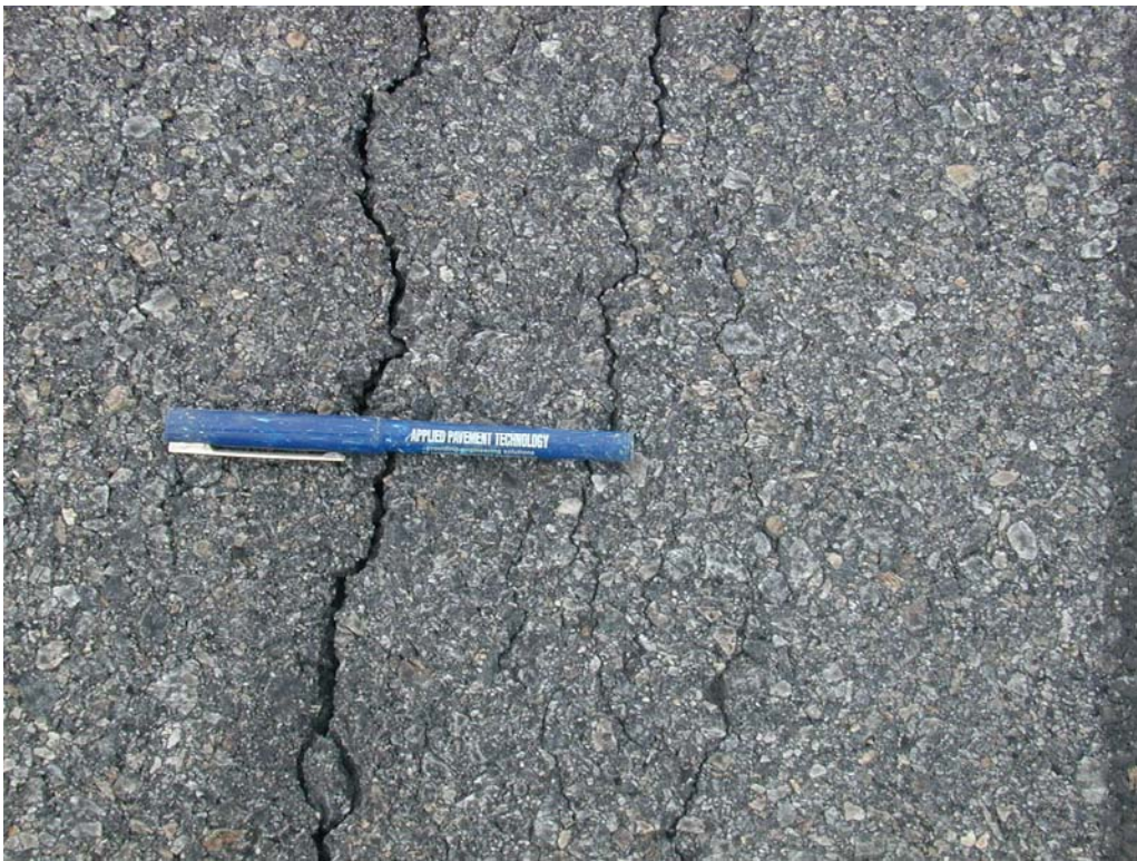
Alligator cracking in section R1331MGRA-10C.
