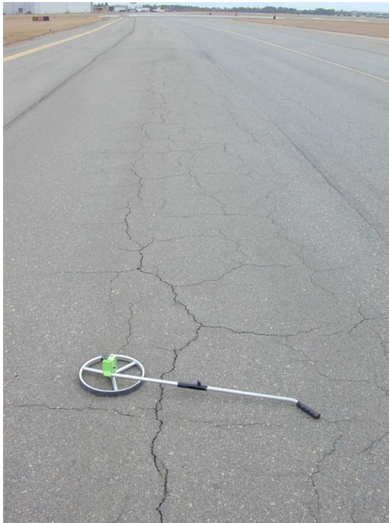
Block cracking in section TCMGRA-10.
