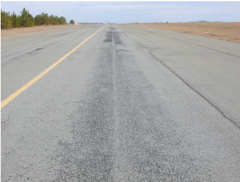
Bleeding in section TBMGRA-30.
