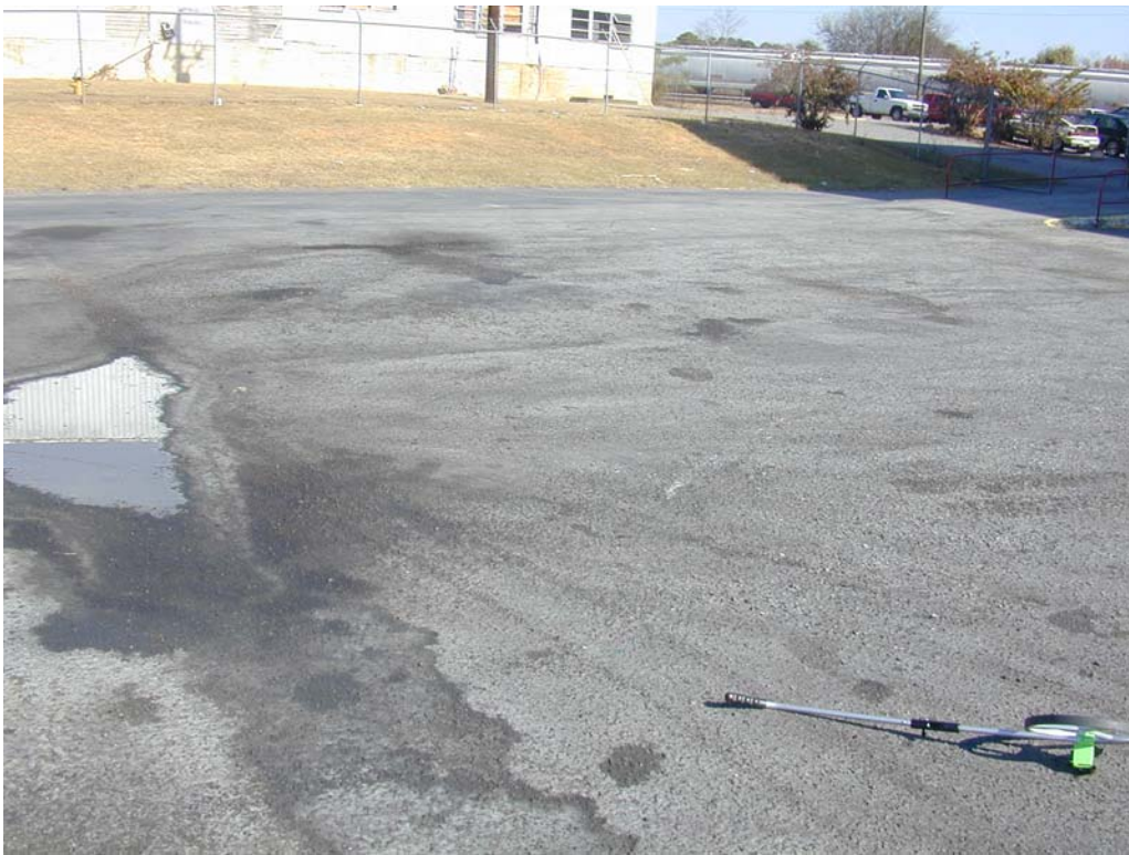
Raveling and weathering in section A01MGRA-80.
