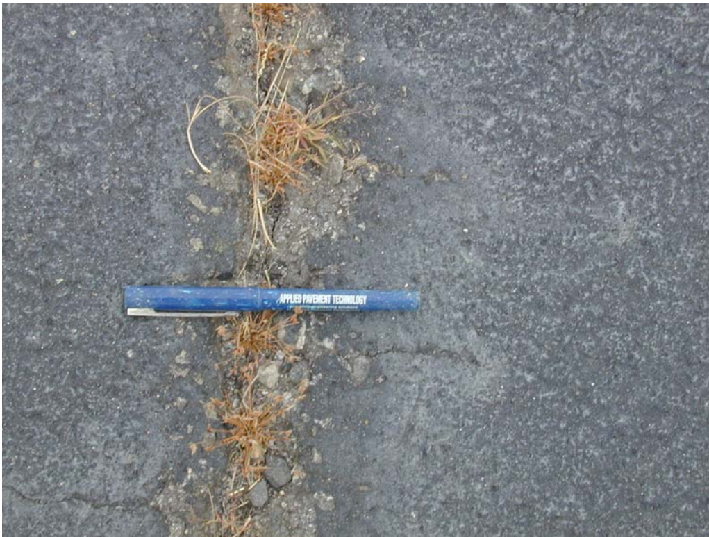
L&T cracking in section R1331MGRA-10N.
