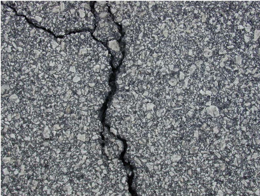
L&T cracking in section TBAB-10.
