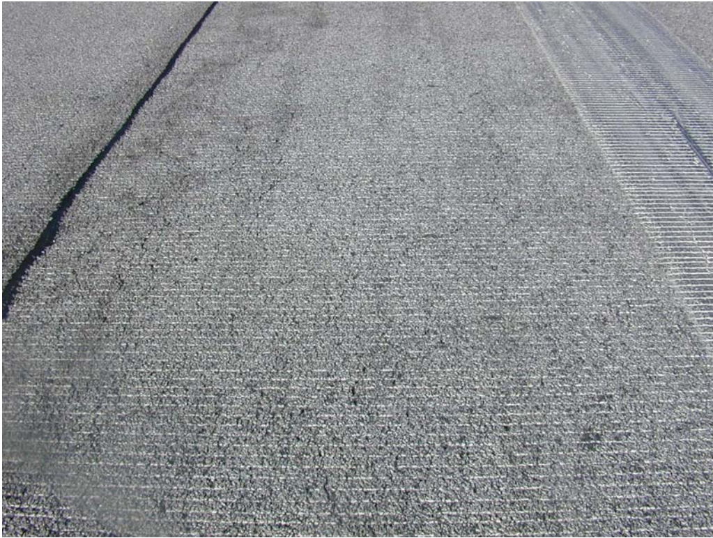
Alligator cracking in section R826AB-10.
