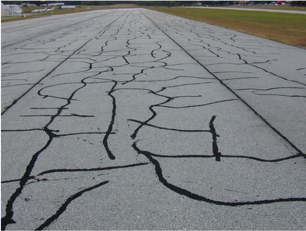
Block cracking in section TAAB-10.
