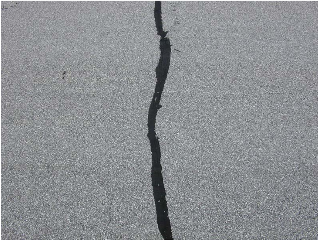
L&T cracking in section T927AB-10.
