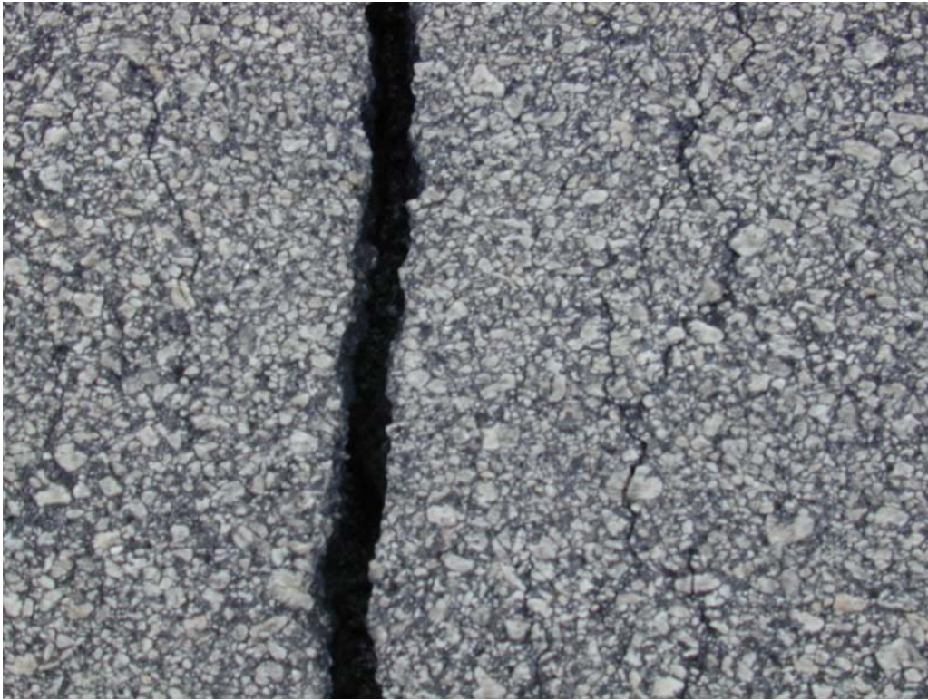
L&T cracking in section TIAB-10.
