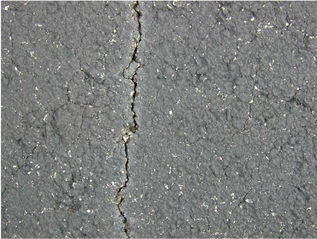
L&T cracking in section A01AB-10.
