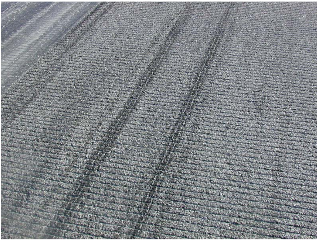
Weathering in section R826AB-10.
