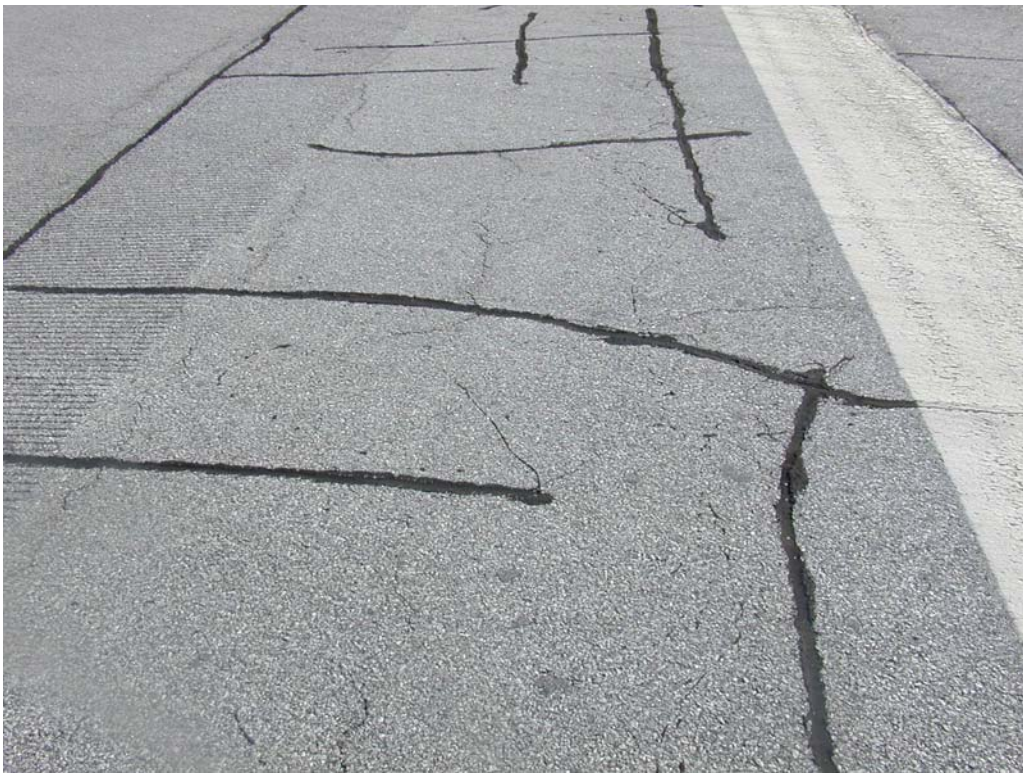
Block cracking in section R826AB-10.
