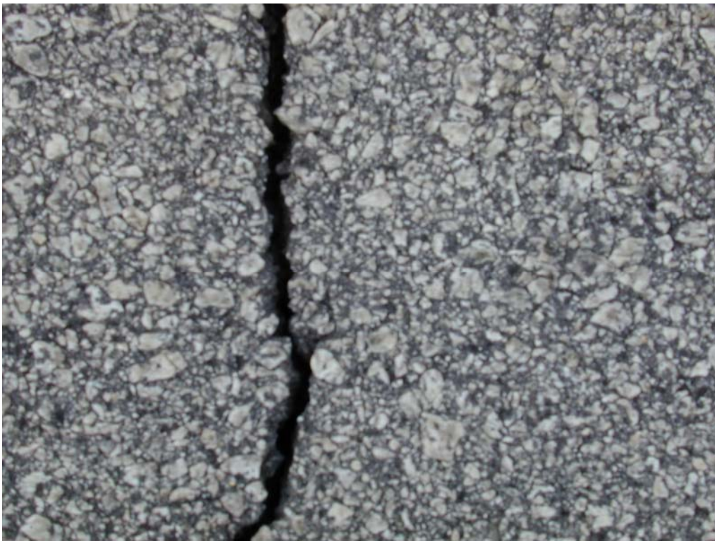
L&T cracking in section TAAB-10.
