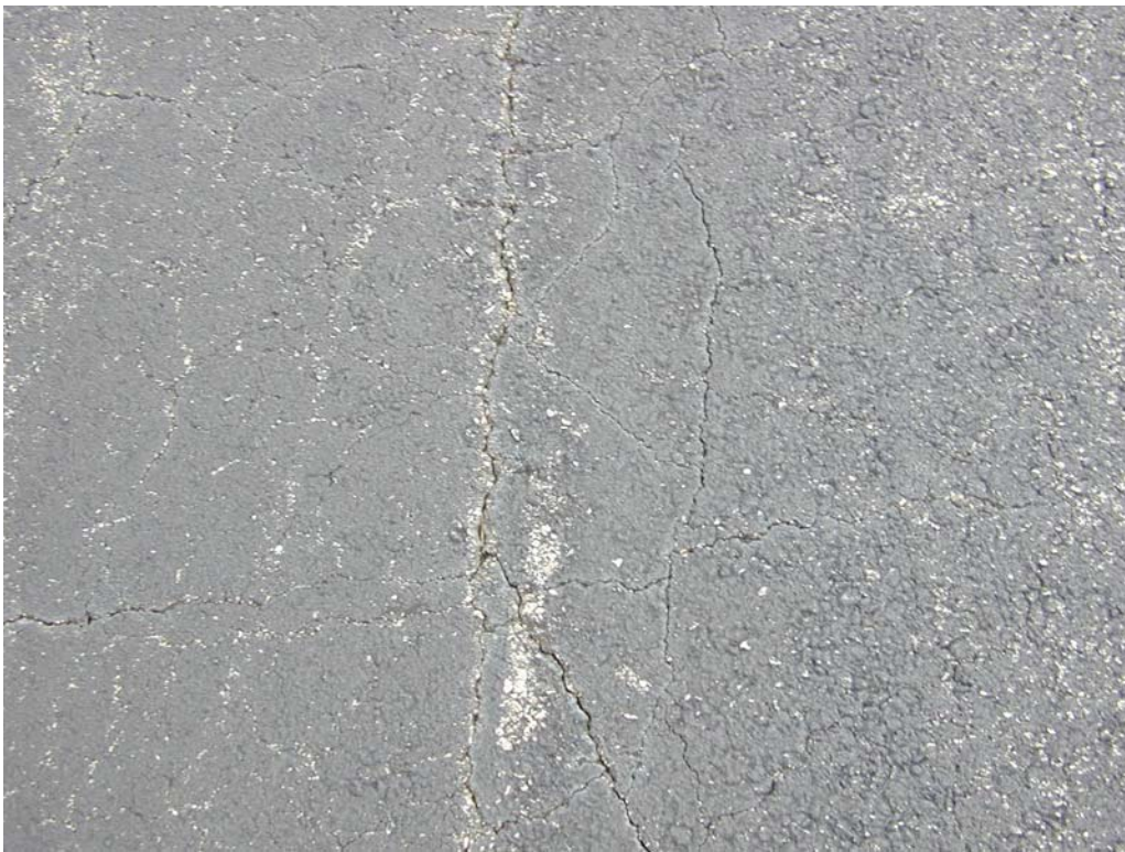
Alligator cracking in section A01AB-10.
