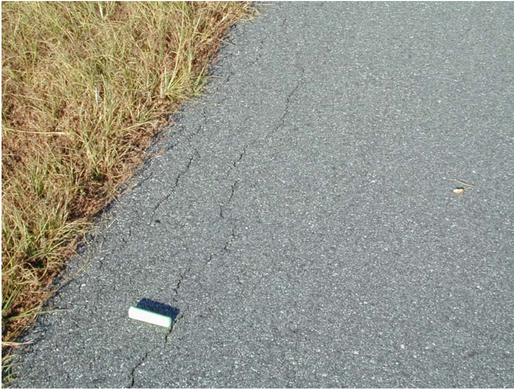
Edge cracking in section TFCL-40.
