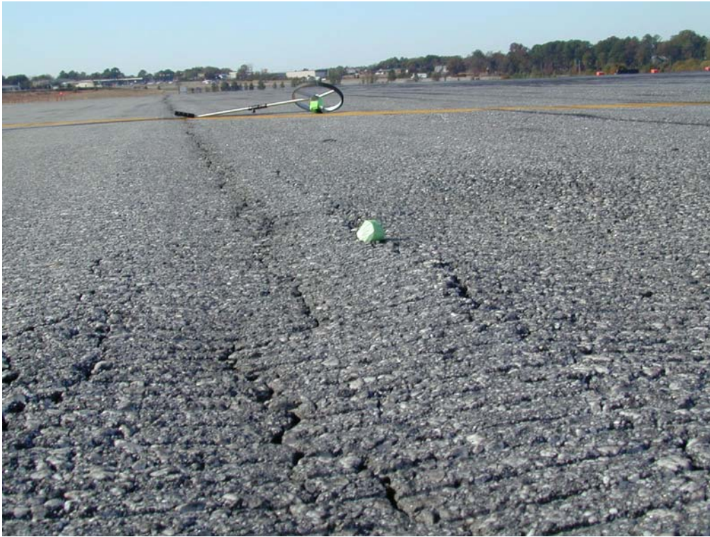
L&T cracking with swell in section R523CL-10.
