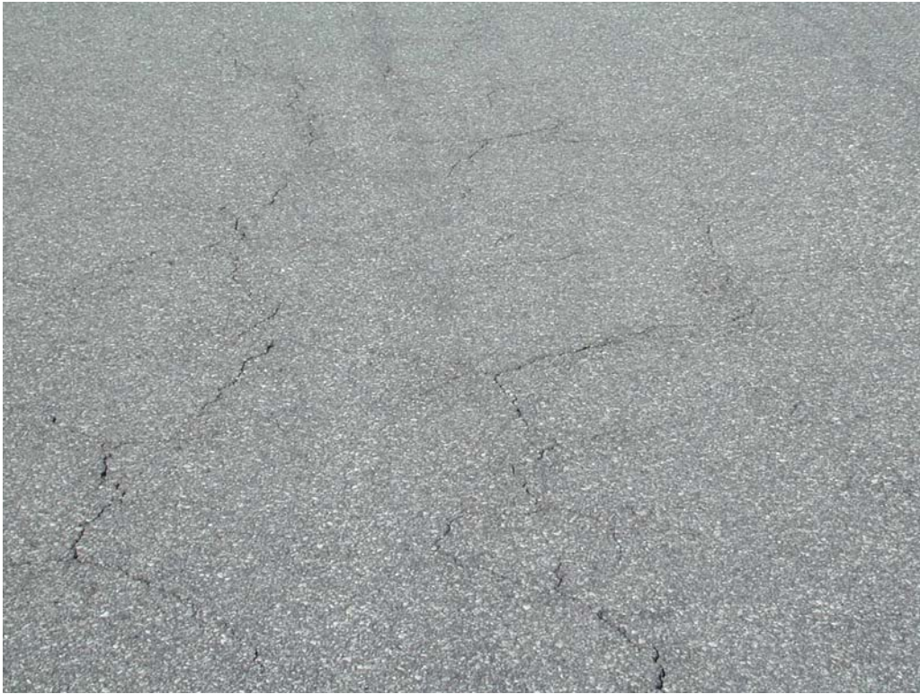
Block cracking in section TCCL-10.
