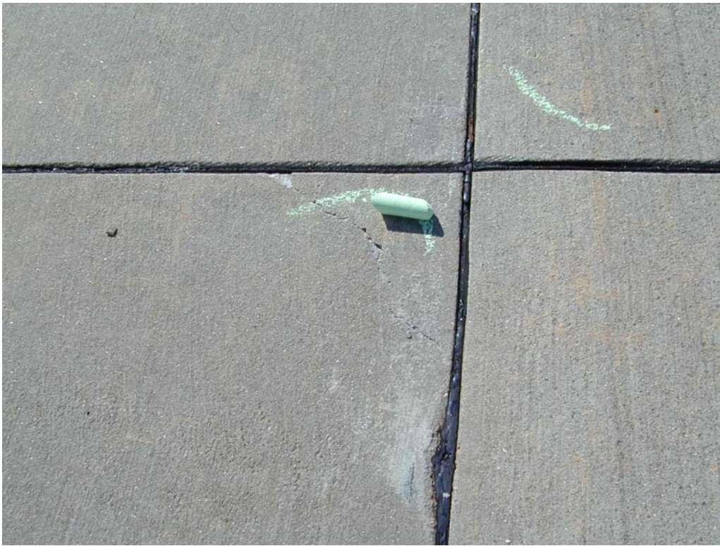
Corner spall in section ATERMCL-10.
