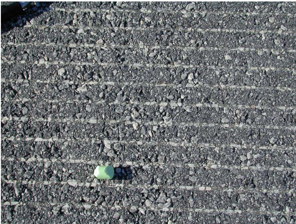
Weathering in section R523CL-10C.
