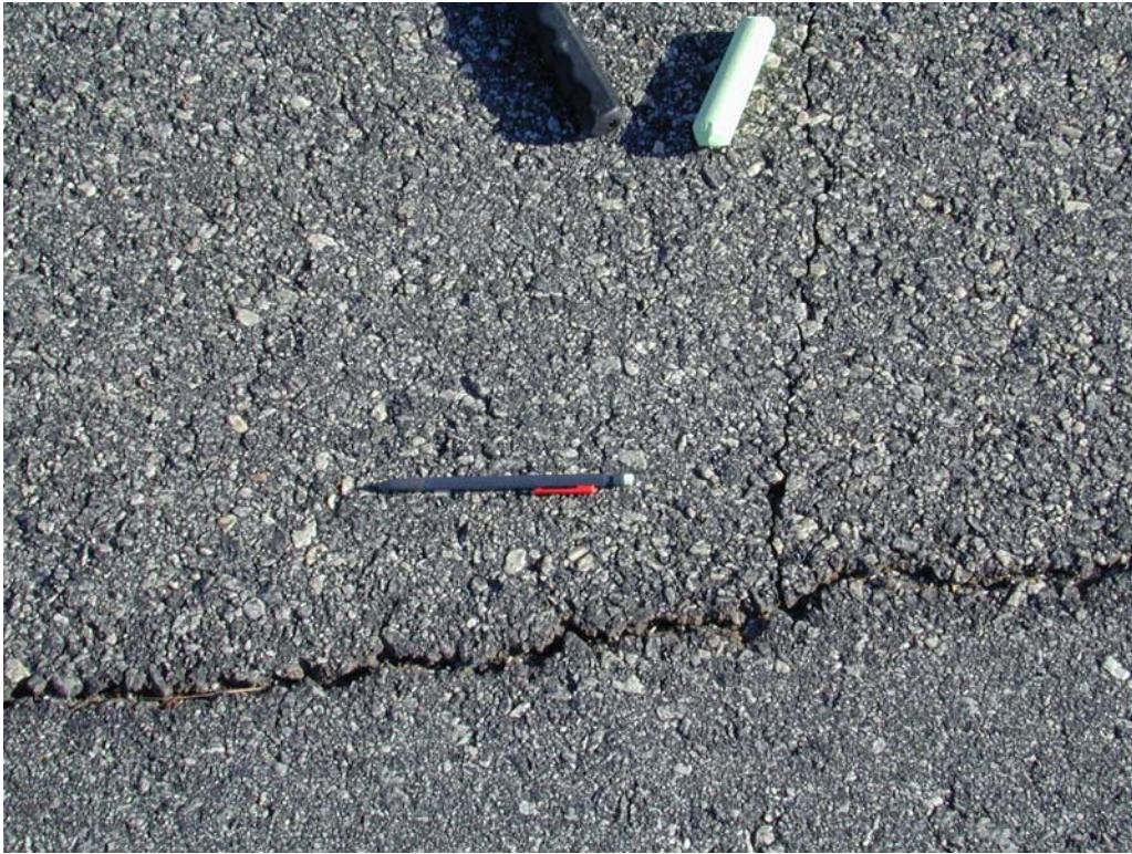
L&T cracking in section TFCL-10.
