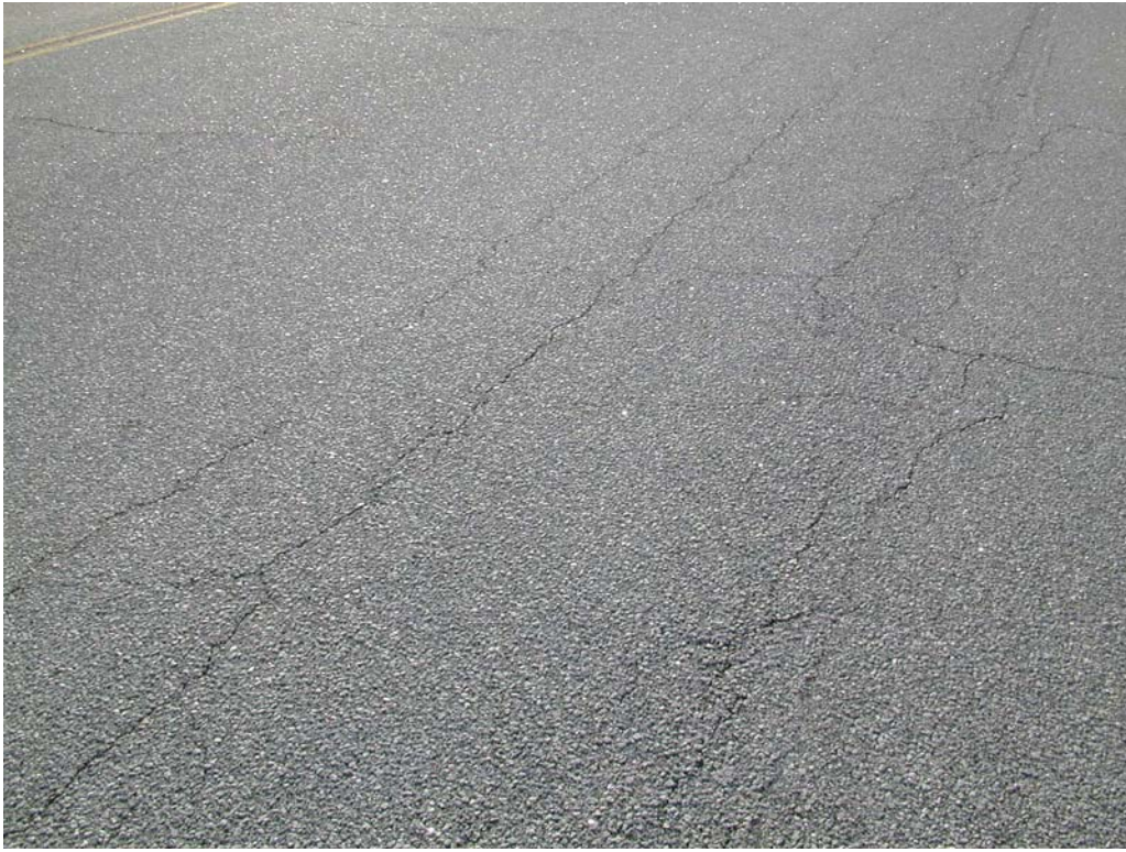
L&T cracking in section TEAGR-10.
