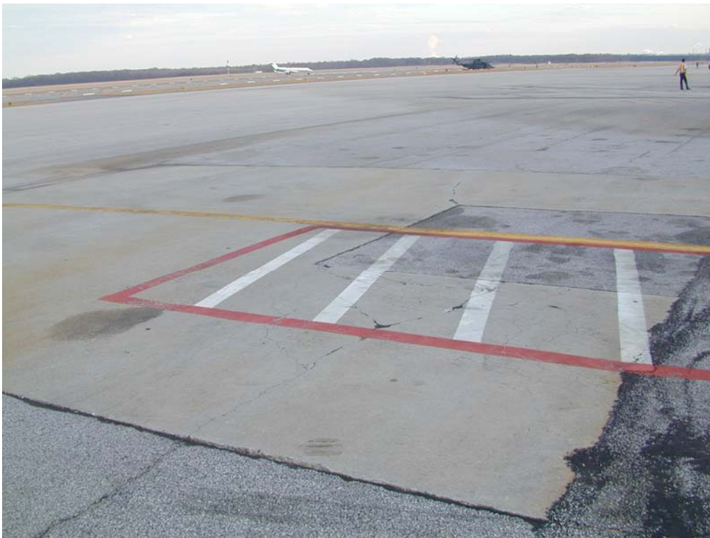
Overview of an additional sample unit with a PCC patch in section A01AGR-30.
