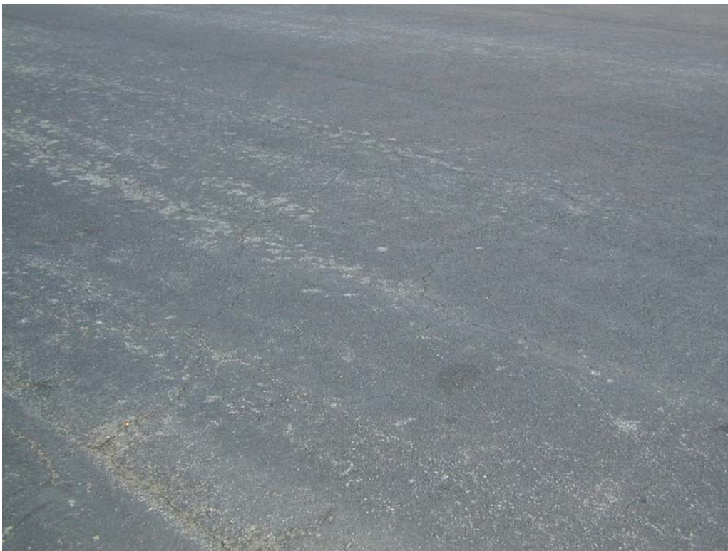
Block cracking in section AGARRETAGR-10.
