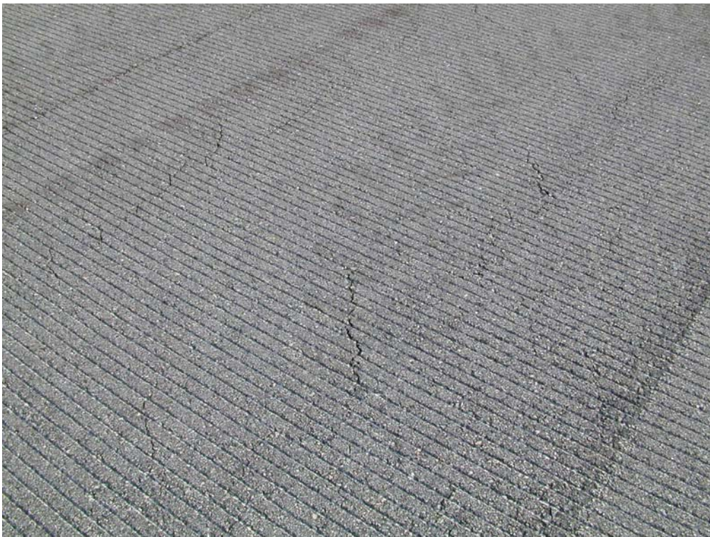
L&T cracking in section R1735AGR-10W.
