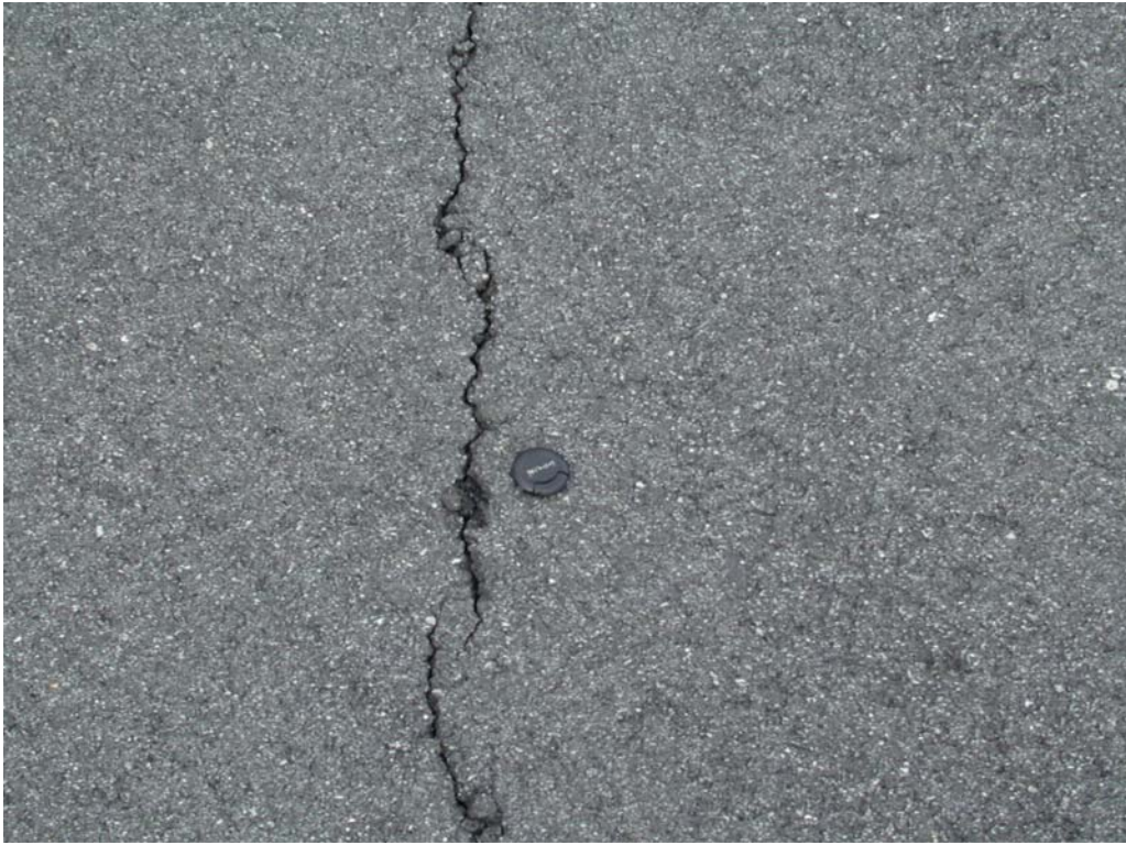
L&T cracking in section R1634AB-10.
