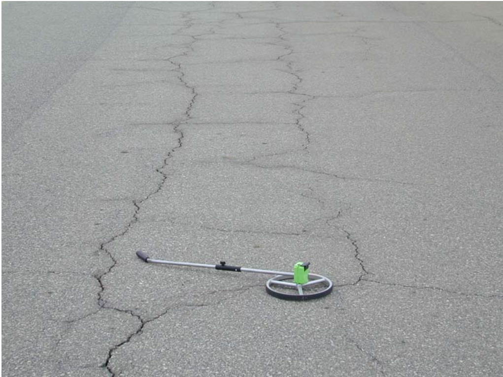
Block cracking in section TCAB-10.
