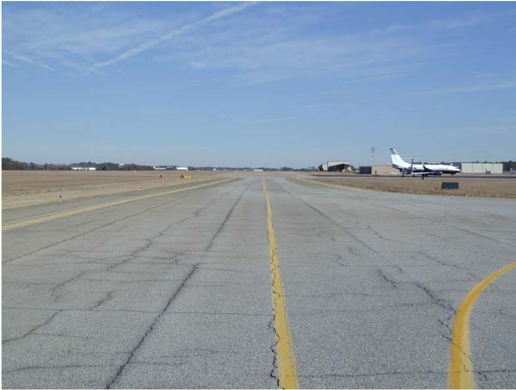
Block cracking in section TEAB-20.
