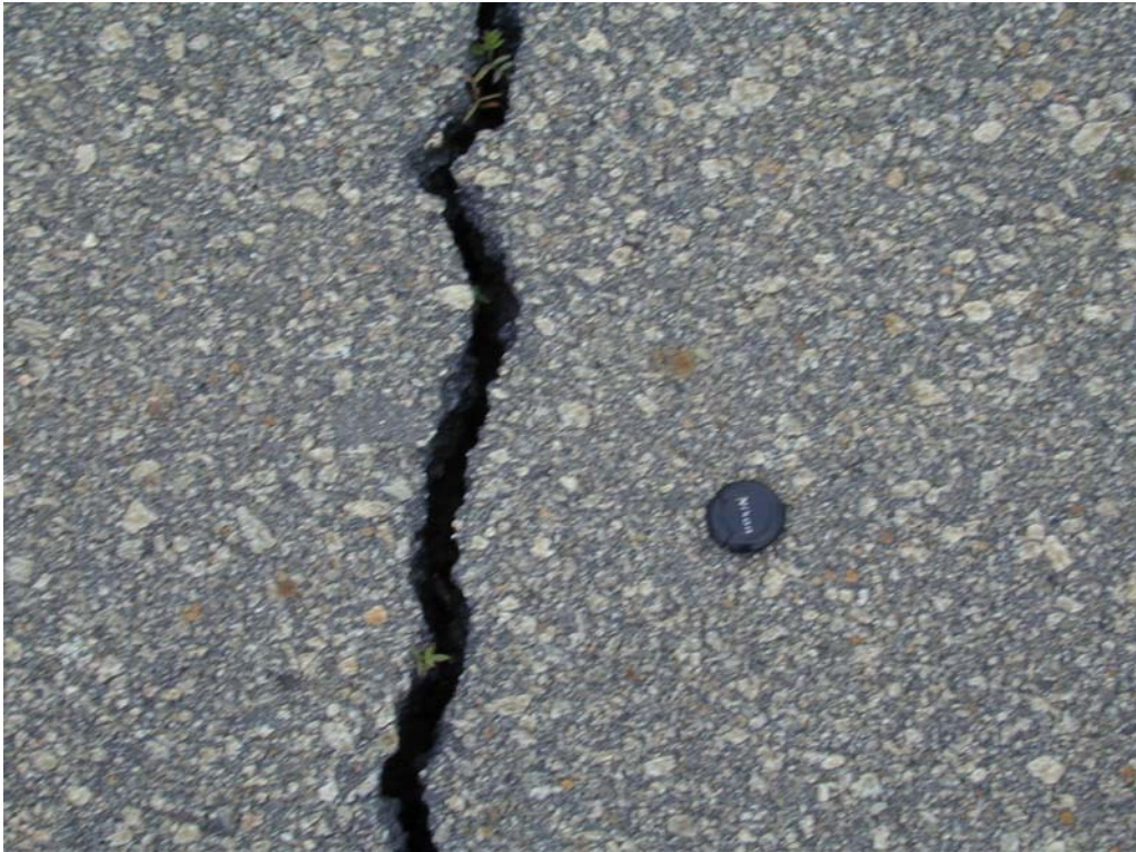
L&T cracking in section TCAB-20.
