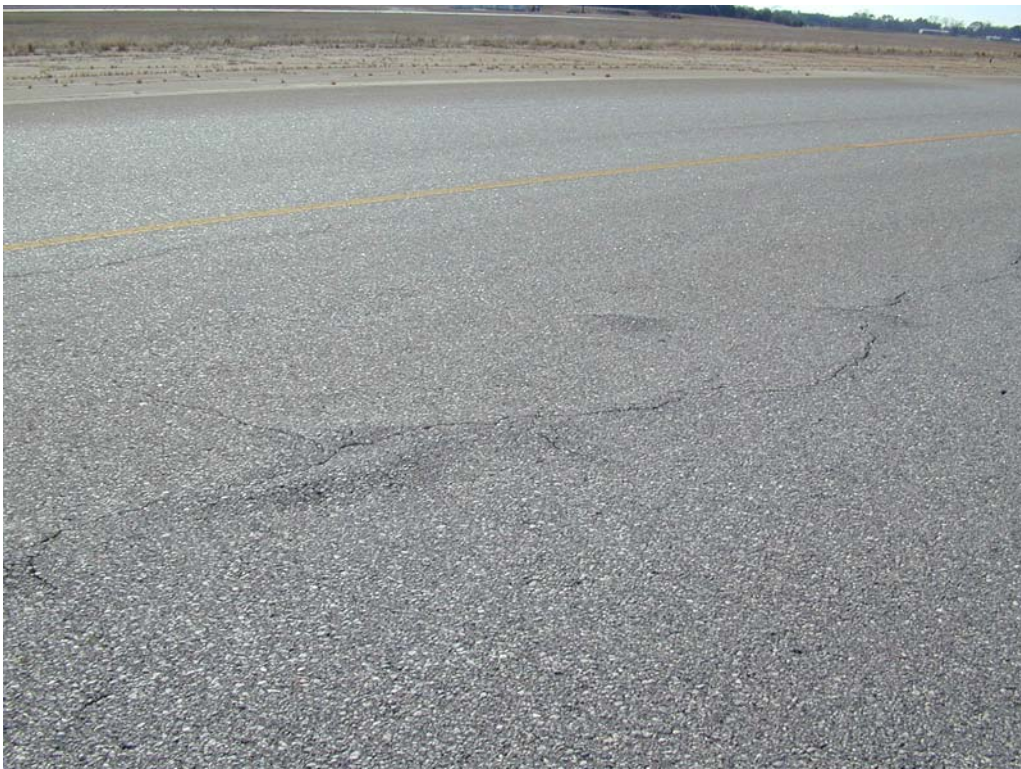
L&T cracking with swelling in section TEAB-20.
