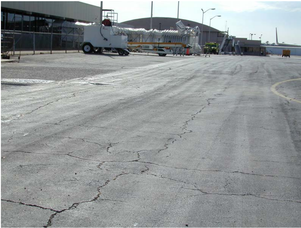
Block cracking in section ATERMAB-10.
