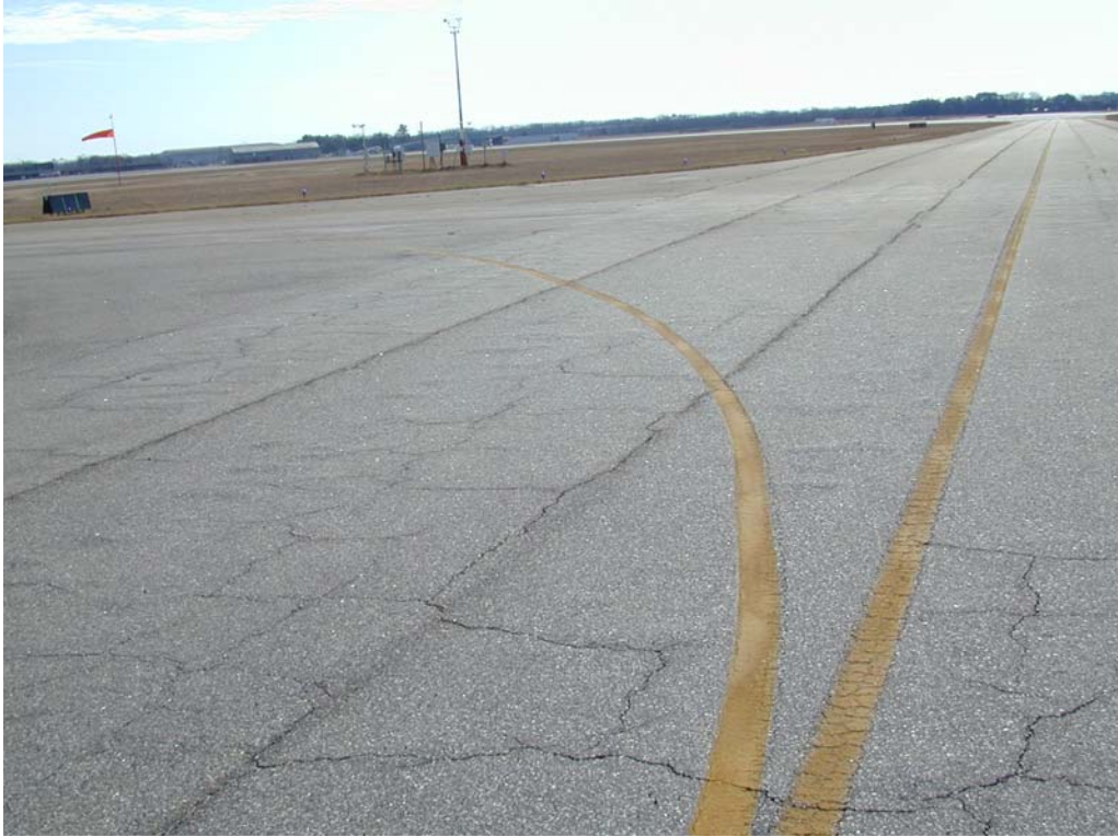
Block cracking in section TBAB-10.
