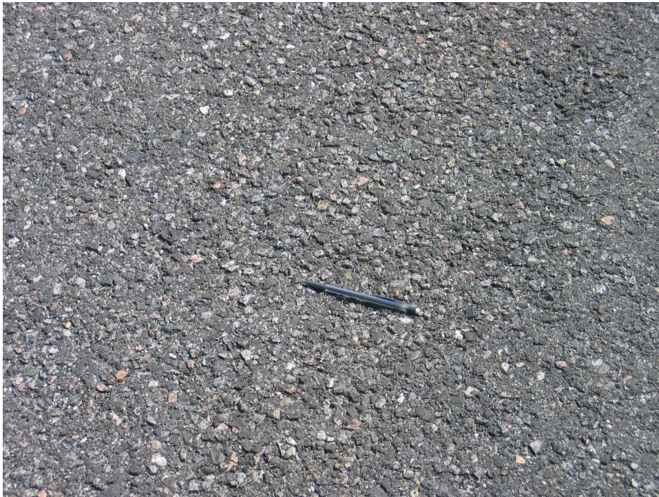
TAAD-10. Raveling and weathering.
