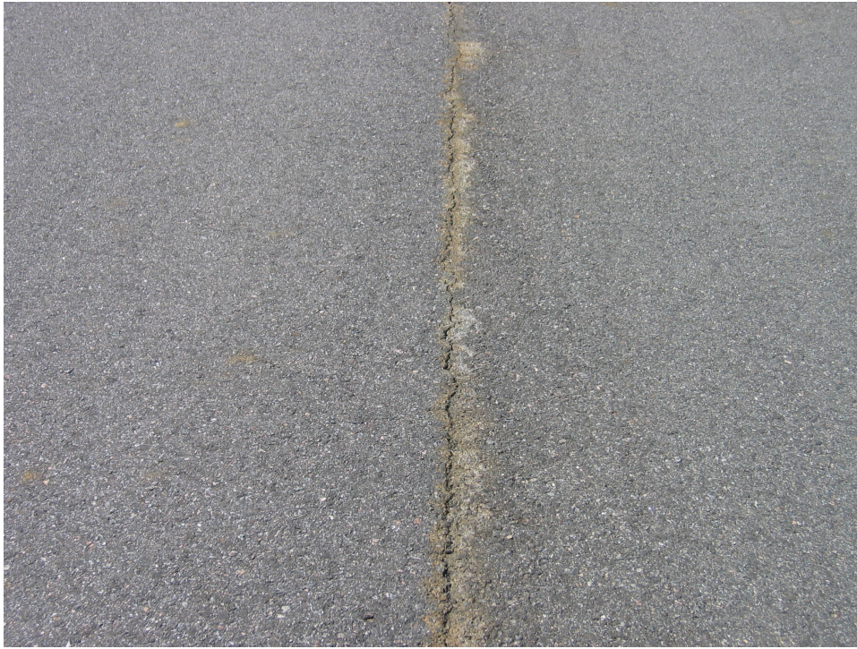
R523AD-10. L&T cracking.
