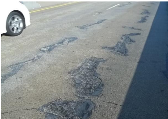
Damaged driving surface SR53west bridge
