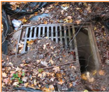
Figure 4.3-1 Missing Proper Cover
