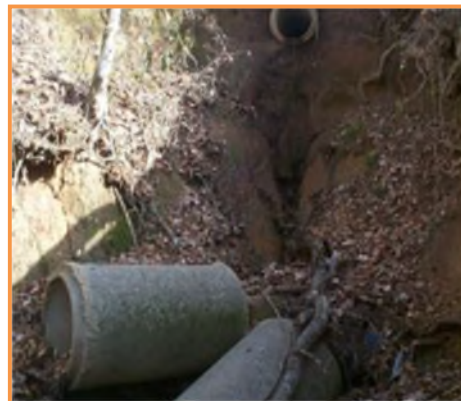
Figure 4.1-4 Severe Erosion and Collapse
