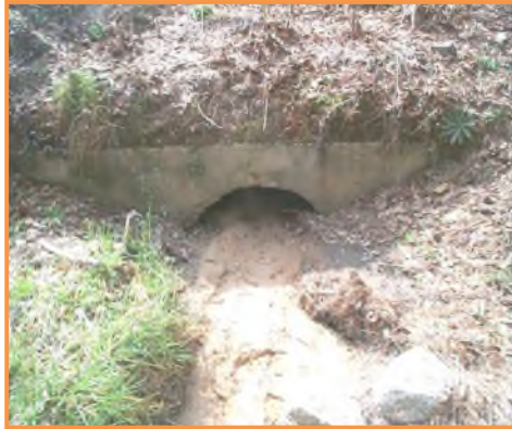
Figure 4.1-1 Pipe Conveyance Blocked with Sediment
