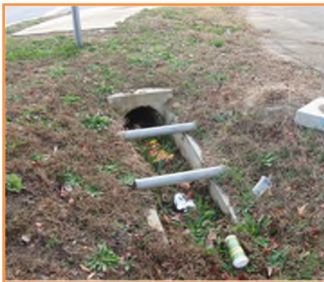
Figure 4.1-3 Pipe Conveyance with Trash
