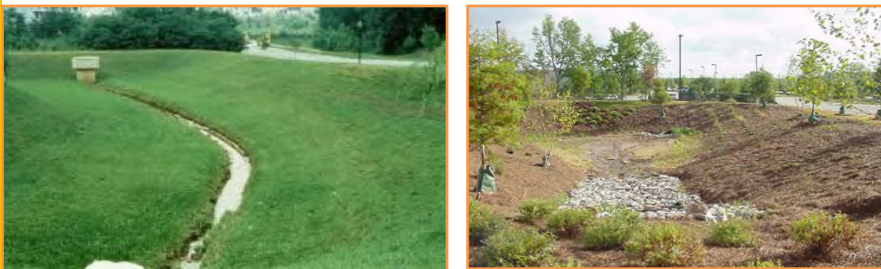
Figure 5.6-1 Dry Detention Basin with Low-Flow Channel (left) and Dry Detention Basin with Landscaping (right)
