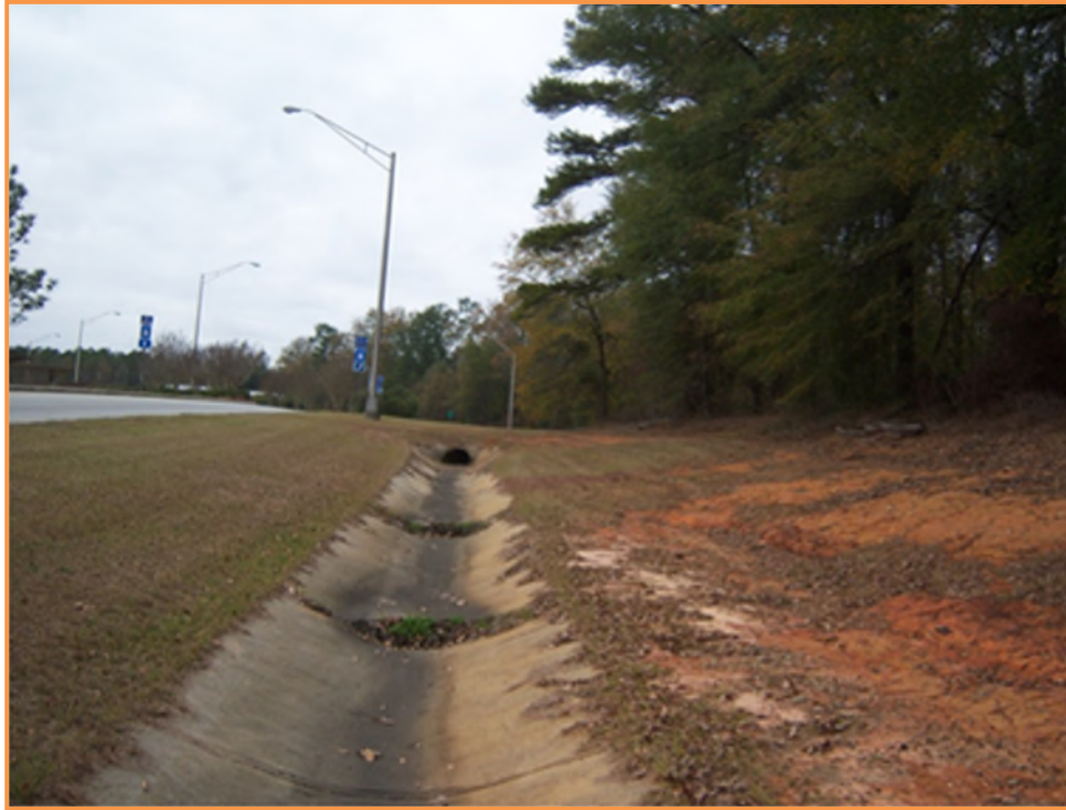
Figure 4.2-1 Cracks and Joint Separation in Concrete Channel
