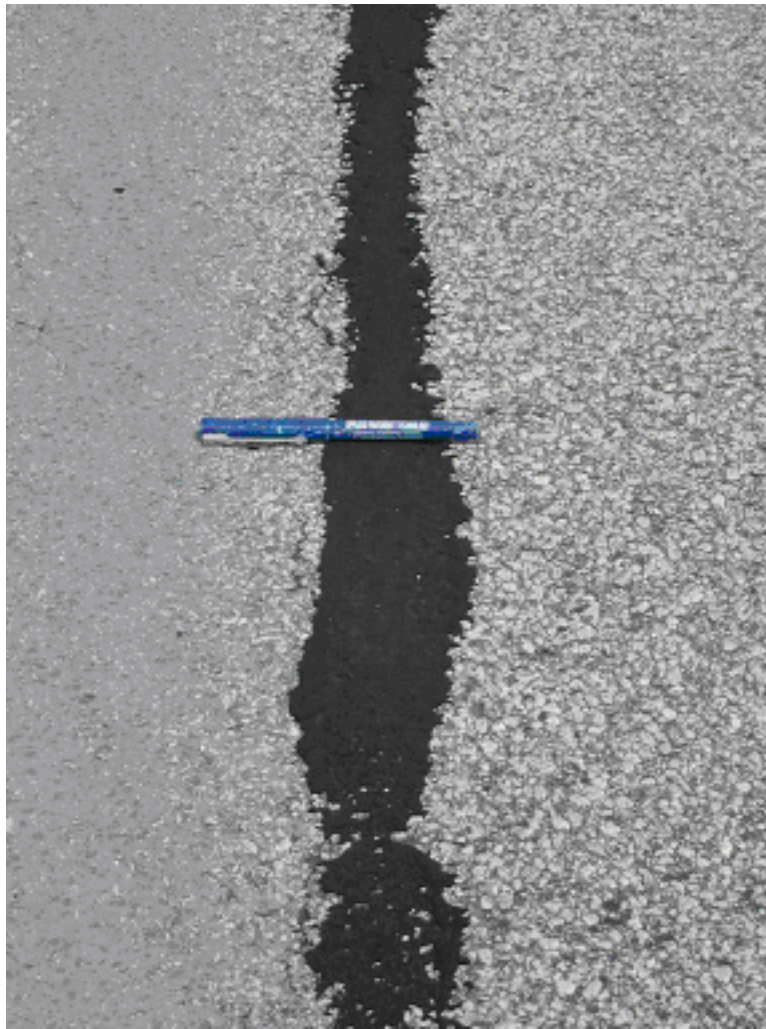
L&T cracking in section R523WI-10.
