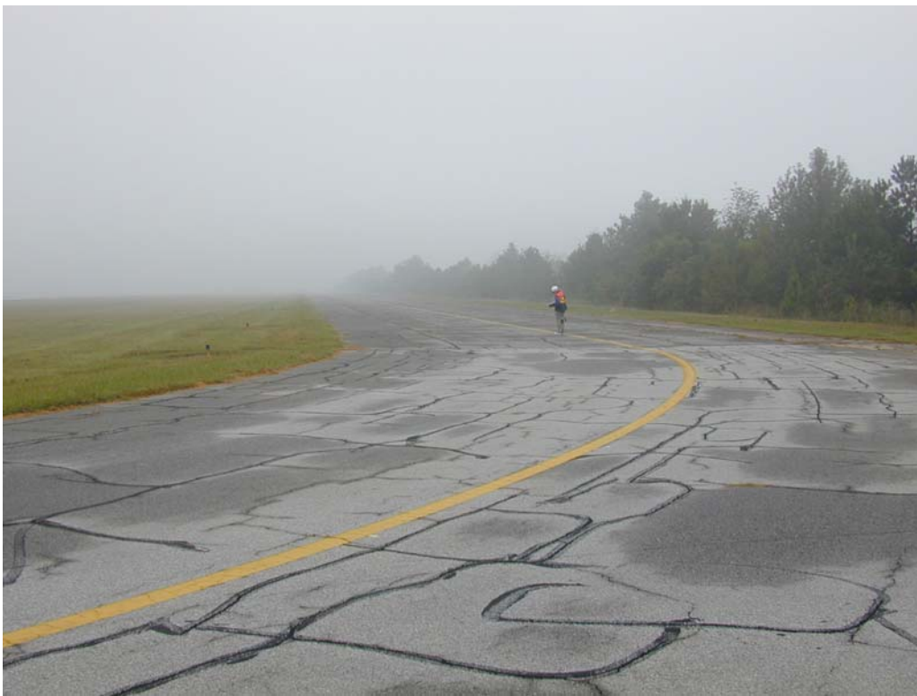
Overview of L&T cracking in section TBWI-10.
