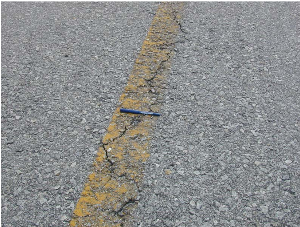
L&T cracking in section THANGWI-20.
