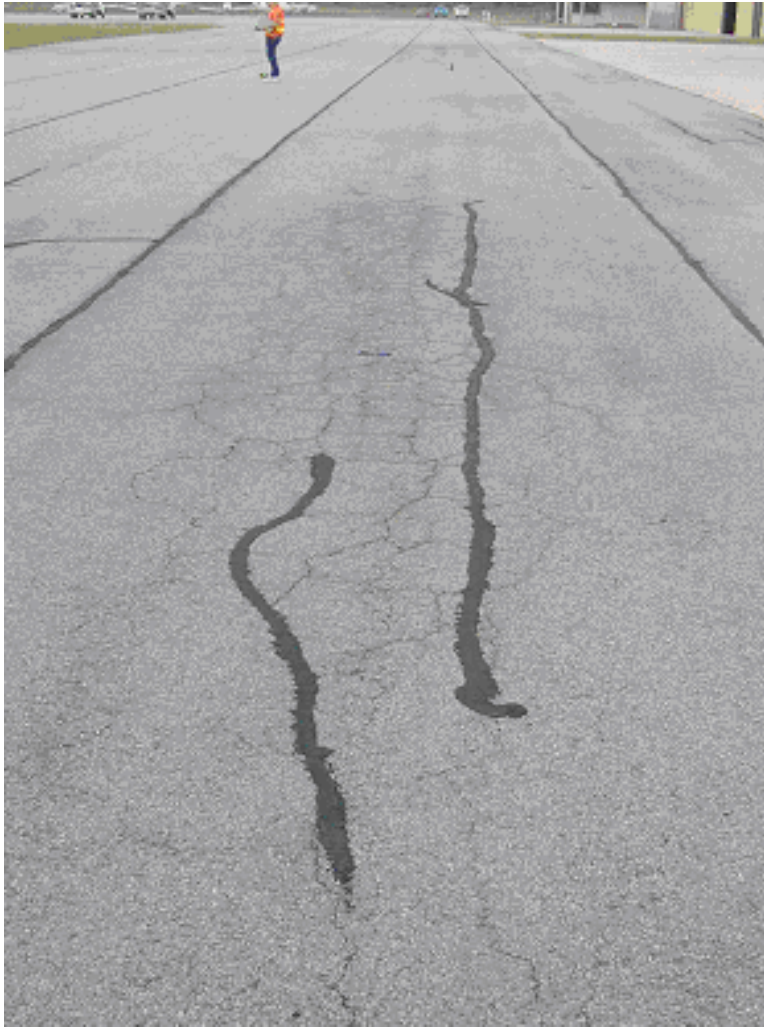
Alligator cracking in section A01WI-10.
