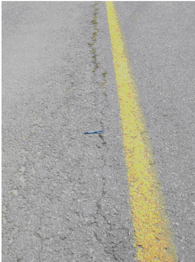
Raveling and weathering in section THANGWI-10.
