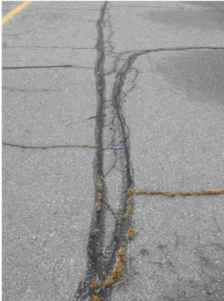
Alligator cracking in section TBWI-10.
