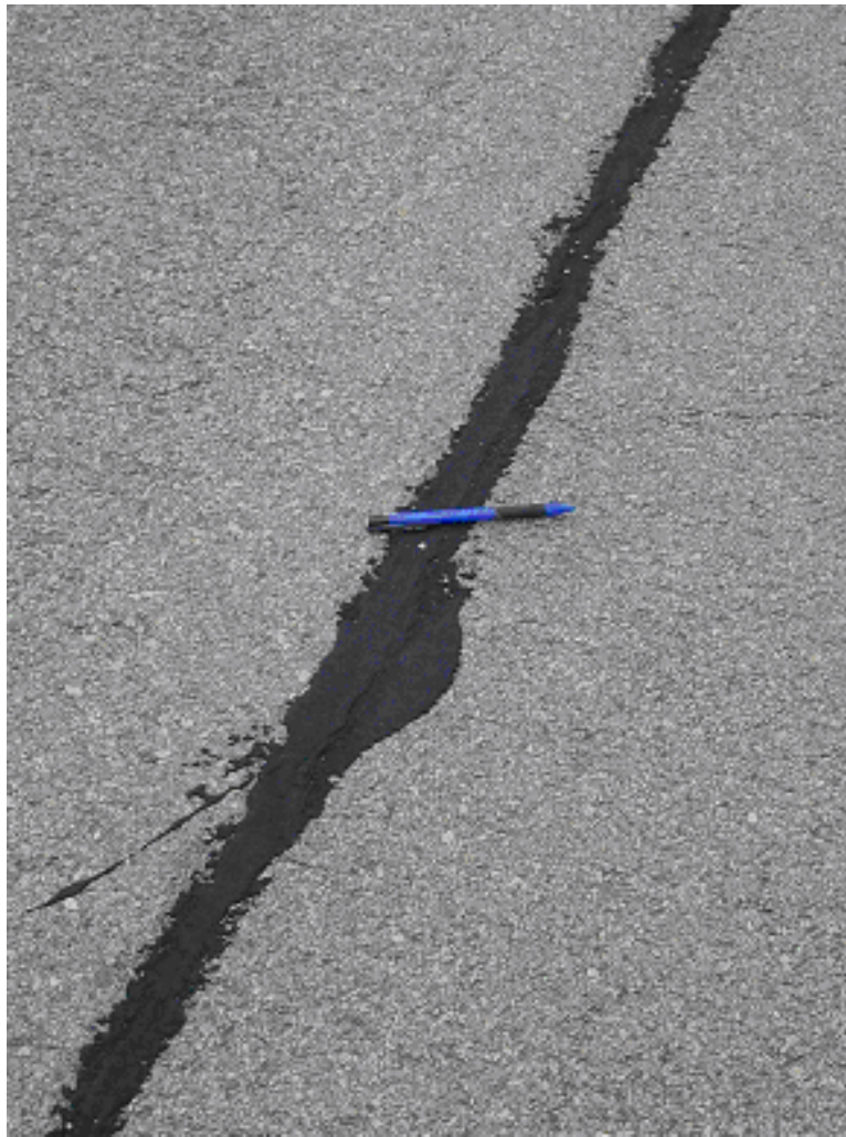
L&T cracking in section A01WI-10.
