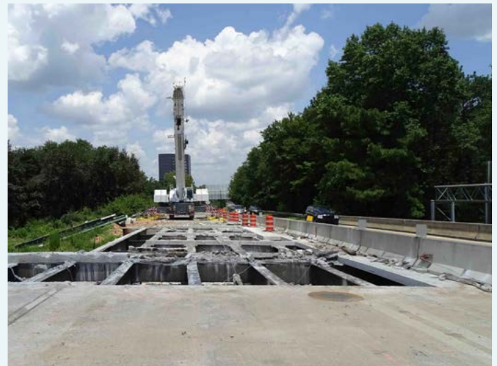
This bridge is located at the north end of the I-75/I-285 interchange next to the I-285 westbound collector-distributor (CD) lanes. Regular detours are scheduled in this area throughout the summer to accommodate the removal of the old bridge, making way for the installation of the new bridge.
