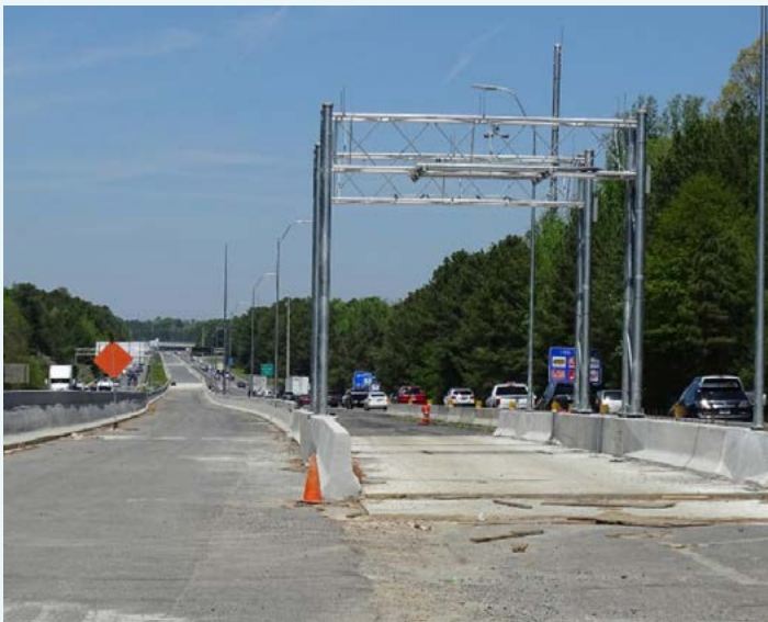
This I-575 slip ramp access point at Big Shanty Road will allow northbound motorists to “slip” out of the Express Lanes and back into the general purpose lanes.
