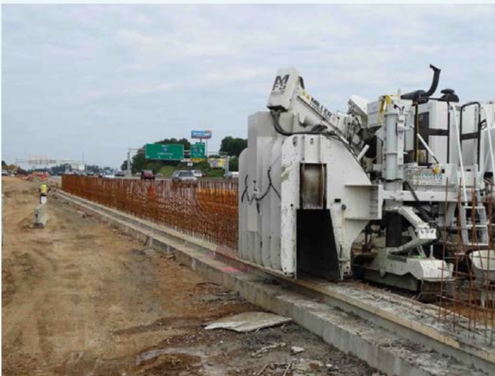
This machine, called a "slip form," installs or "slips" into place permanent concrete barrier walls near I-75 and Bells Ferry Road. These walls will serve to divide Express Lane traffic from the existing general purpose lanes.
